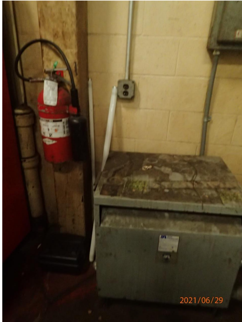
Photo 1: Two spent fluorescent lamps were observed without being in a closed, labeled, and dated container.
