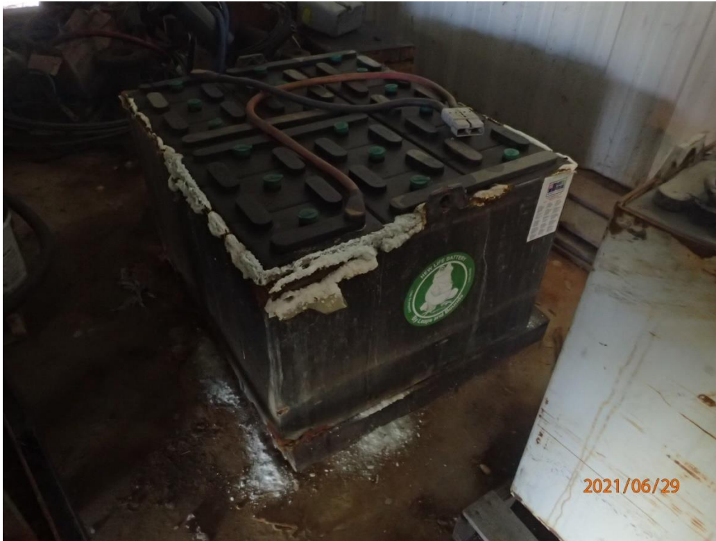
Photo 8: Leaking forklift battery, not labeled or properly closed in a container.
