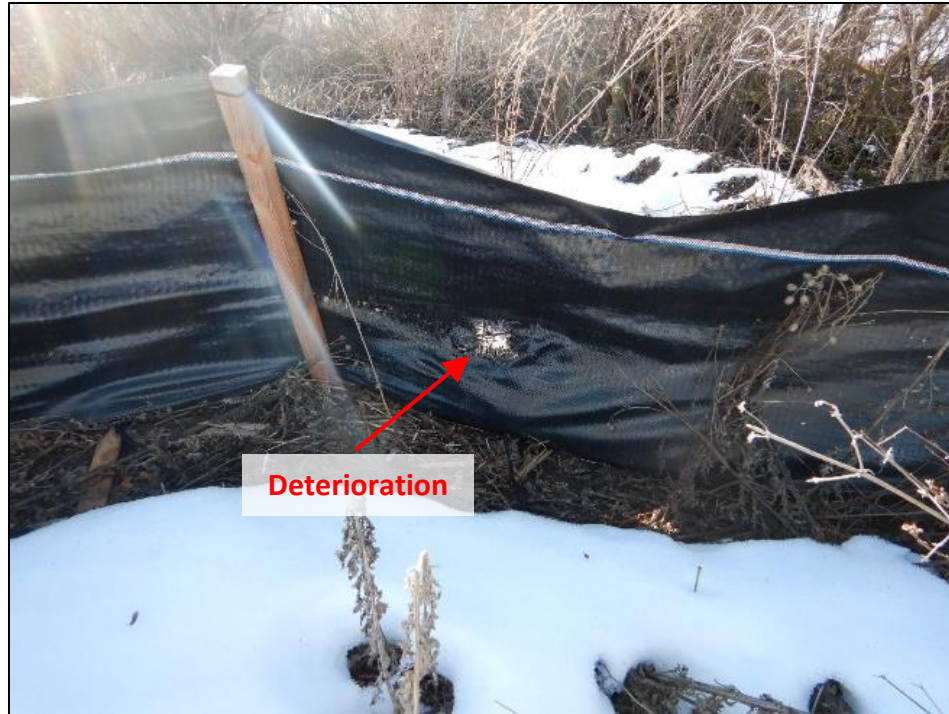
Photograph 9. View, facing south, of a section of the silt fence along the Site's southern perimeter. Note the deterioration. The silt fence is located east of Photograph 8 .
