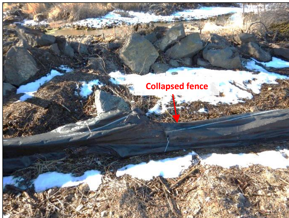
Photograph 8. View, facing south, of a collapsed silt fence along the Site's southern perimeter. The silt fence is located east of Photograph 7 .
