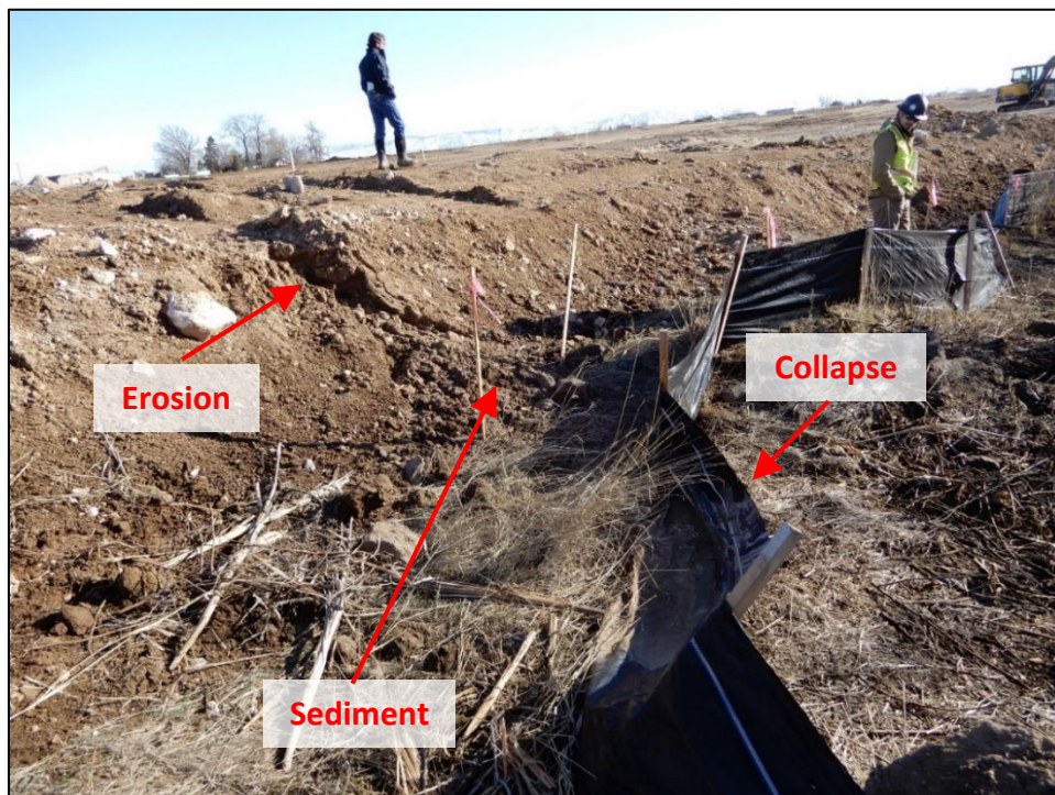
Photograph 10. View, facing east, of a collapsed silt fence along the Site's south-central perimeter. Note the erosion and sediment adjacent to the silt fence.
