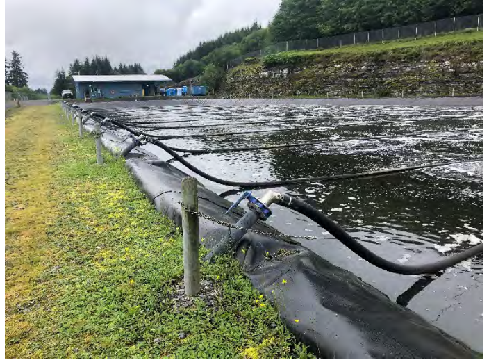
Photo #:10 (IMG_2389) Description: Photo of the aeration basin and diffusers.
