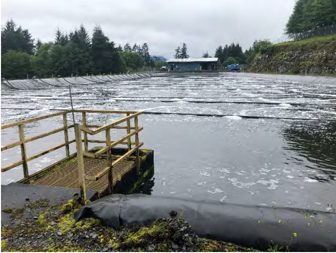
Photo #:09 (IMG_02388) Description: Photo of the outlet of the aeration basin
