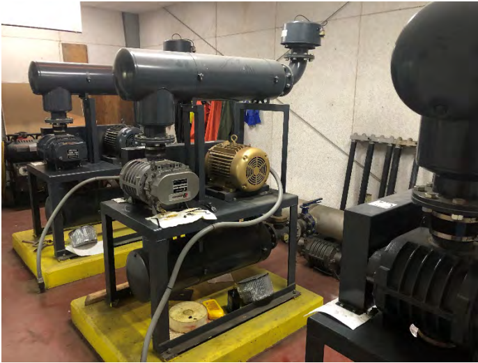
Photo #:11 (IMG_2390) Description: Photo of the 3 blowers that power the aeration basin.
