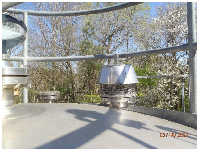
Figure 26: P3140038.JPG: Equipment on the top of the Used Acetone Tank
