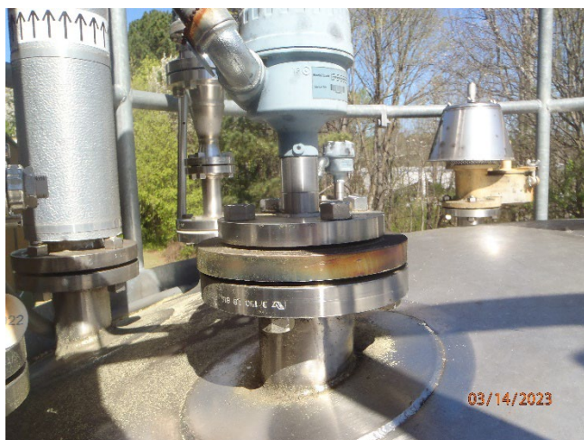
Figure 21: P3140033.JPG: Equipment on the top of the Used Acetone Tank
