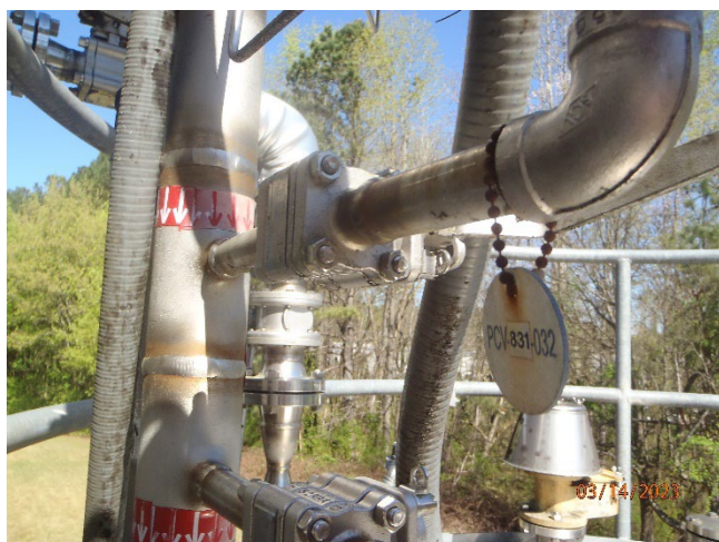
Figure 29: P3140041.JPG: Equipment on the top of the Used Acetone Tank
