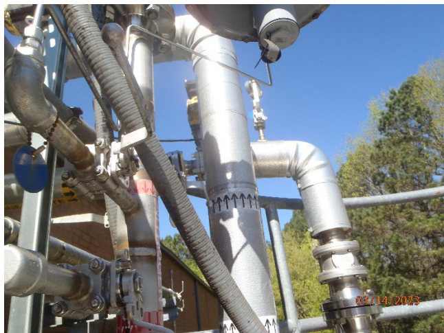
Figure 27: P3140039.JPG: Equipment on the top of the Used Acetone Tank
