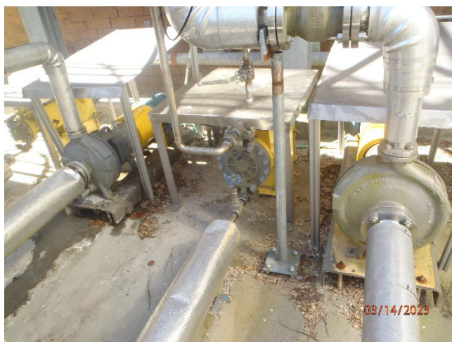
Figure 12: P3140020.JPG: Leaking pump
