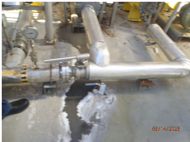
Figure 9: P3140017.JPG: Acetone flowing from actively leaking pump and solidified waste.
