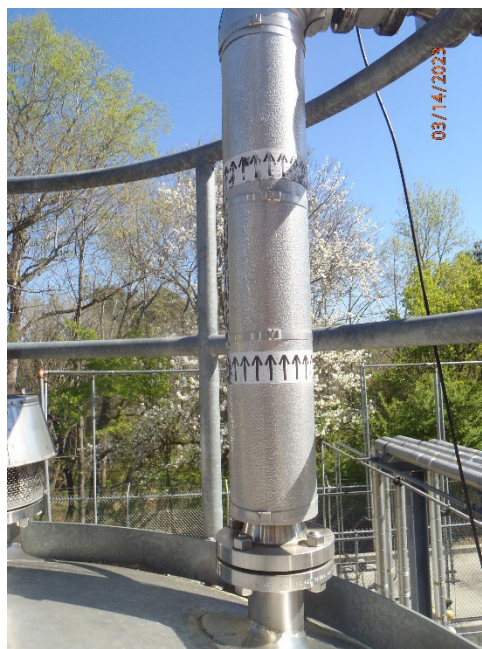
Figure 24: P3140036.JPG: Equipment on the top of the Used Acetone Tank
