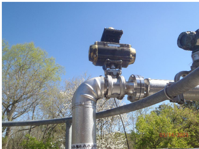
Figure 25: P3140037.JPG: Equipment on the top of the Used Acetone Tank
