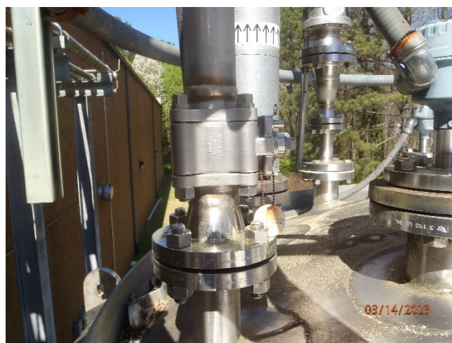
Figure 20: P3140032.JPG: Equipment on the top of the Used Acetone Tank
