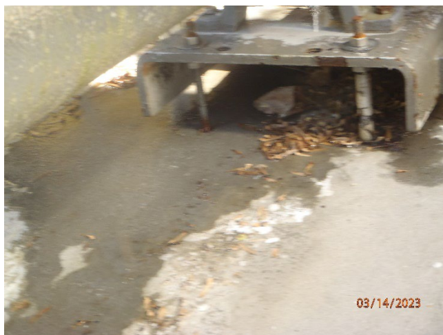
Figure 16: P3140027.JPG: Leaking Pump
