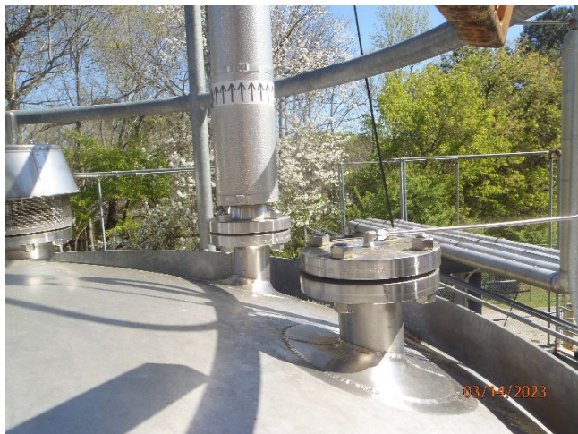
Figure 23: P3140035.JPG: Equipment on the top of the Used Acetone Tank
