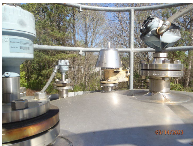
Figure 22: P3140034.JPG: Equipment on the top of the Used Acetone Tank
