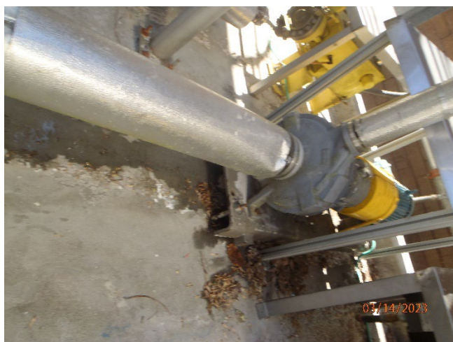
Figure 13: P3140021.JPG: Leaking Pump
