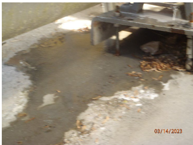
Figure 15: P3140026.JPG: Leaking pump
