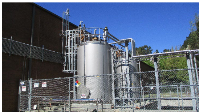
Figure 40: IMG_0070.JPG: Tank Farm Overview
