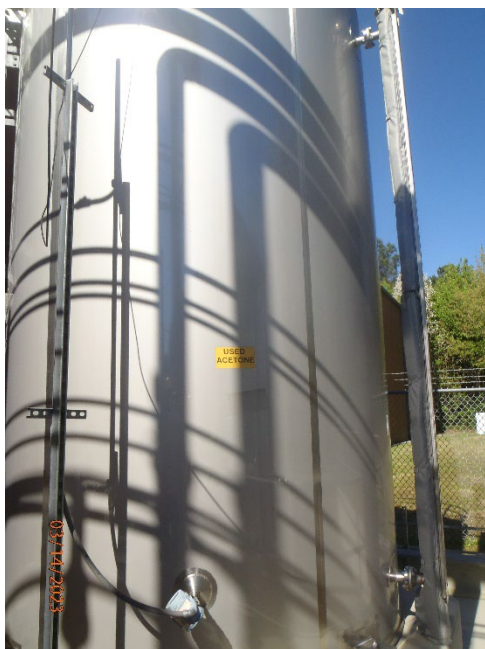
Figure 11: P3140019.JPG: Used Acetone label on tank
