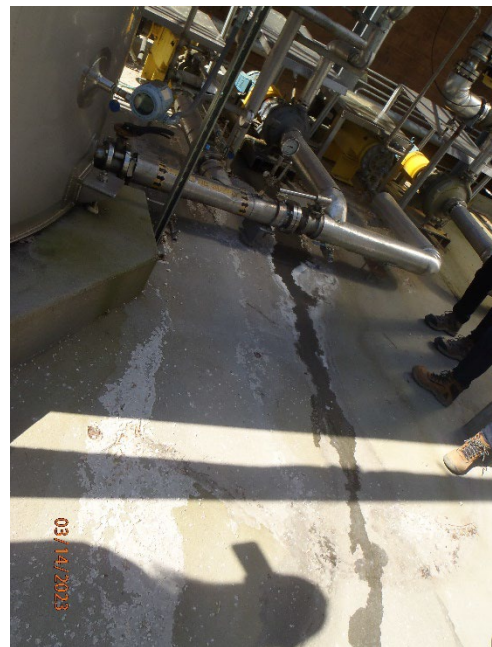
Figure 8: P3140016.JPG: Active leak from pump in secondary containment
