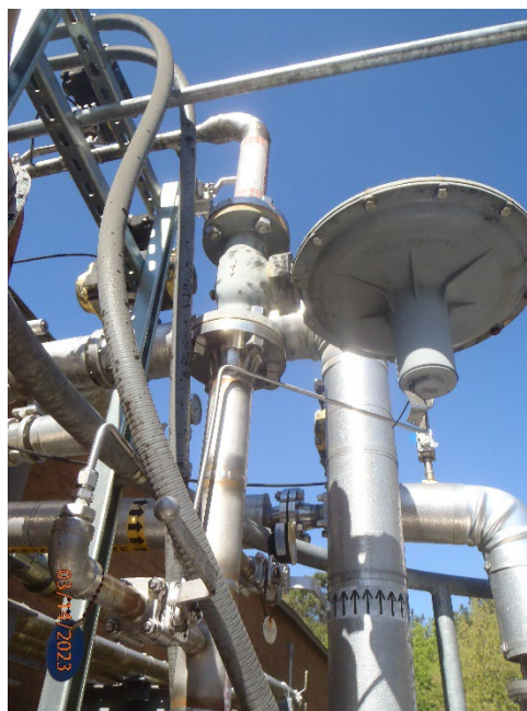
Figure 28: P3140040.JPG: Equipment on the top of the Used Acetone Tank
