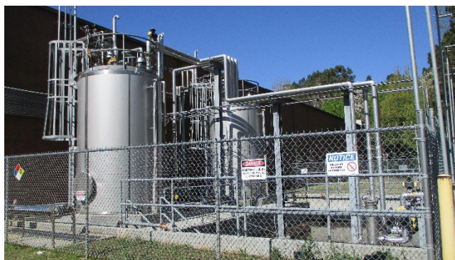
Figure 41: IMG_0071.JPG: Tank Farm Overview
