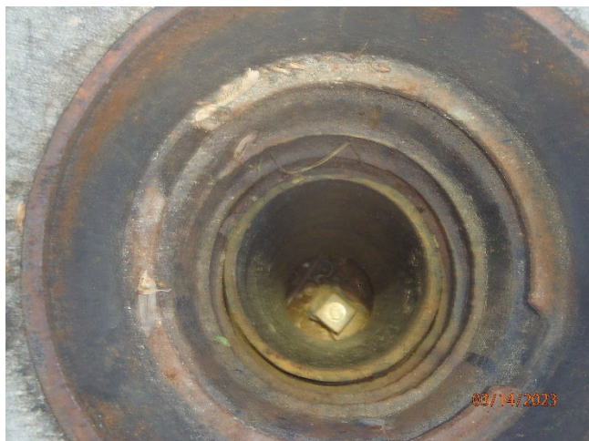
Figure 17: P3140028.JPG: Valve used to control the release of liquid from the Secondary Containment Pit
