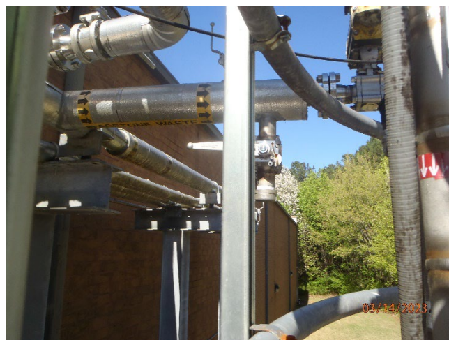
Figure 30: P3140042.JPG: Equipment on the top of the Used Acetone Tank
