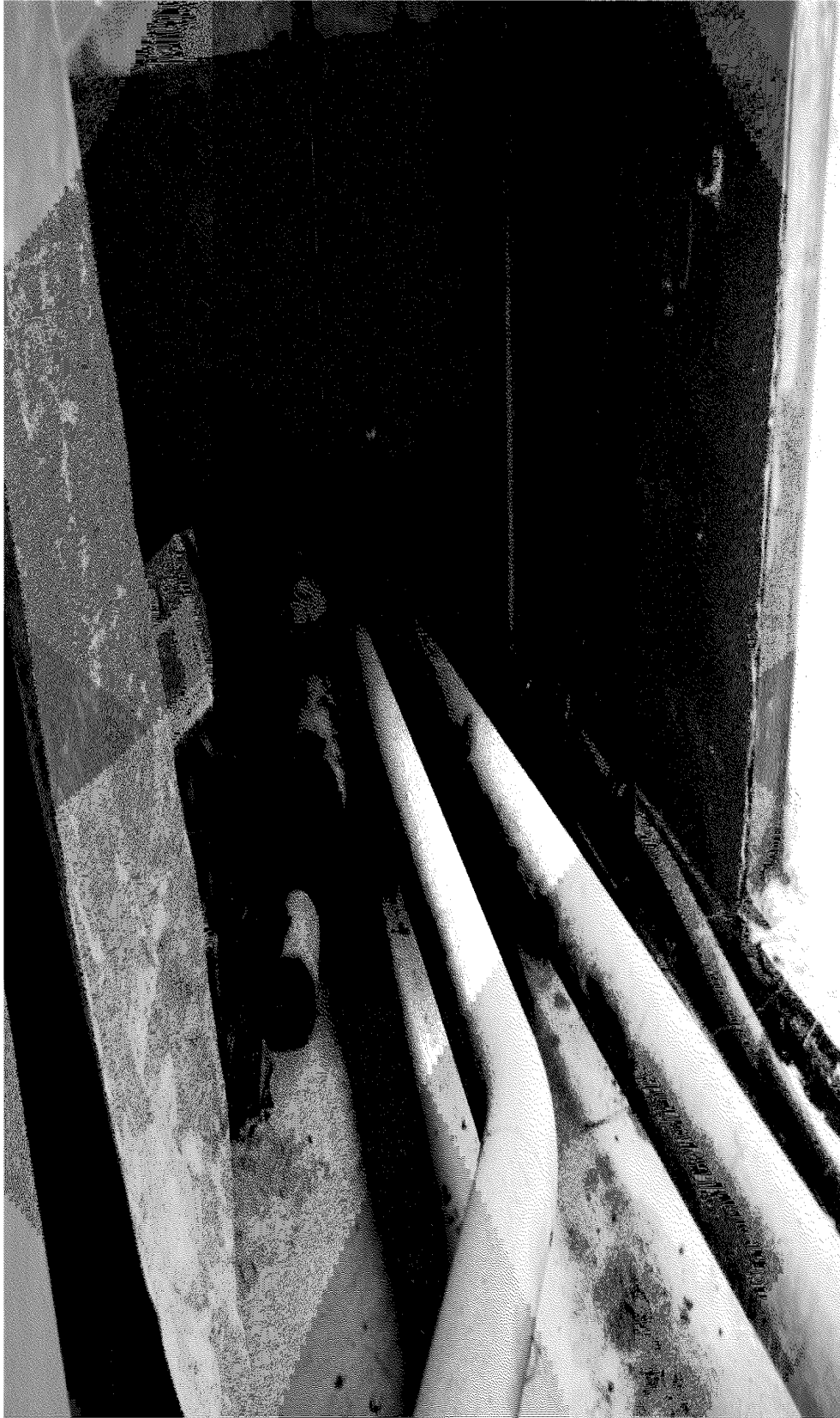
Inside pump house
