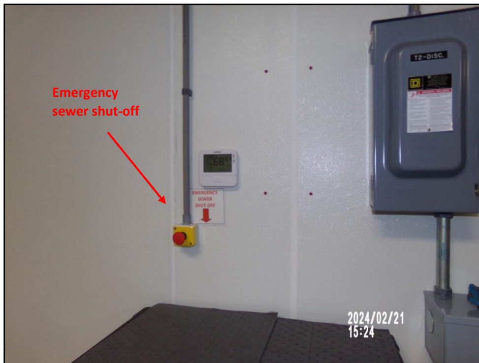
Photo 1: Emergency shut off button located in the facility's pretreatment room.
