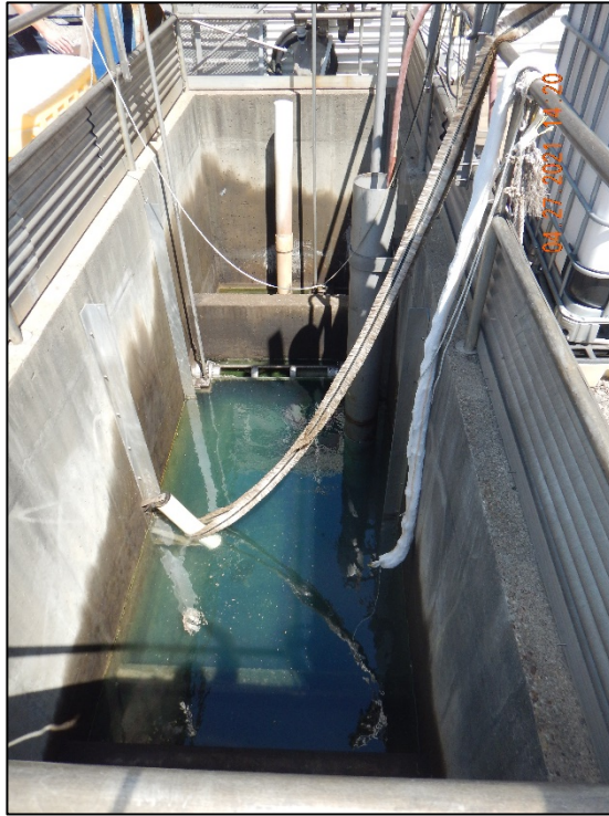
DSCN2379. View, facing east, of an oil/water separator in the Outfall 003 clear water sewer system area.
