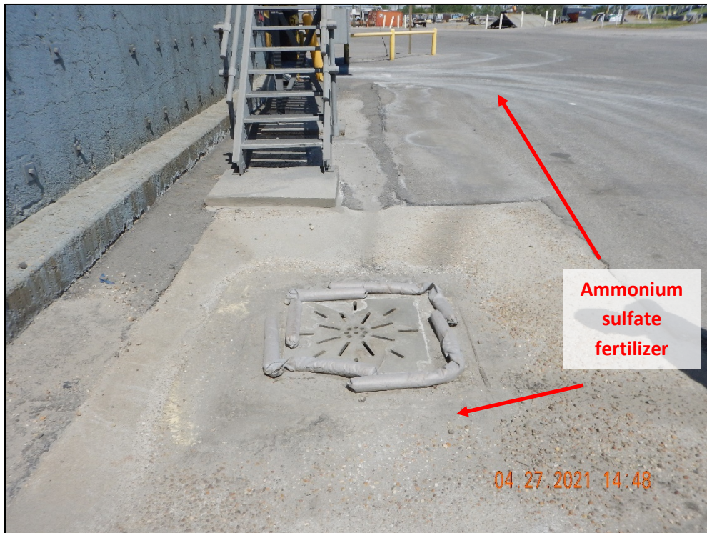
DSCN2386. View, facing east, of an inlet flowing to Outfall 004. Note the presence of ammonium sulfate fertilizer on the ground surrounding the inlet.
