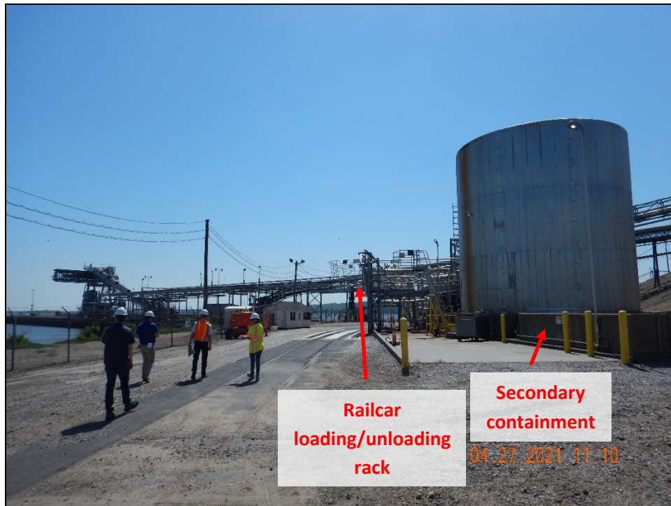
DSCN2338. View, facing south, of two oleum tanks in secondary containment and a railcar loading/unloading rack.
