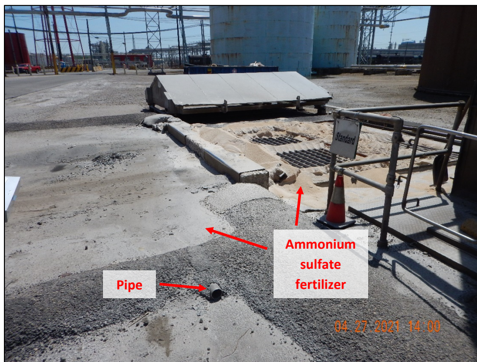
DSCN2376. View, facing south, of ammonium sulfate fertilizer pit with a small pipe through the bermed unloading area. Note the presence of fertilizer on the ground in the area.
