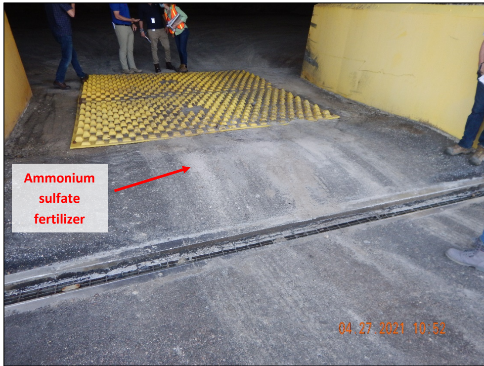
DSCN2329. View, facing south, of the entryway to the fertilizer storage warehouse. Note the heavy fertilizer tracking over and inside the storm drain in the entryway.
