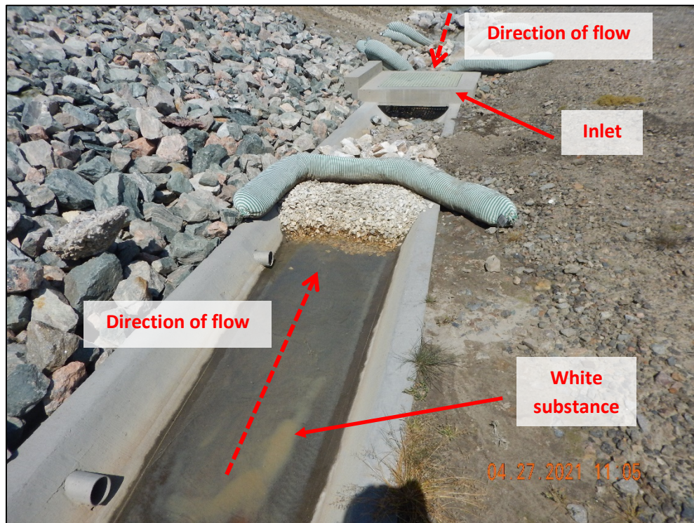
DSCN2335. View, facing north, of the stormwater inlet from DSCN2336. Note the presence of the same unknown white substance in the water upgradient of the inlet.
