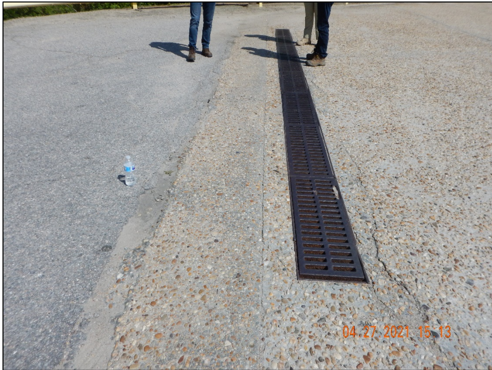
DSCN2397. View, facing east, of a stormwater drain in the parking lot of the drum unloading area. This drain flows to the nearby stormwater Outfall 908.
