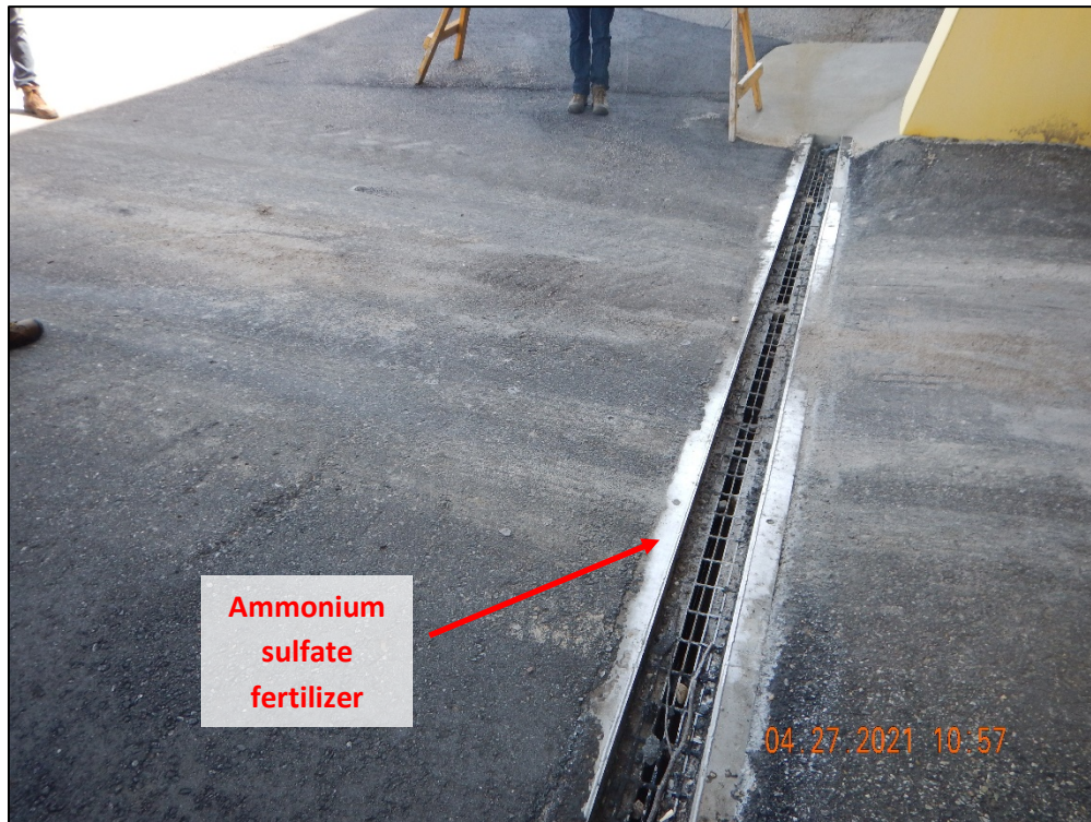
DSCN2332. Alternate view, facing east, of the entryway to the fertilizer storage warehouse. Note the fertilizer in and around the storm drain to Outfall 906.
