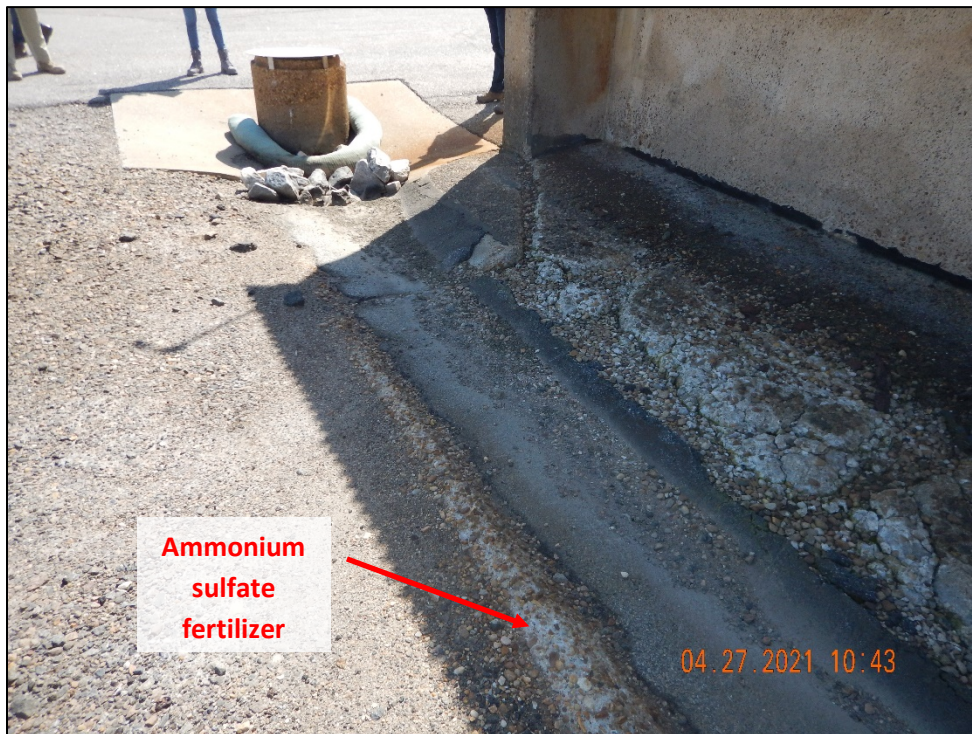
DSCN2325. View, facing east, of the ditch and stormwater inlet at the northeast corner of the northernmost fertilizer warehouse. Note the white fertilizer staining in the ditch.
