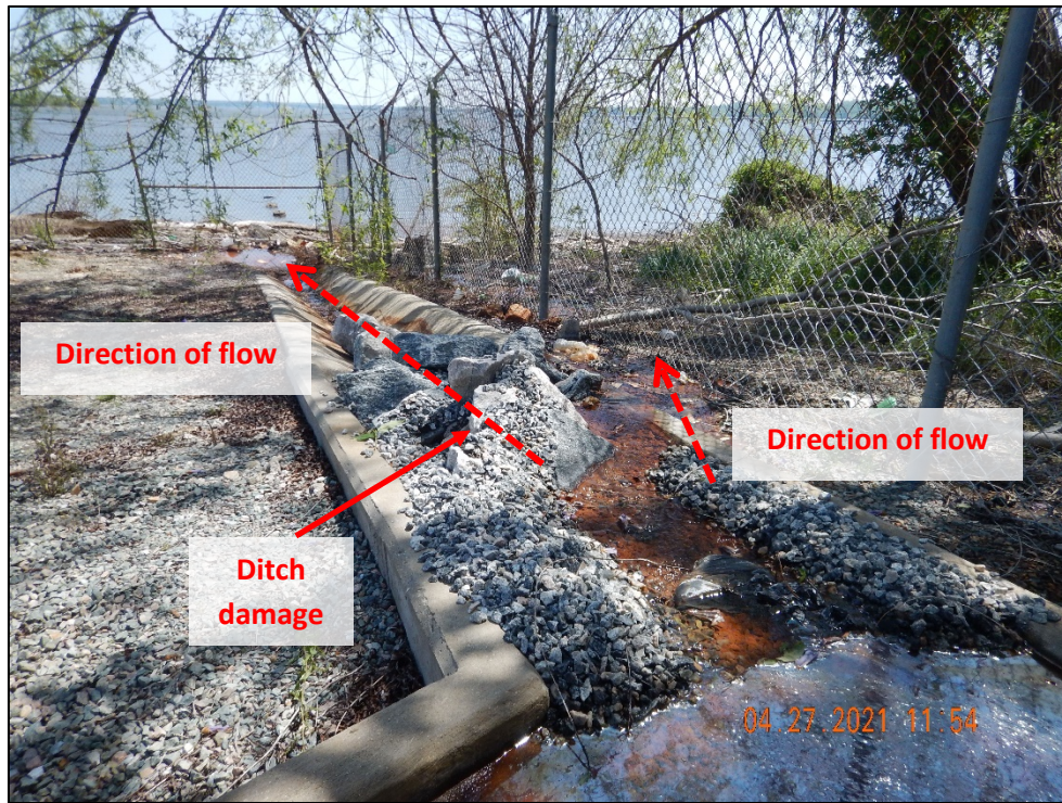
DSCN2359. View, facing east, of the red dry-weather flow running into the James River. Note the damage to the concrete ditch and flow spilling over the side of the ditch.
