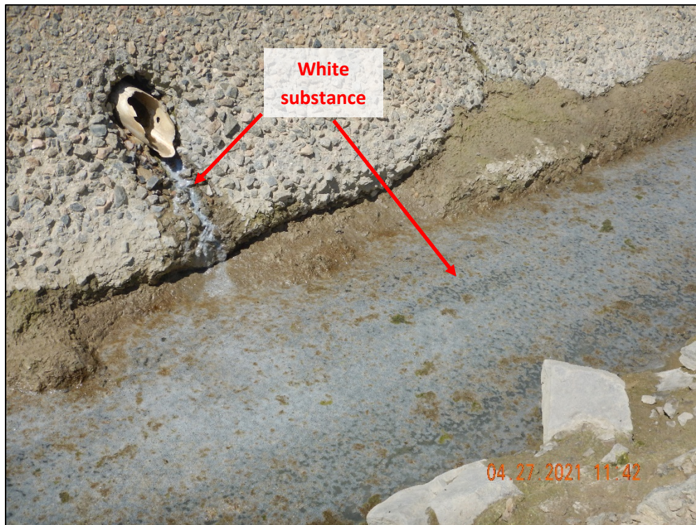
DSCN2350. View, facing northwest, of a small pipe in the side of the steep slope draining an unknown white liquid into the ditch to Outfall 905.
