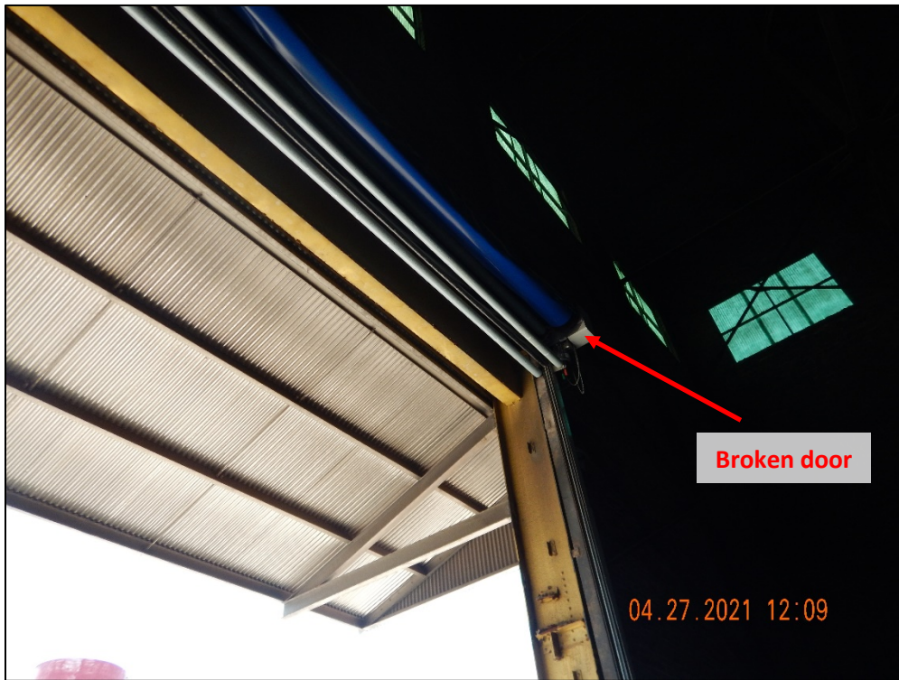
DSCN2368. View of a fast-closing door in the entryway to the fertilizer warehouse. Note that it was not functioning at the time of the EPA inspection.
