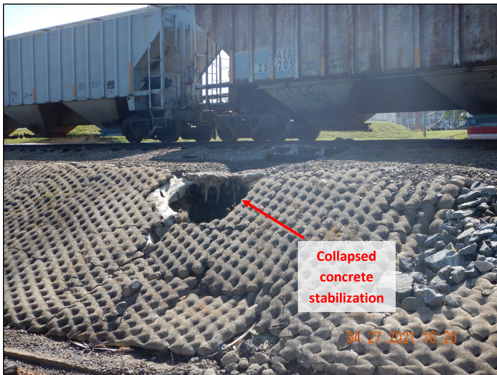
DSCN2318. View, facing southeast, of a collapsed portion of the concrete stabilization on the slope between the rail tracks and the north perimeter fence.
