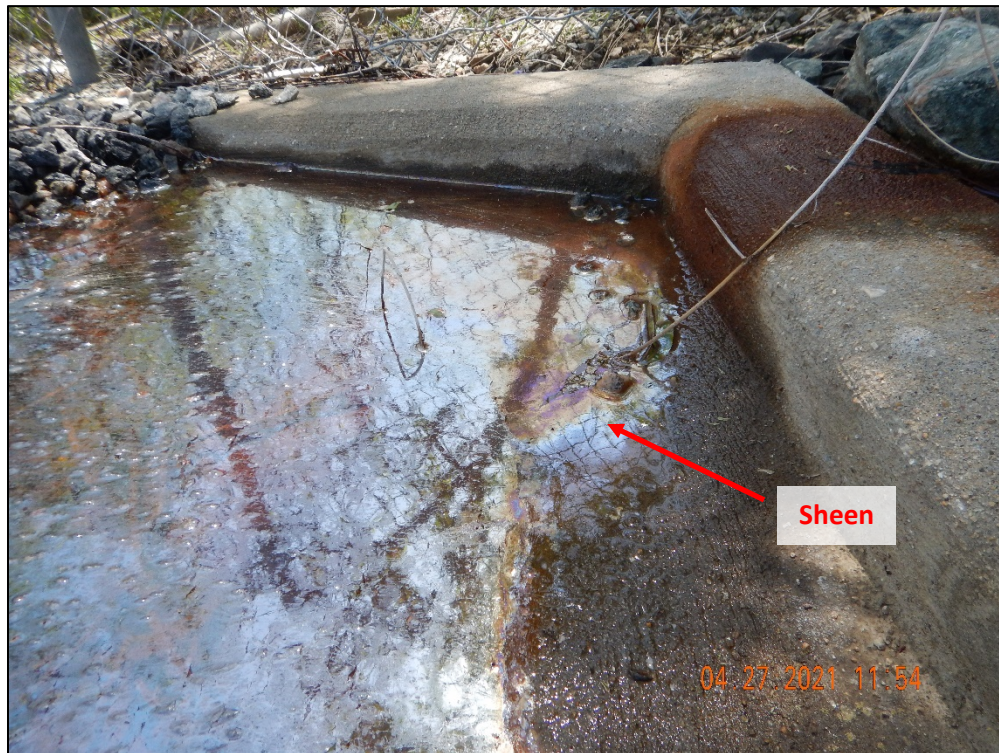
DSCN2360. View of surface sheen at the end of the concrete ditch from DSCN 2358 and DSCN 2359.
