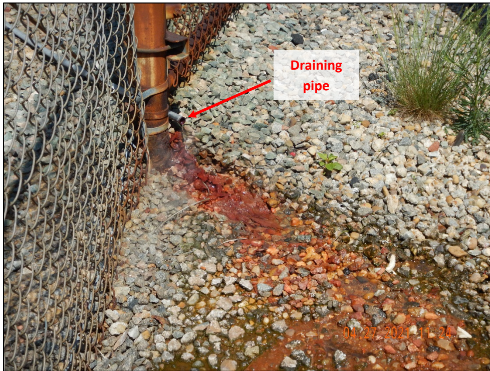
DSCN2342. View of a small pipe draining a steaming liquid onto the shoreline of the James River. Facility representatives stated it was a low-pressure steam drain.
