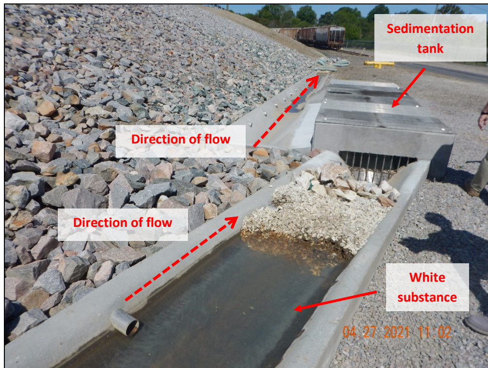
DSCN2333. View, facing north, of a sedimentation tank to the south of the stormwater inlet used for Outfall 906 sampling. Note the presence of an unknown white substance in the water.
