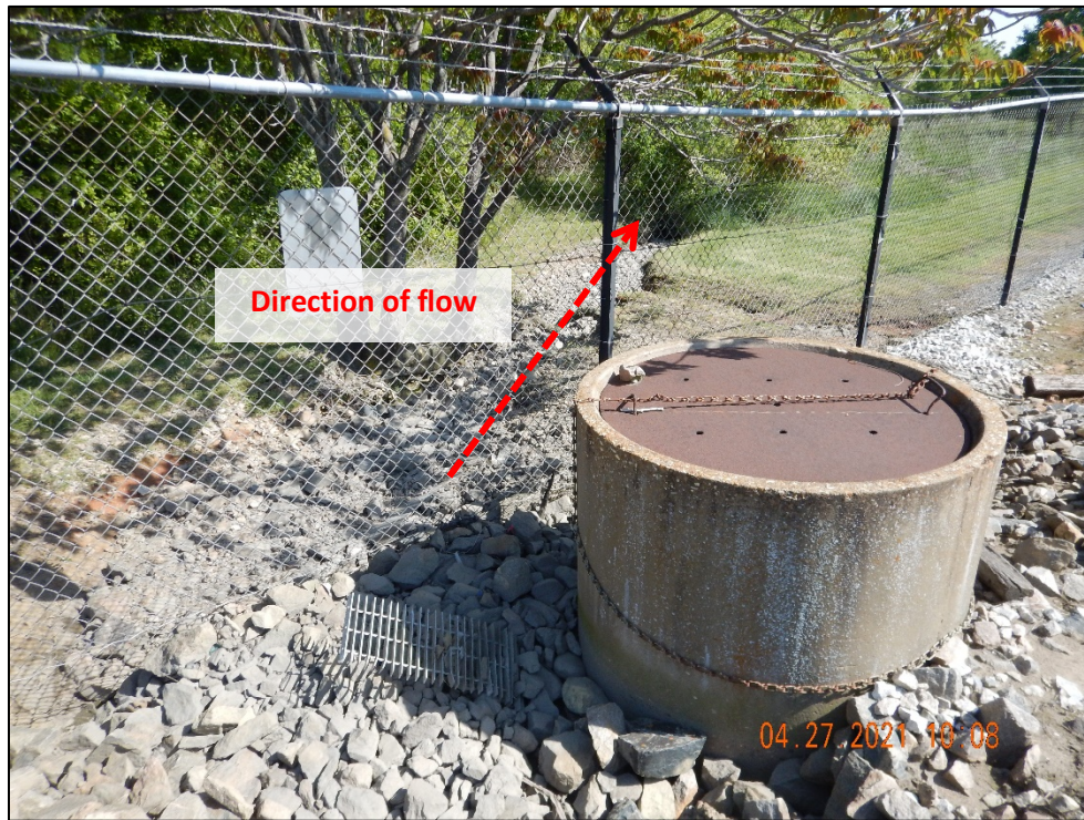
DSCN2311. View, facing northeast, of the manhole where Facility representatives collect samples for Outfall 912. Note the signs of sheet flow beyond the north perimeter fence.
