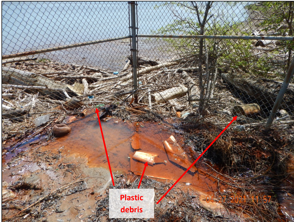
DSCN2361. View, facing southeast, of the area between the end of the concrete ditch and the James River. Note the presence of plastic debris on the ground.
