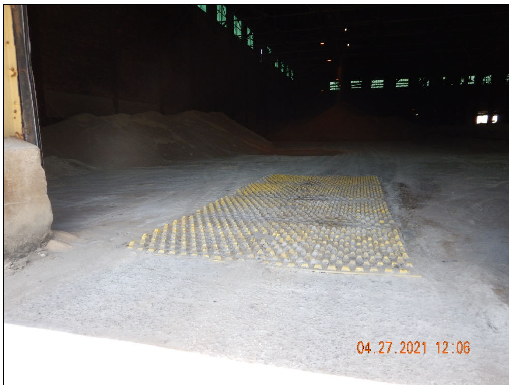
DSCN2366. View of the foreign object debris system in the entryway to the warehouse from DSCN 2364 and DSCN 2365. The debris system was heavily laden with fertilizer.
