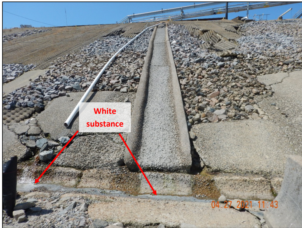
DSCN2351. View, facing west, of a concrete drainage ditch running down the steep slope. Note the presence of an unknown white substance in the ditch.
