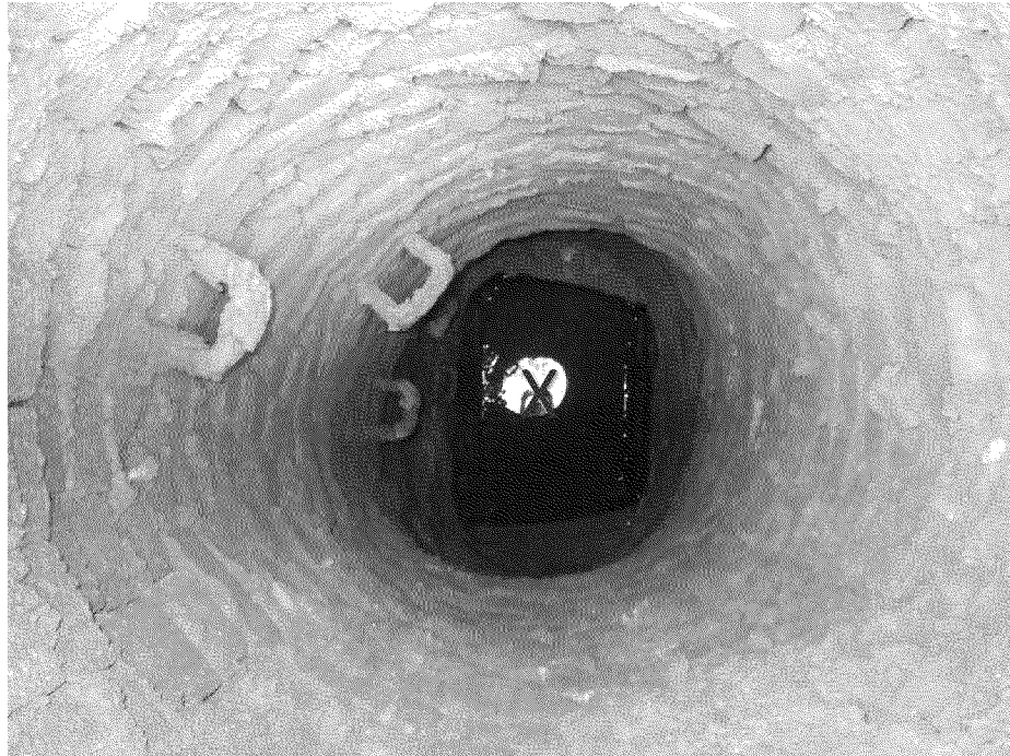
Photo 3: MH5380 (photo taken 10/2/2024 at approx. 10:26) Manhole located near Tewksbury St, discharging into the Merrimack River. Sample points are indicated by a red X.
