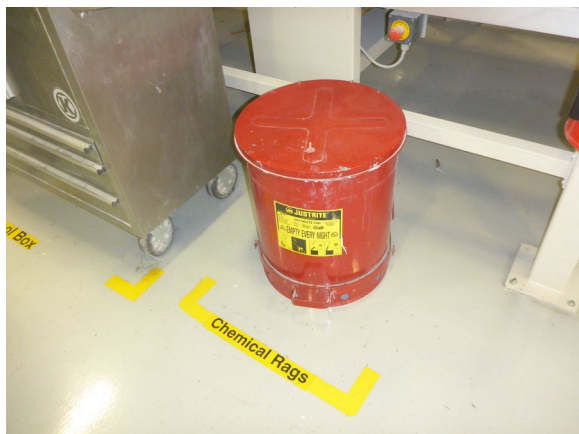
Photo 4: One of at least seven flip-top flammable cans used to accumulate dirty rags and wipes generated throughout the Solvent-Based Finishing Program as hazardous waste solids. Each of the flip-top flammable cans was labeled as oily waste, but none was labeled with the words “hazardous waste” or with an indication of the ignitable or toxic hazards of its contents. This container was observed near the Flat-Line Automated System.
