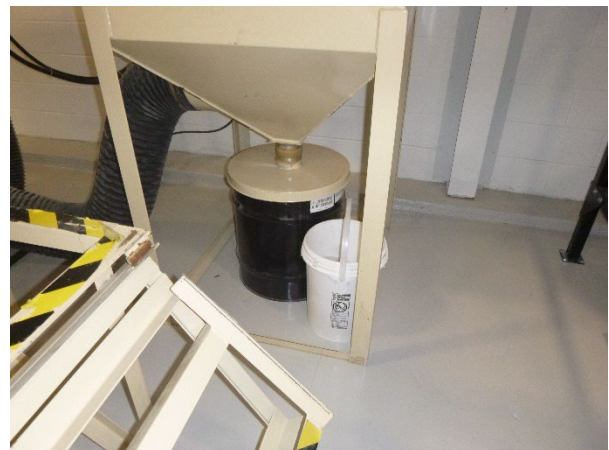
Photograph 26: Building 717 - Blast Media Booths.
