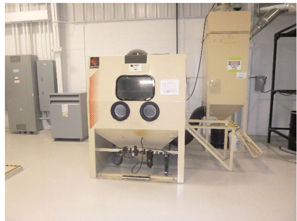
Photograph 25: Building 717 - Blast Media Booths.
