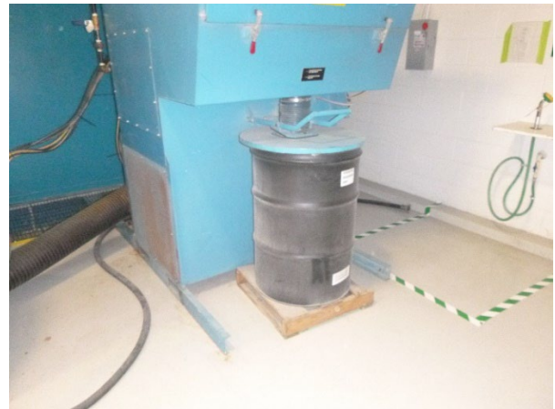
Photograph 29: Building 717 - Blast Media Booths.
