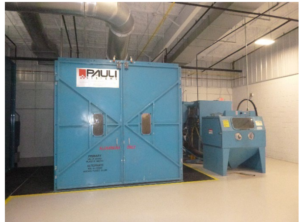
Photograph 24: Building 717 - Blast Media Booths.
