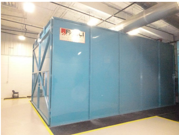
Photograph 28: Building 717 - Blast Media Booths.
