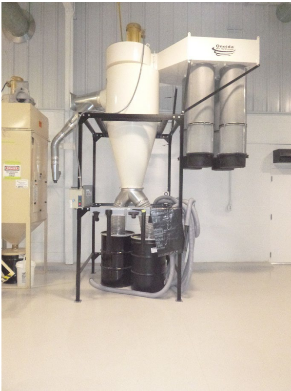
Photograph 27: Building 717 - Blast Media Booths.
