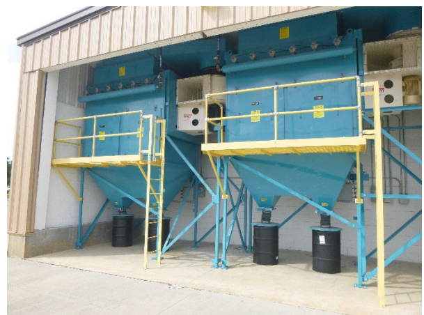
Photograph 30: Building 717 - Blast Media Booths.
