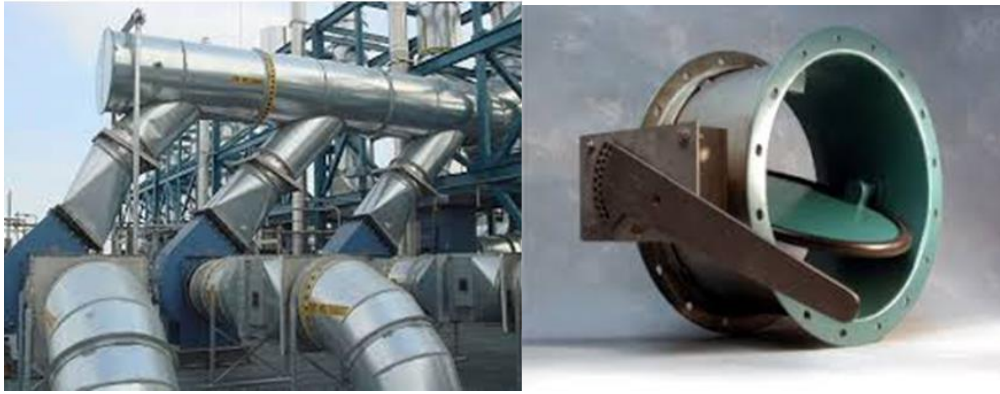
Figure 21: Exhaust system components used for corrosive chemicals such as acid and hydrogen fluoride gas (image on the left courtesy of GlobalFoundries) (Fab-Tech 2023).
