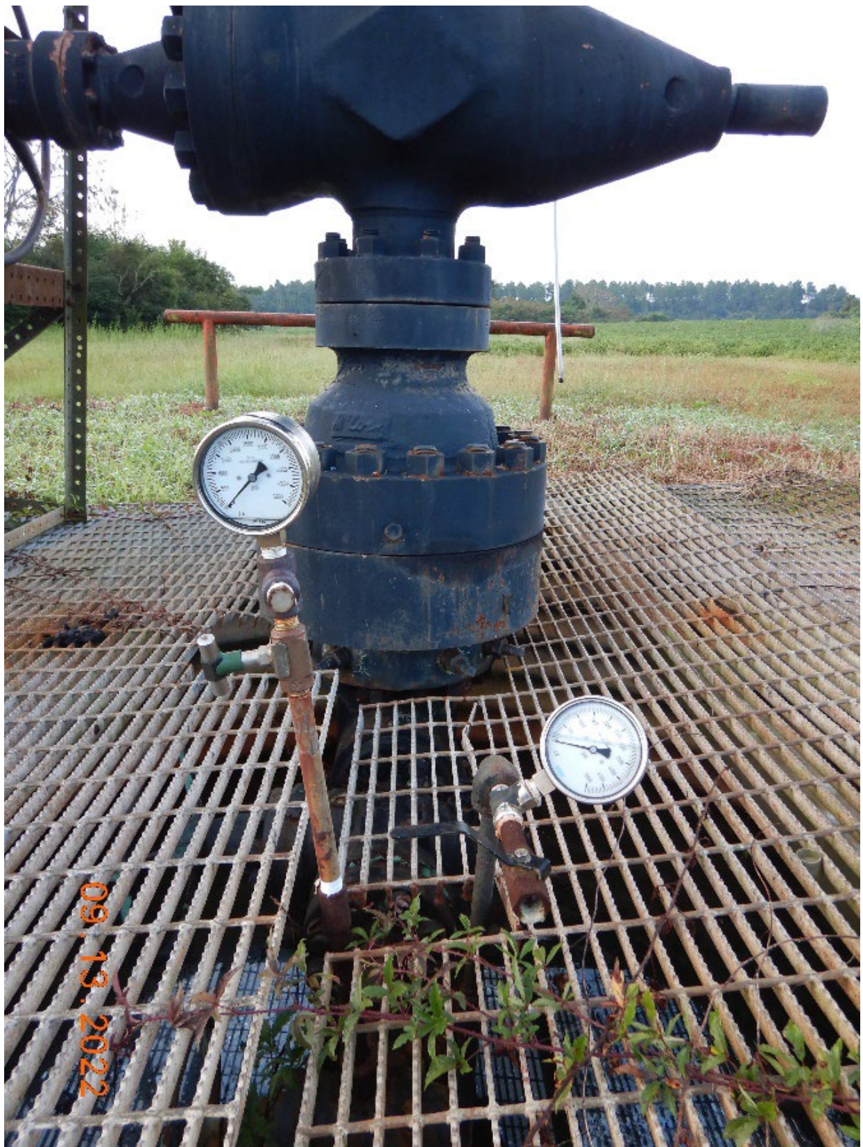
Photograph 3: Looking south, closeup view of surface casing pressure gauge (0 psi) and production casing pressure gauge (0 Psi).
