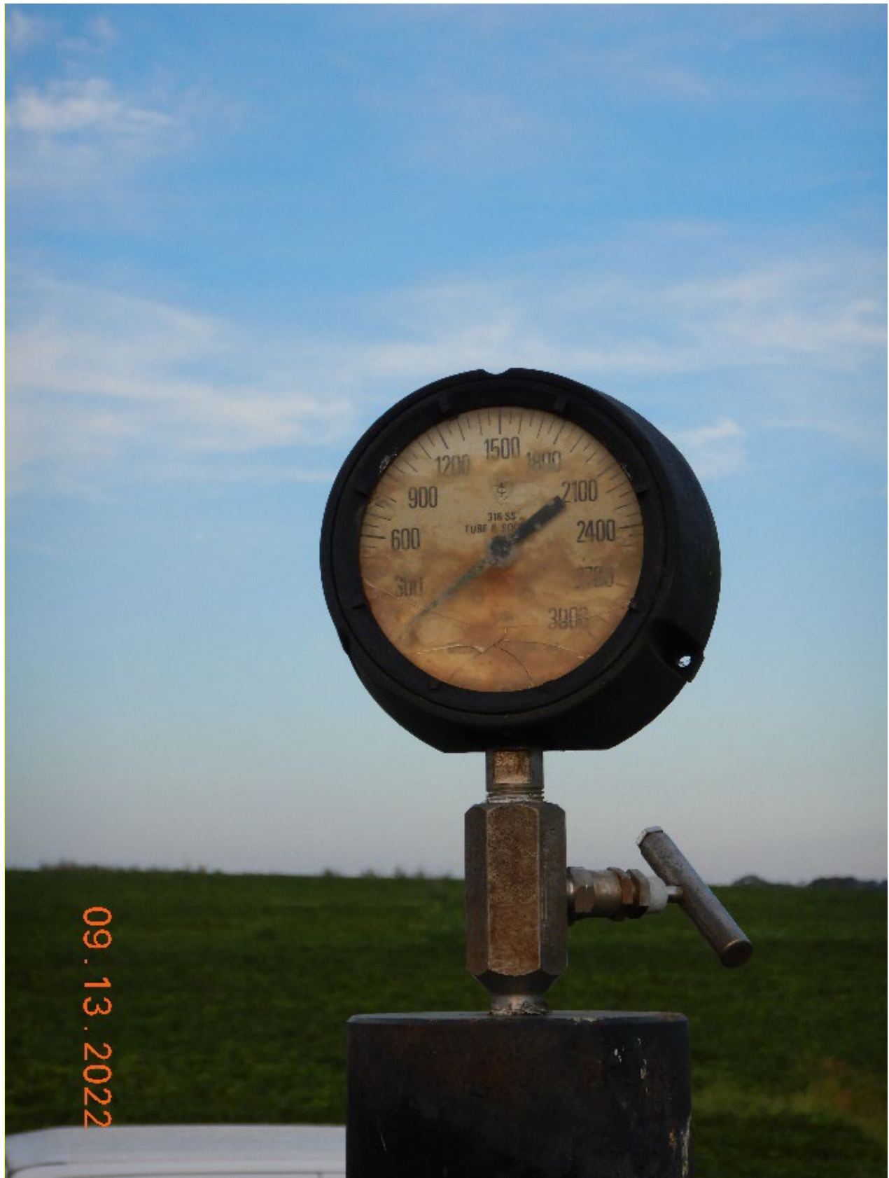
Photograph 4: Looking west, closeup view of internal pressure gauge reading 0 psi.
