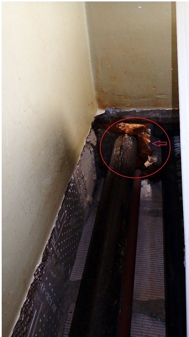
Figure 14: Pipe in second floor Janitor Closet/Slop Sink. Annotated is the paper material observed by EPA Inspectors.
