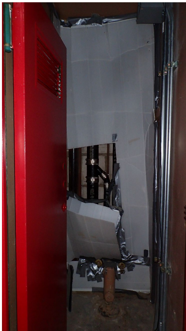
Figure 13: Cardboard cover for wall cavity in Janitor Closet/Slop Sink on the third floor. The cover had fallen prior to EPA Inspectors arriving to observe. Note the pipes in the cavity are free of insulation.
