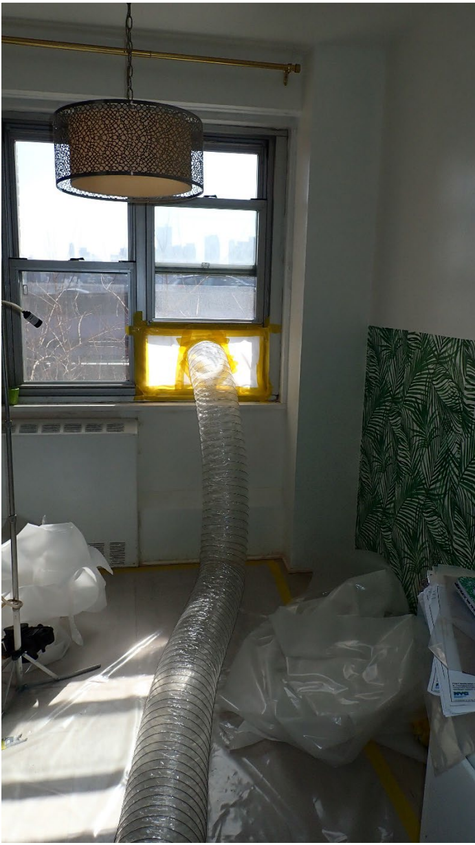
Figure 16: Exhaust piping leading to open air outside of the apartment.
