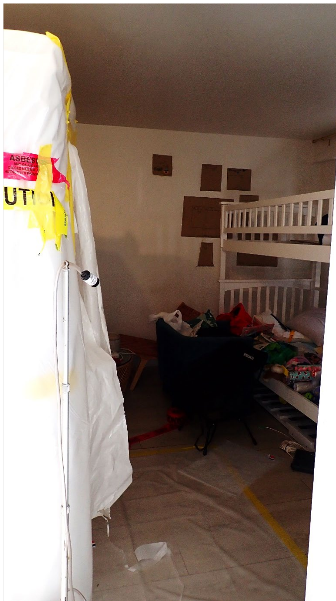
Figure 18: Back (exit) of the decon area.
