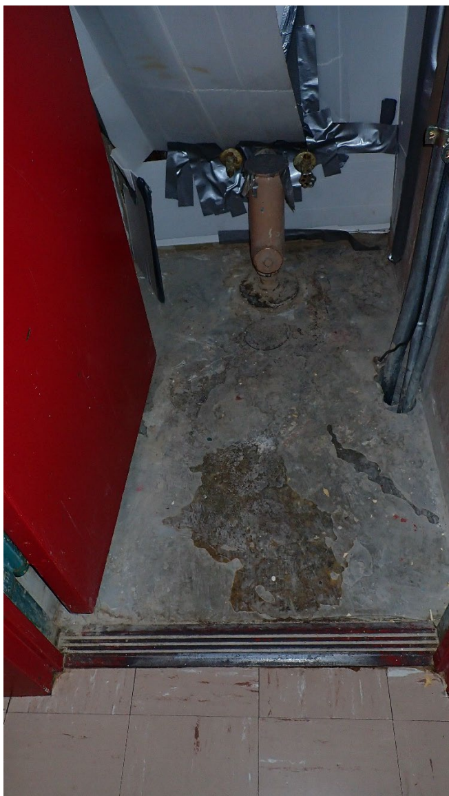
Figure 12: Third floor Janitor Closet/Slop Sink. Note the lack of debris on the floor.
