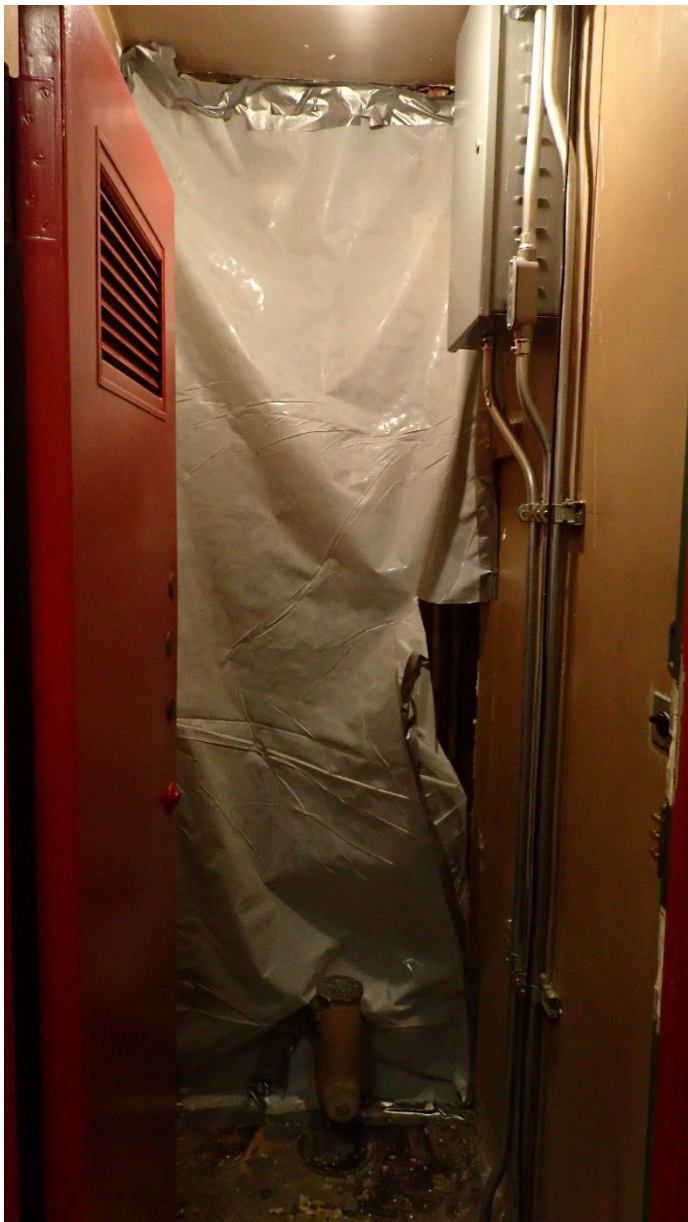
Figure 9: Plastic sheet observed covering the cavity where asbestos abatement was done previously. Janitor Closet/Slop Sink, fourth floor.
