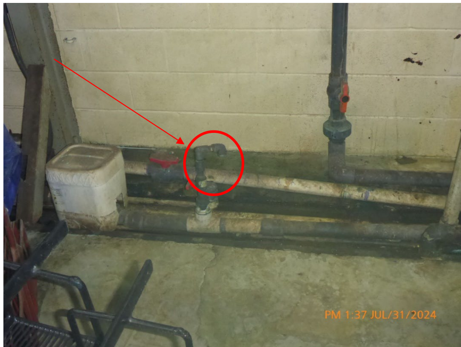
Photograph 7: Grab sample location at SMG. Arrow is pointing to the pipe where samples are collected (circled).
