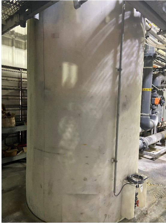
Photograph 4: Reactor 3 holding tank – microfilter feed tank at Dynamet. Photo provided by the Dynamet representative following the inspection.
