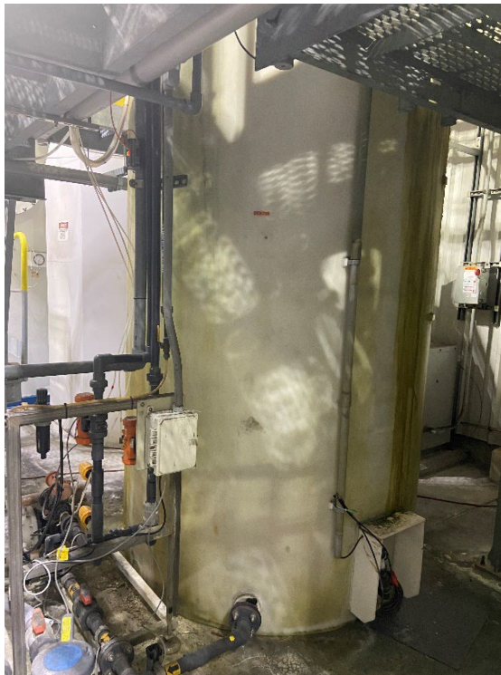
Photograph 3: Reactor 1 mix tank at Dynamet. Photo provided by the Dynamet representative following the inspection.
