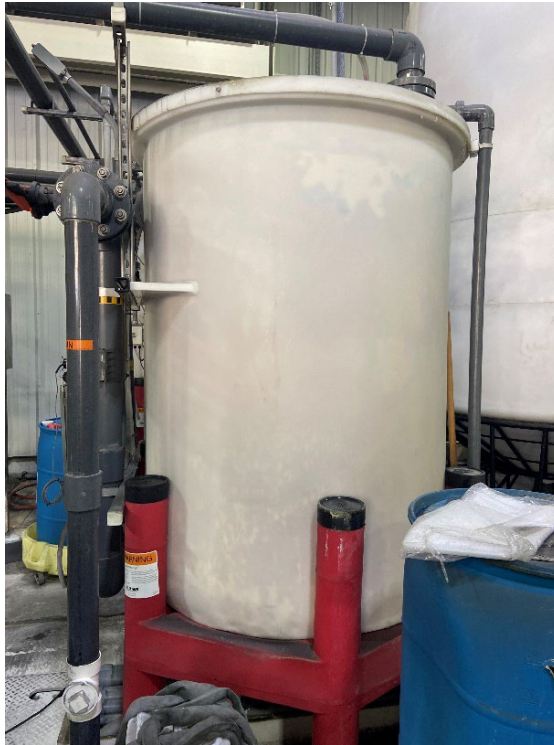
Photograph 2: Final pH and flow monitoring tank at Dynamet. Photo provided by the Dynamet representative following the inspection.
