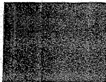
Visible joints —taped or filled joints in dry wall construction showing through finish coat.
