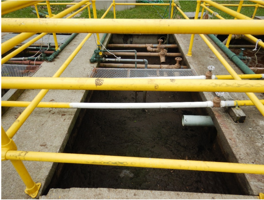
12: DSCN0190 Description: first sludge tank Location: WWTP Camera Direction: southwest Date/Time: 6/9/2021 12:01
