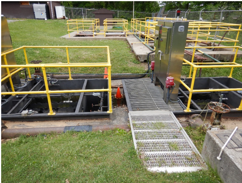
7: DSCN0185 Description: sand filters units (in foreground), note unit at left has been lifted out of the ground Location: WWTP Camera Direction: southwest Date/Time: 6/9/2021 11:48
