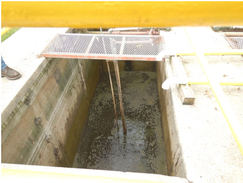
13: DSCN0191 Description: empty sludge tank Location: WWTP Camera Direction: southwest Date/Time: 6/9/2021 12:01
