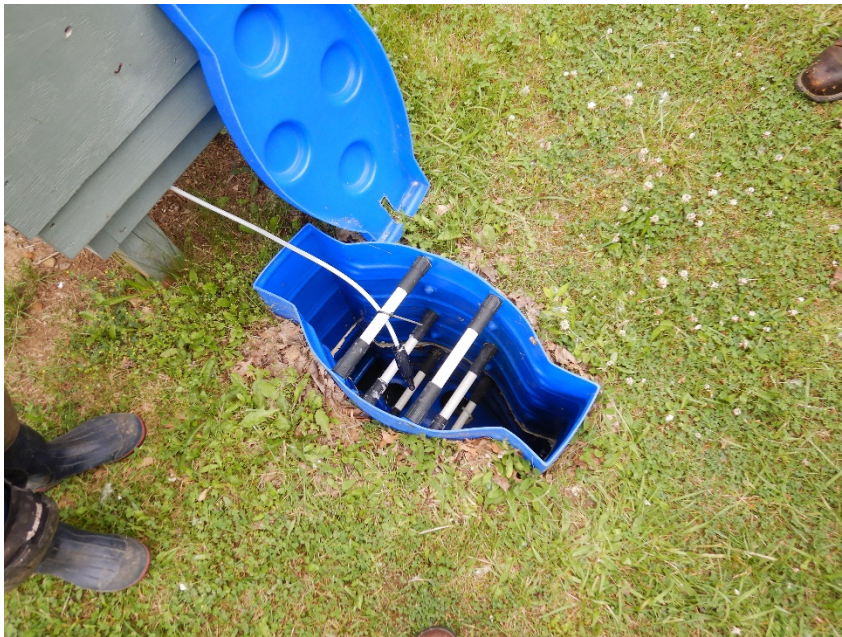
9: DSCN0187 Description: Dechlorination pit Location: WWTP Camera Direction: ground Date/Time: 6/9/2021 11:48
