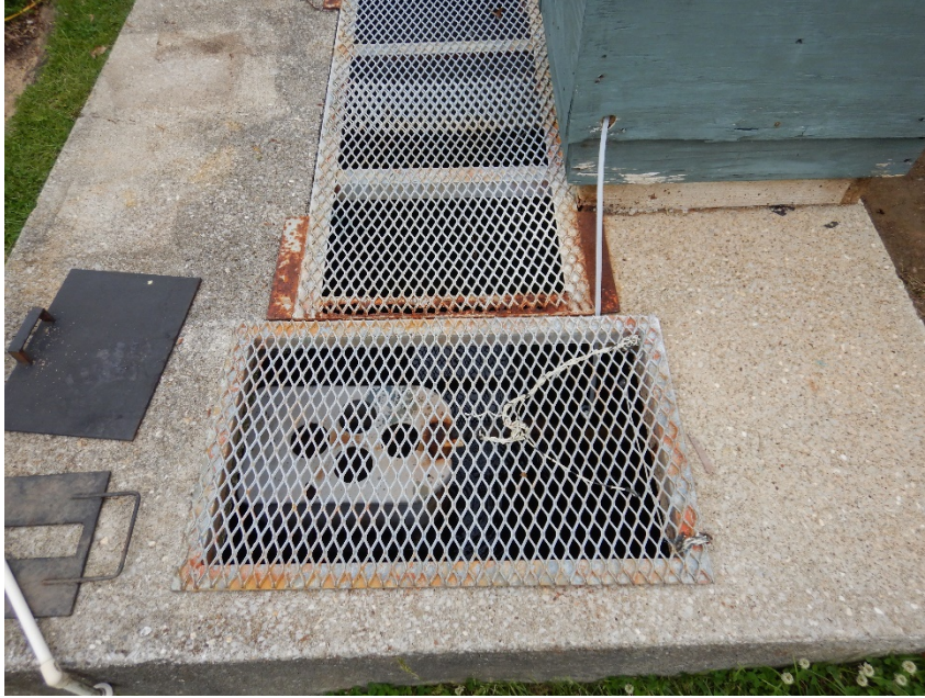
8: DSCN0186 Description: Chlorination tank Location: WWTP Camera Direction: ground Date/Time: 6/9/2021 11:48
