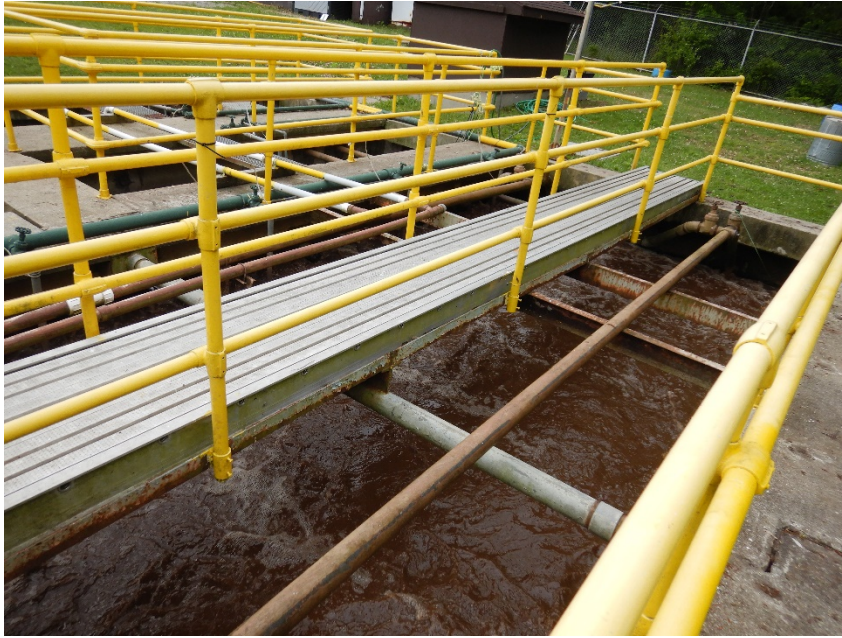
4: DSCN0182 Description: Aeration tank Location: WWTP Camera Direction: southwest Date/Time: 6/9/2021 11:12
