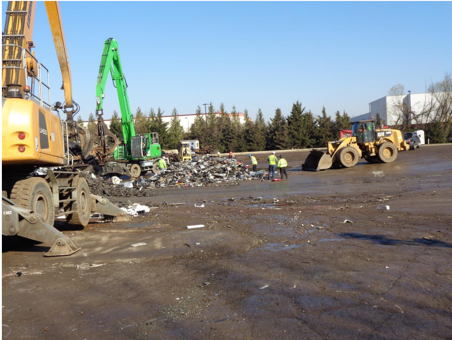
Hand sorting a newly dropped load of scrap. Note red fire extinguisher on the ground.
