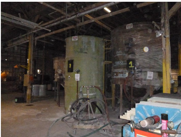
Photograph 9: Wastewater Treatment Tanks.
