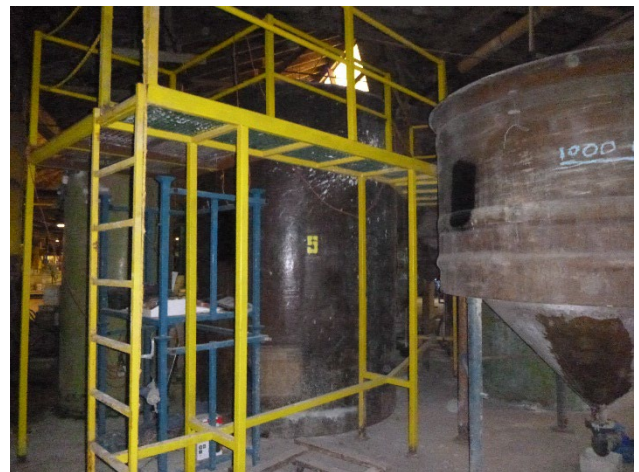
Photograph 12: Wastewater Treatment Tanks.
