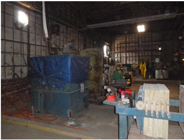
Photograph 13: Wastewater Treatment Tanks.
