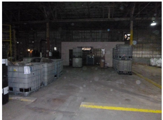
Photograph 6: Compressor Room CAA.
