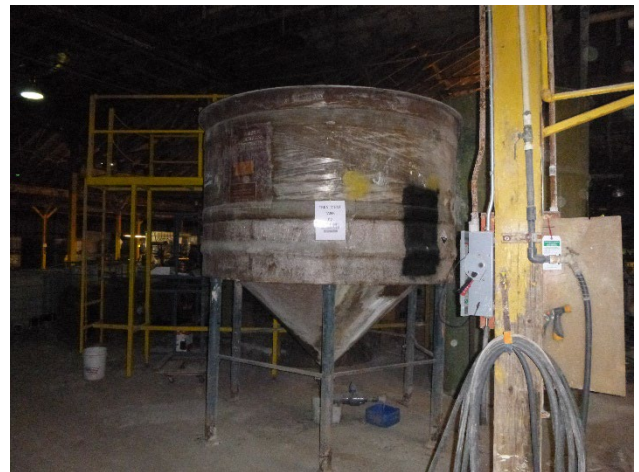
Photograph 11: Wastewater Treatment Tanks.
