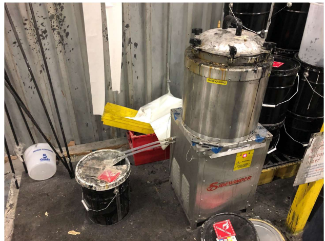
Photo 5: Solvent Recovery System 1.
