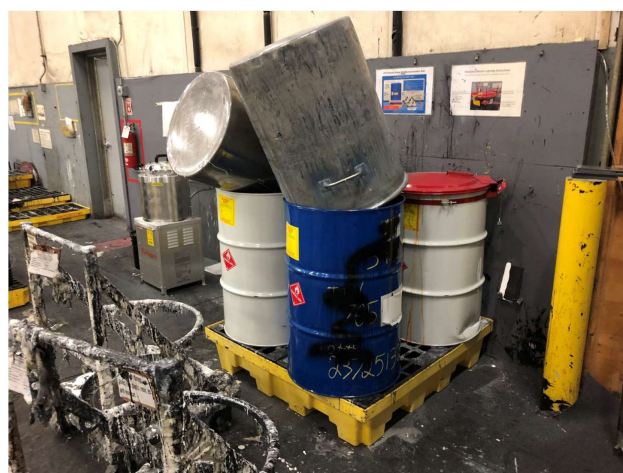
Photo 28: Solvent Recovery System 2 and Pots draining into containers.
