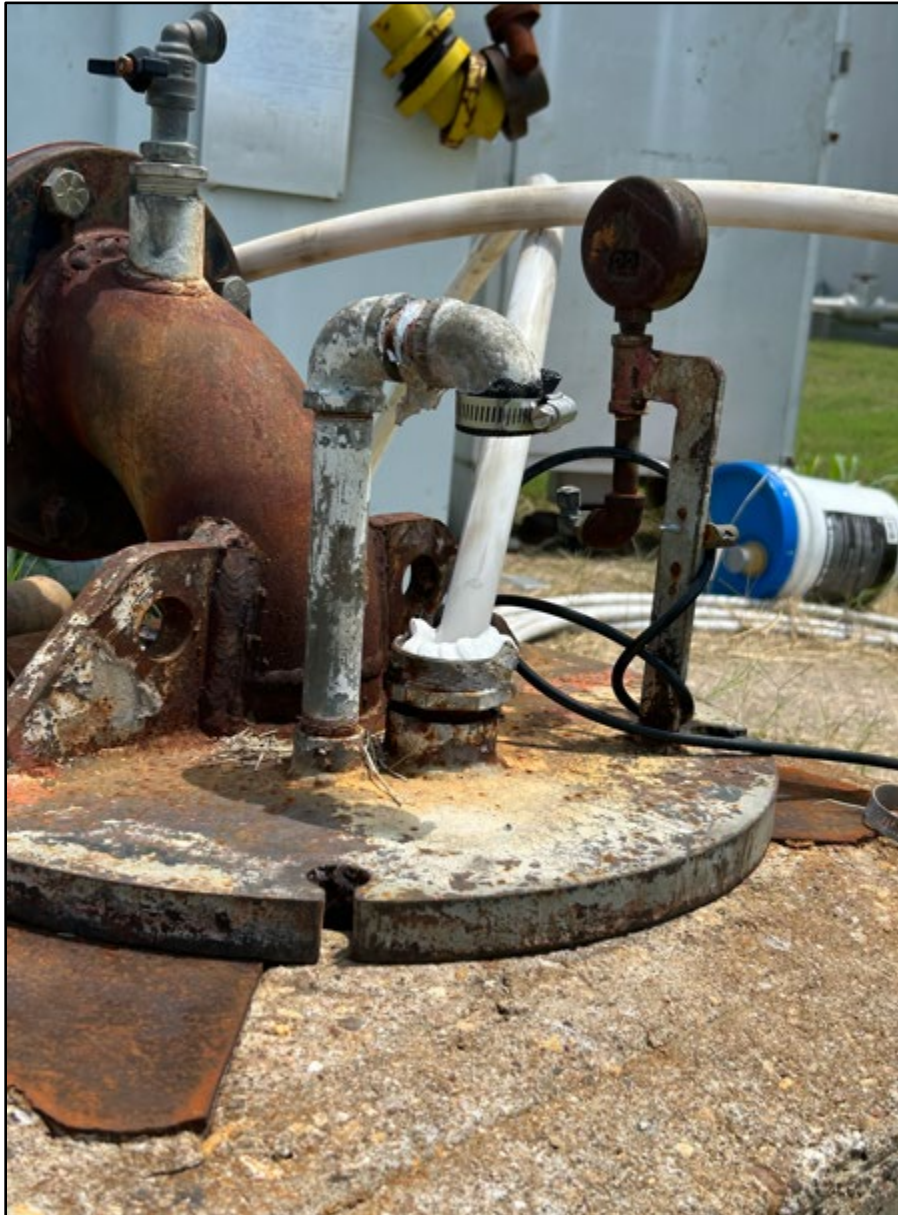
Description: Plant 6. Well No. 4 wellhead with conduit penetration sealed and vent screen installed (Observation 10). Photo received June 6, 2025.
