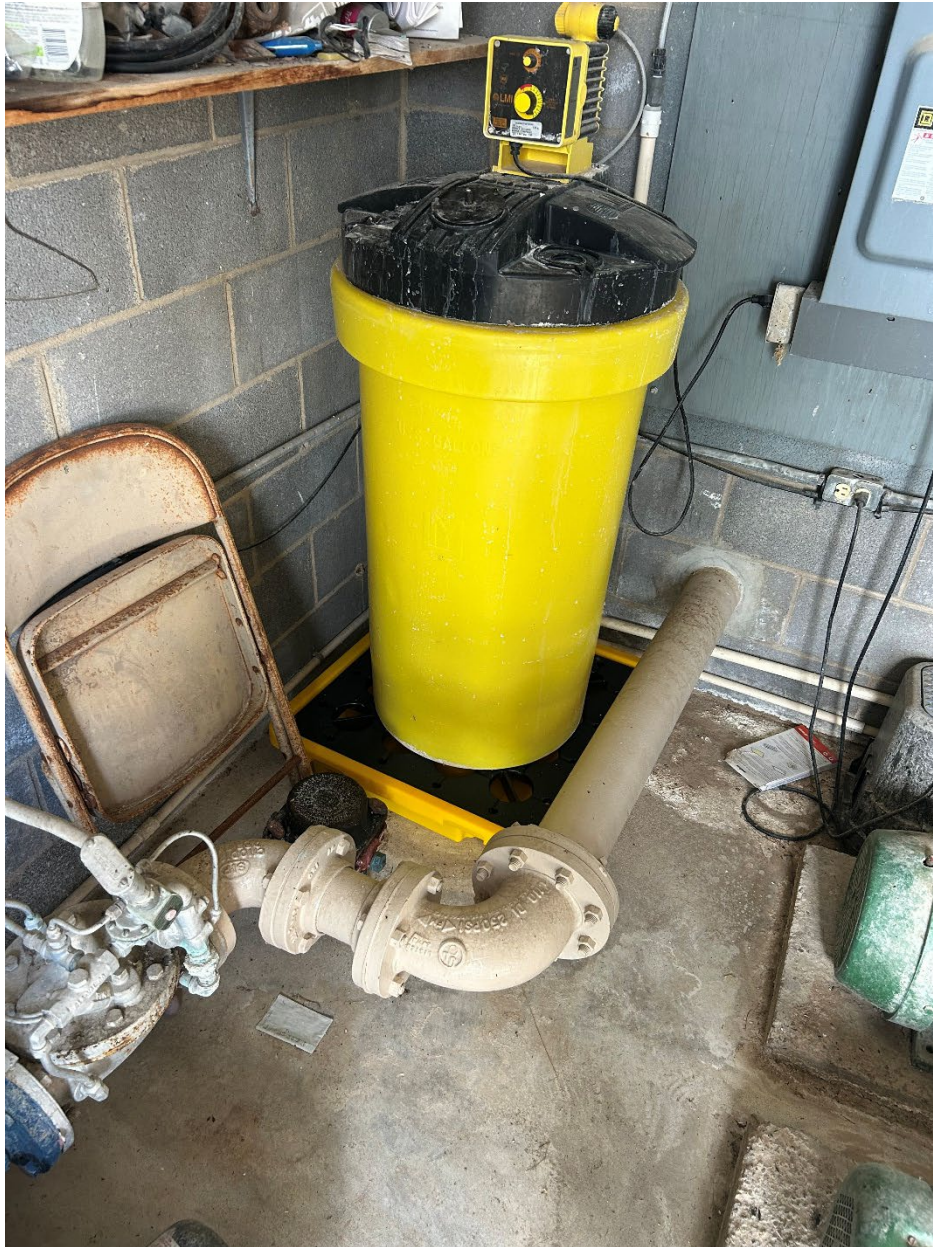
Description: Containment provided for polyphosphate feed barrel at Plant 6 (Observation 7). Photo received June 24, 2025.
