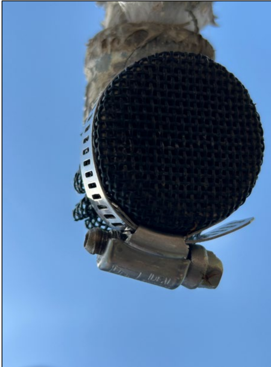
Description: Plant 6. Vent with screen installed on Well No. 4 (Observation 10). Photo received June 6, 2025.
