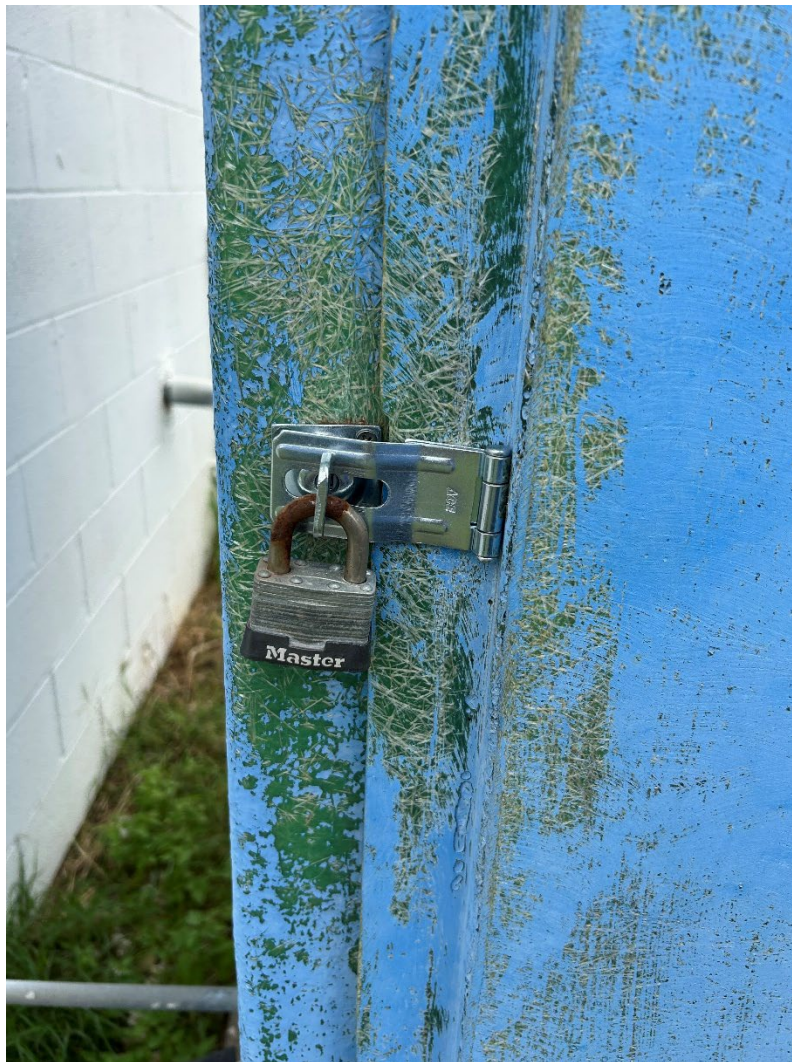
Description: Lock installed on Plant 11 chlorine gas room. Photo received June 20, 2025.
