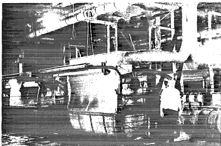
Fig. 3. Placing a curtain in front of the "dolly washer" reduced the opening one half and almost doubled the velocity of air flow at the bottom of the opening.
