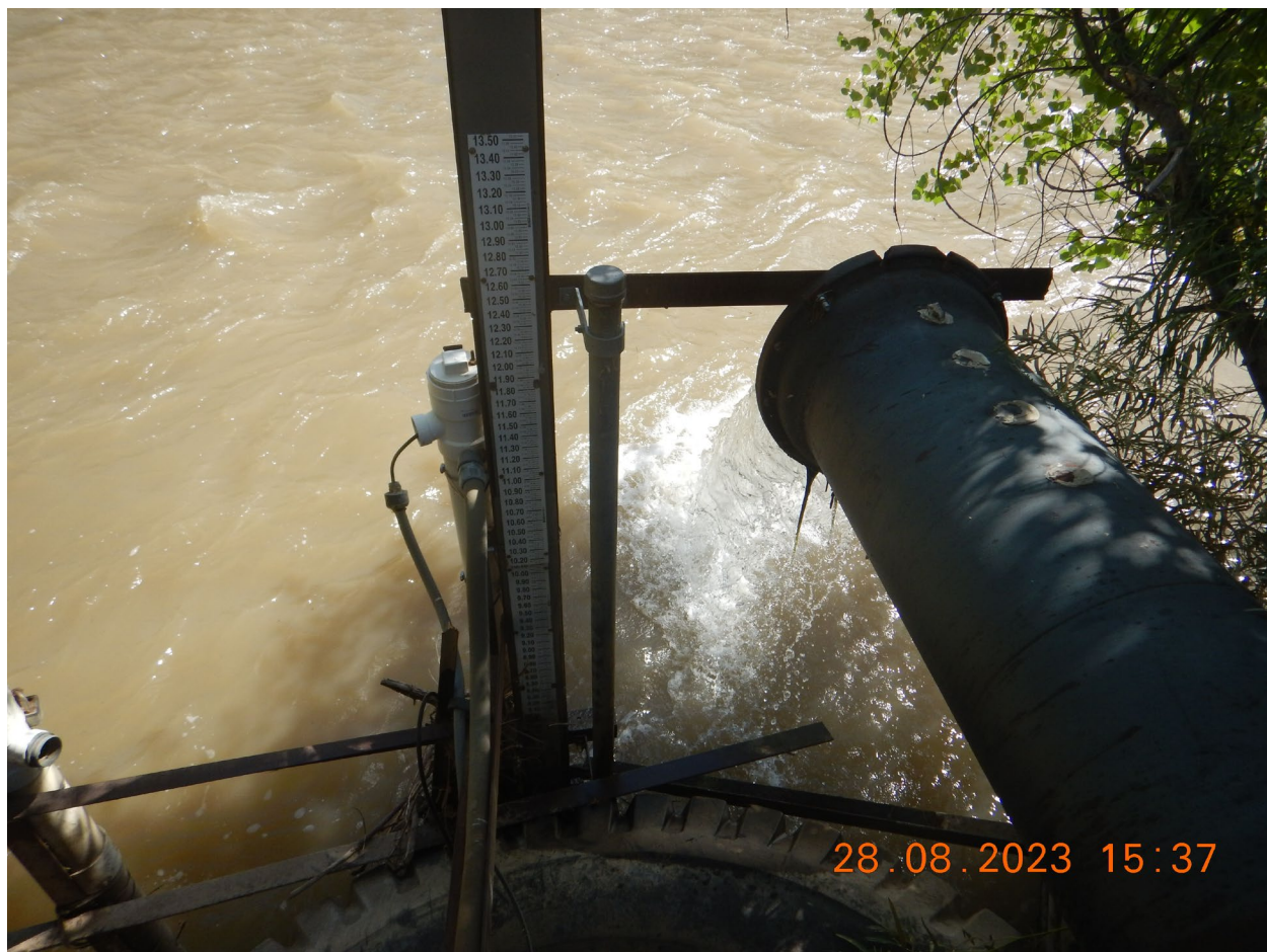
View of the WWTP outfall (discharge) of effluent into the Animas River. (DSCN2618). Photographed by D. Esparza
