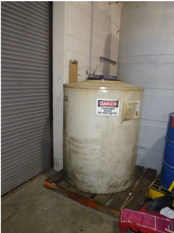
Photo 20: Used Oil Tank.
