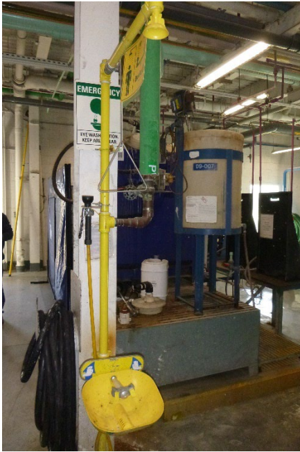
Photograph 89. WWTP CAA Decontamination Equipment
