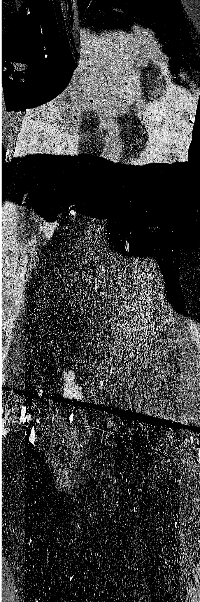
Oil Spill Staining on Pavement
