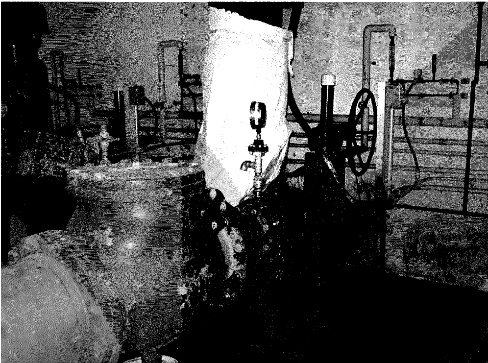
Photo 3 – Part of Emergency Generator, Catch Basin, and Shut-off Valve (far right of photo)
