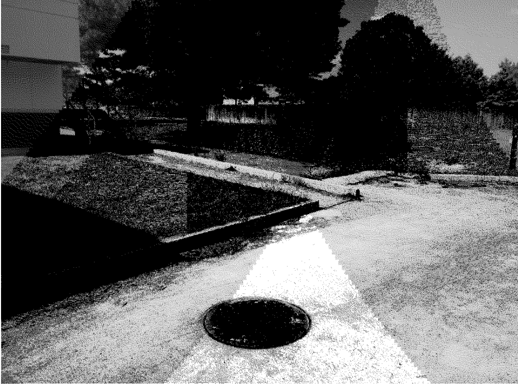
Photo 4 – One of Three Final Clarifiers
