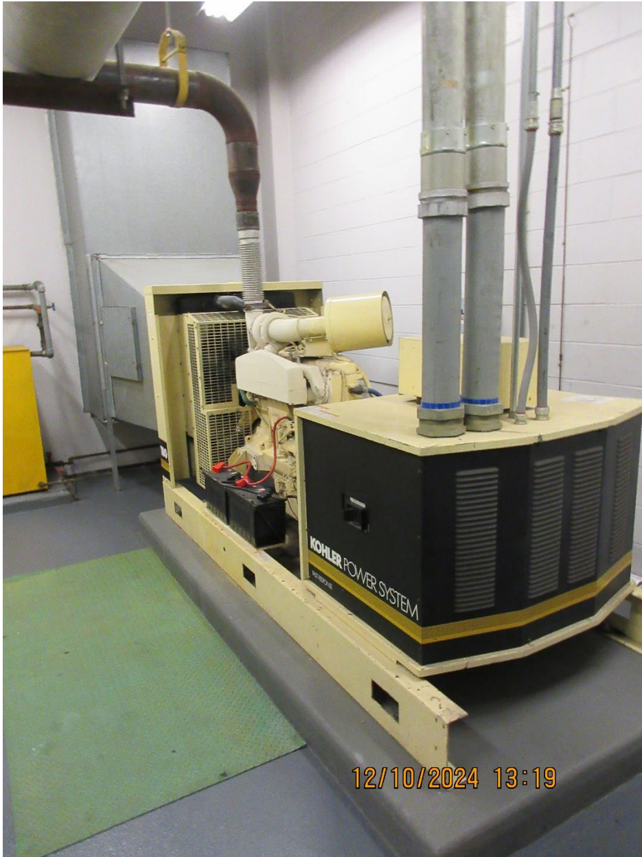
Photo 1 – Emergency Generator Room
