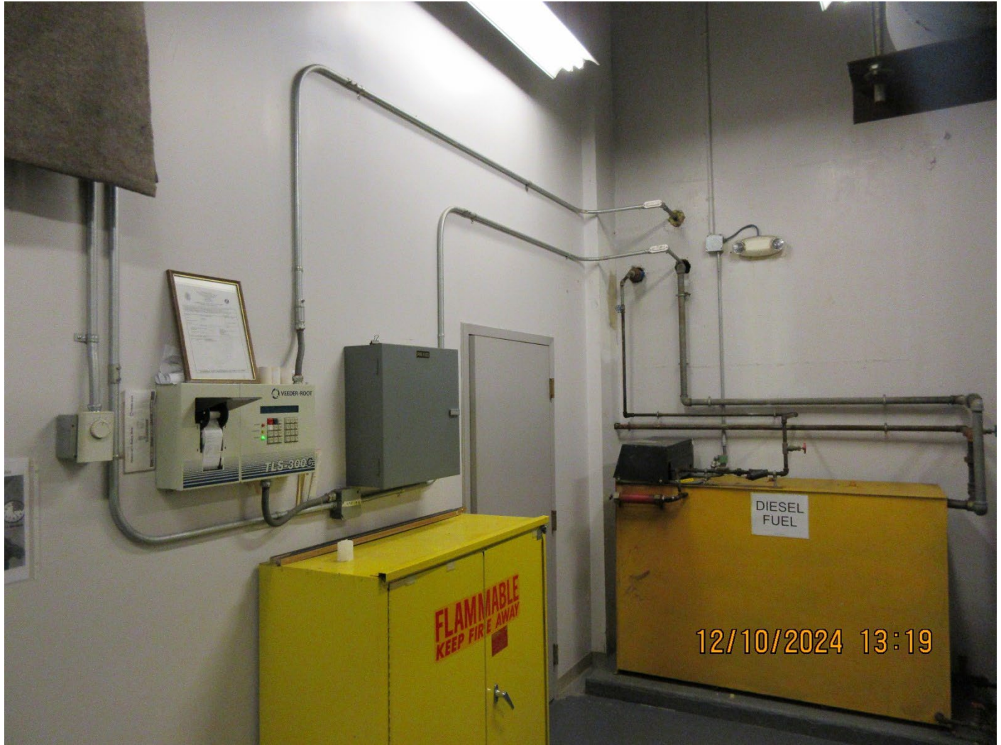
Photo 4 – Day tank (marked with "DIESEL FUEL" sign)
