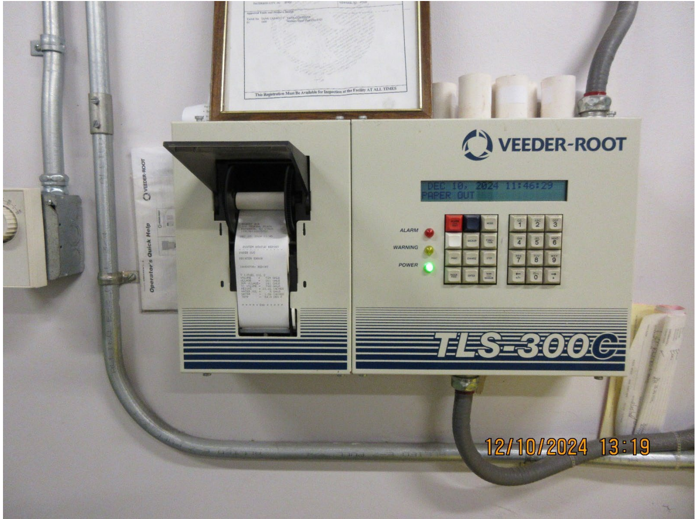
Photo 3 – Veeder Root TLS 300-C Automatic Tank Gauge (ATG)
