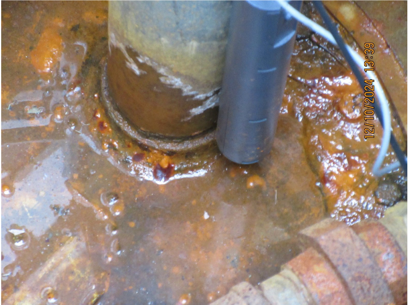
Photo 9 – Liquid sensor located 3+ inches from the bottom of the turbine sump.
