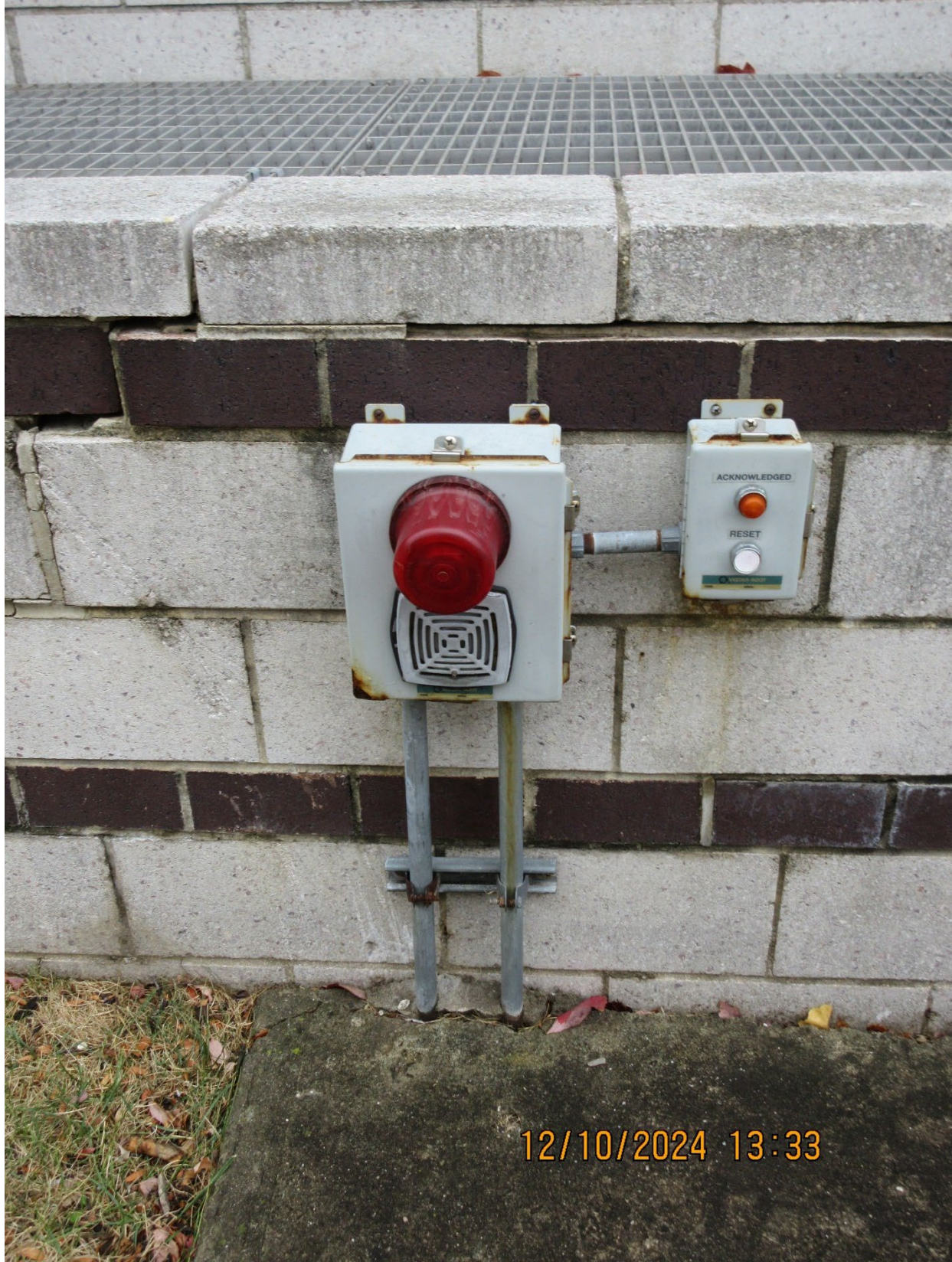
Photo 11 – High Level Alarm (HLA) seen from the front.
