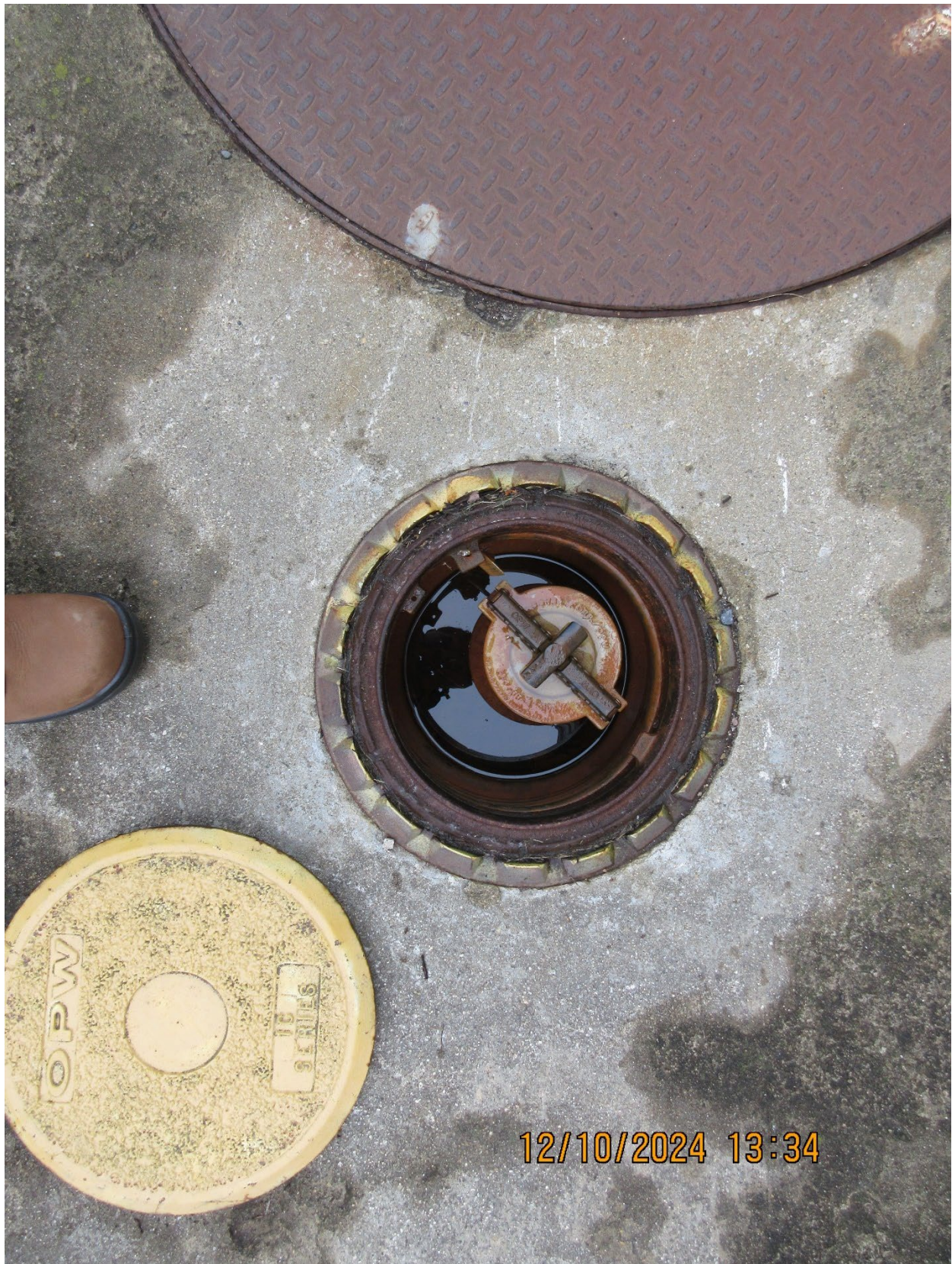
Photo 12 – Fuel port and spill bucket seen from above.
