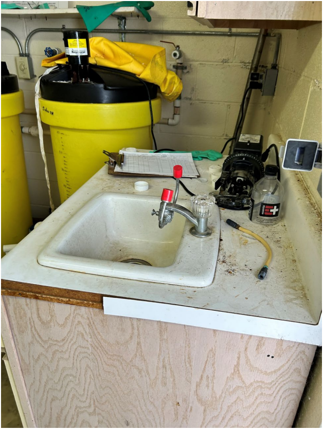
PH – Eye Wash device was not working correctly
