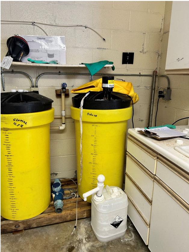
PH Piping – Soda Ash Tank Not in Use
