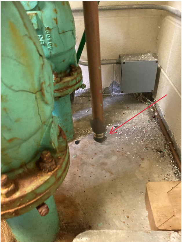
PH Piping – ARV w/ Screen
