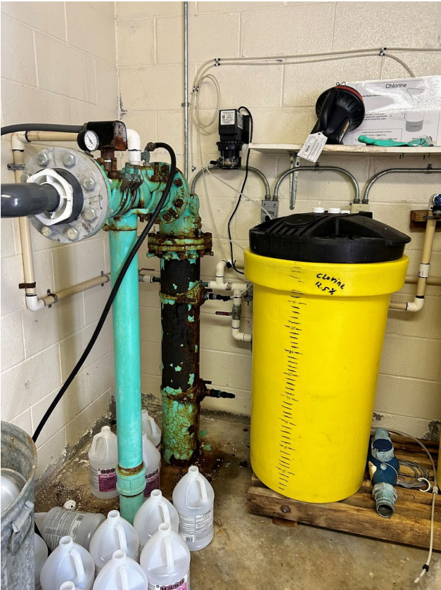
PH Piping – Chlorine Tank
