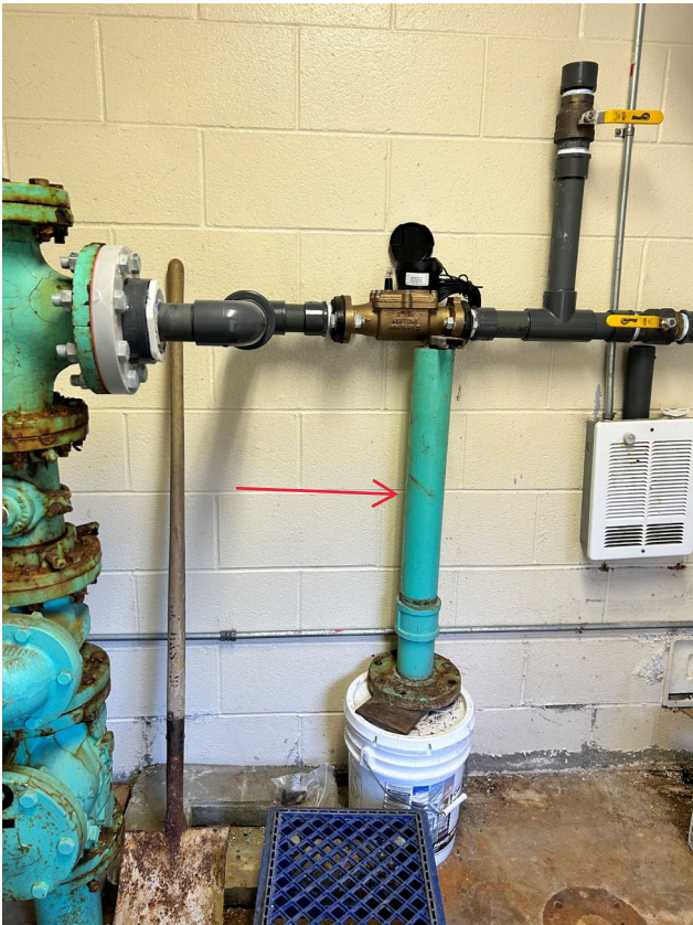
PH Piping – Need an appropriate support
