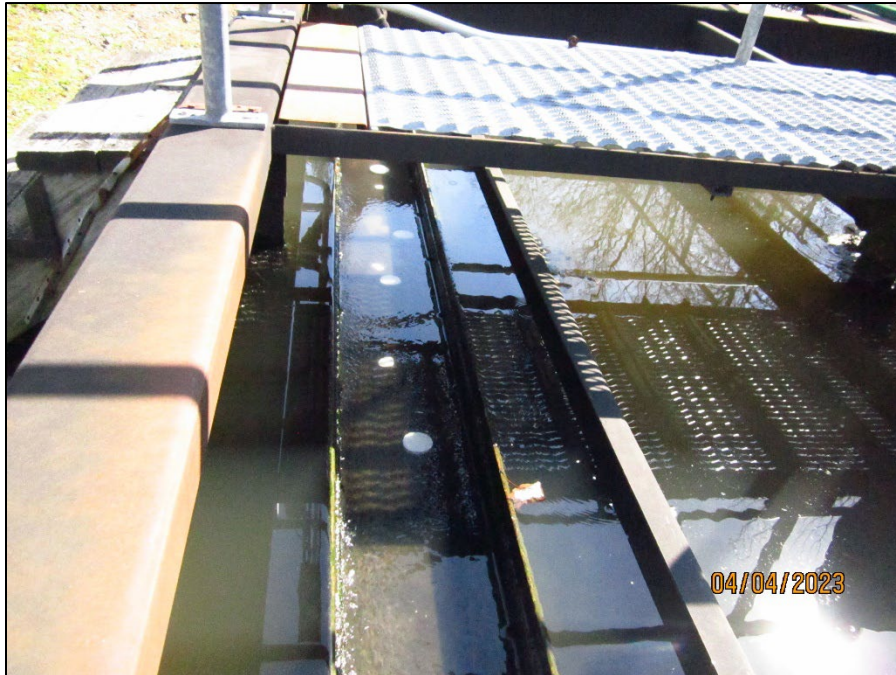
Photograph 14. IMG_0043.JPEG View of the effluent weir trough leading to the CCC. Note the multiple chlorine tablets at different stages of dissolving.
