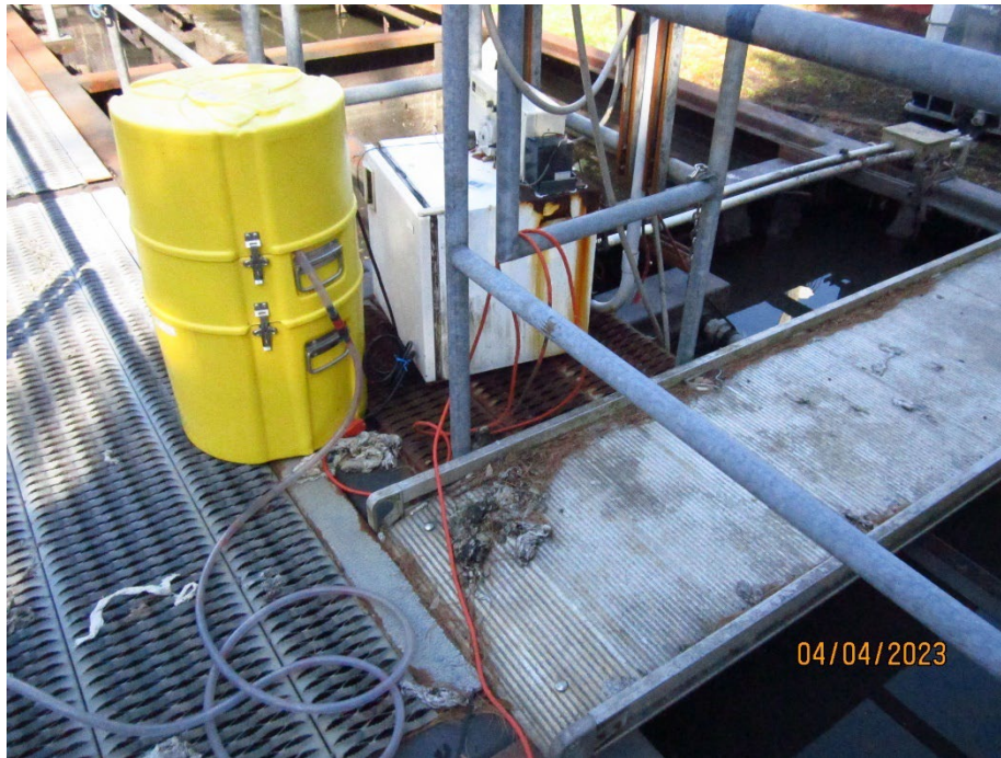
Photograph 3. IMG_0010.JPEG View of the current influent sampler and old influent sampler unit. There was miscellaneous tubing laying around the walkway and electrical cords hanging above the water. A scaffolding walkway was installed on the exterior of the safety railing; its use was unknown at the time of inspection.
