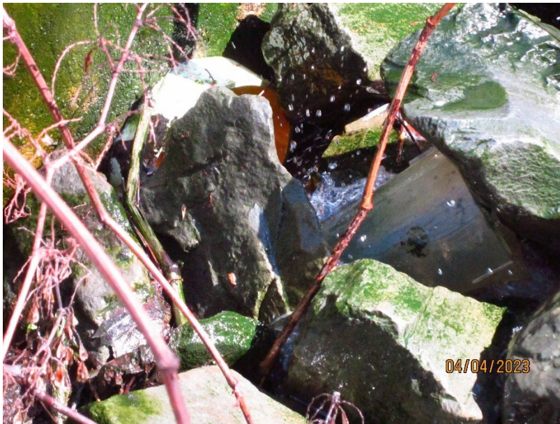
Photograph 20. IMG_0068.JPEG Close-up view of Outfall 001. Note the plastic debris lodged in the riprap.
