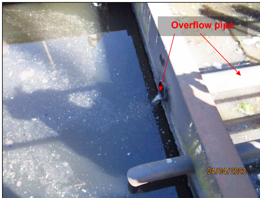
Photograph 5. IMG_0021.JPEG View of one of two gravity overflow lines (north side of the WWTP) from the EQ basin to the aeration basin.
