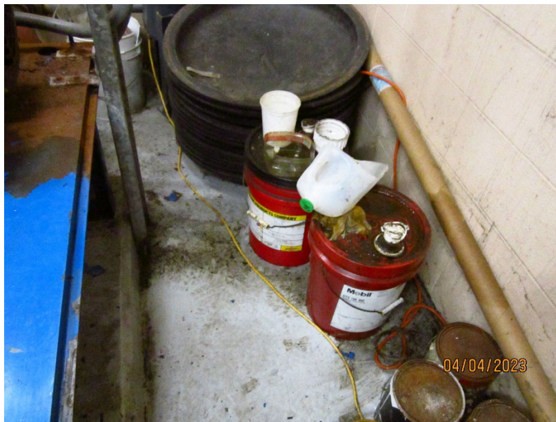
Photograph 21. IMG_0072.JPEG View of paint and oil stored in the blower room without secondary containment.
