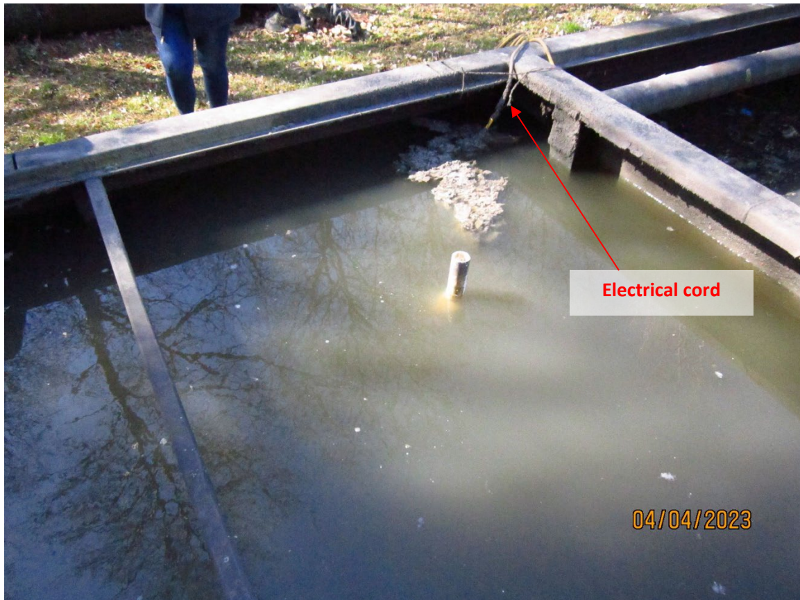
Photograph 2. IMG_0009.JPEG View of floating solids in EQ basin. Note the yellow electrical cord below the water level in the corner of the tank.
