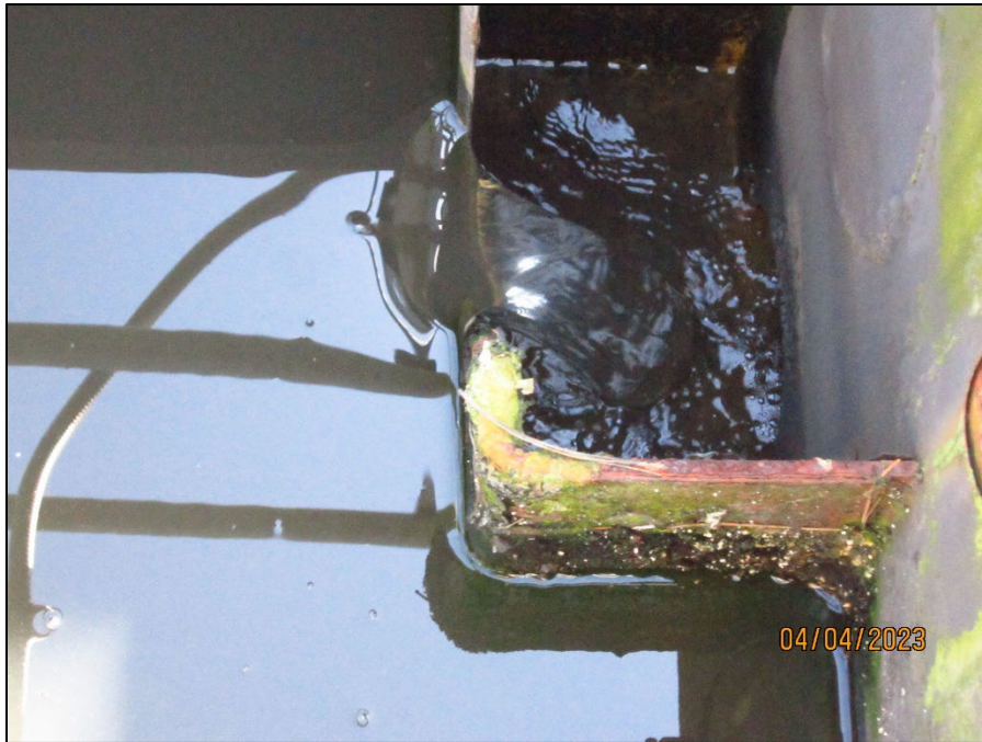
Photograph 17. IMG_0052.JPEG View of effluent weir leading to Outfall 001. Note there was no staff gauge (primary measuring device) for measuring the height of the water.
