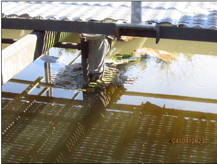
Photograph 15. IMG_0045.JPEG View of the bulking solids in the clarifier near the skimmer. Note how the debris is tightly packed and not breaking up easily. Also note the vegetation growth on the floating debris.
