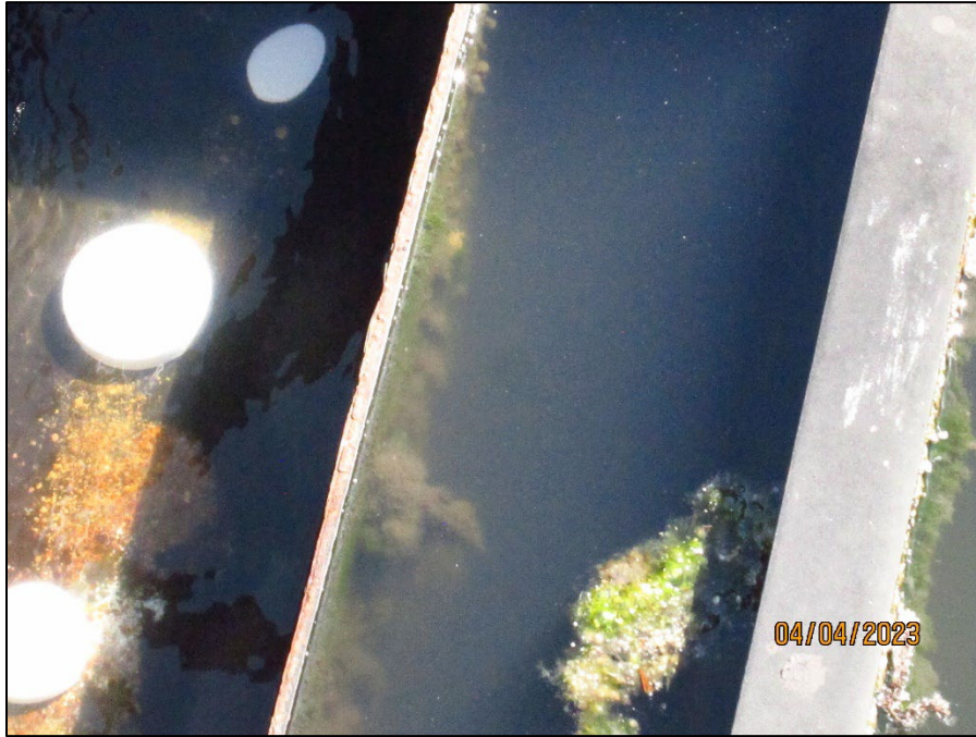
Photograph 13. IMG_0039.JPEG Close-up view of the weir trough and effluent baffle. Note the cloudiness observed in Photograph 12 is caused by pin floc. Floating debris with algal growth was also observed.
