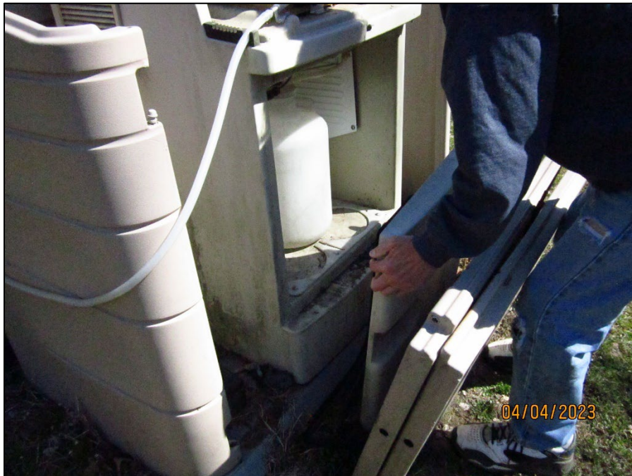
Photograph 18. IMG_0058.JPEG View of the Plant's effluent sampler. Note that the door to the refrigeration unit was no longer attached to the sampler and had fallen off. No thermometer was observed inside. The door was held in position by leaning plastic shed components.
