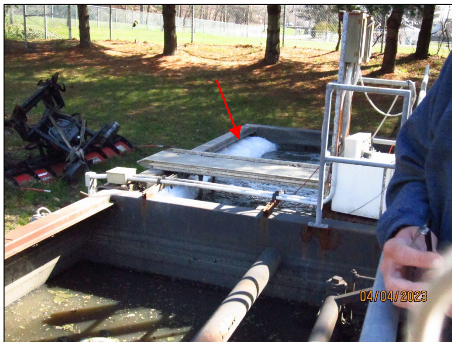
Photograph 8. IMG_0027.JPEG View of the EQ basin when the blowers were turned on. Note the heavy foam build-up.
