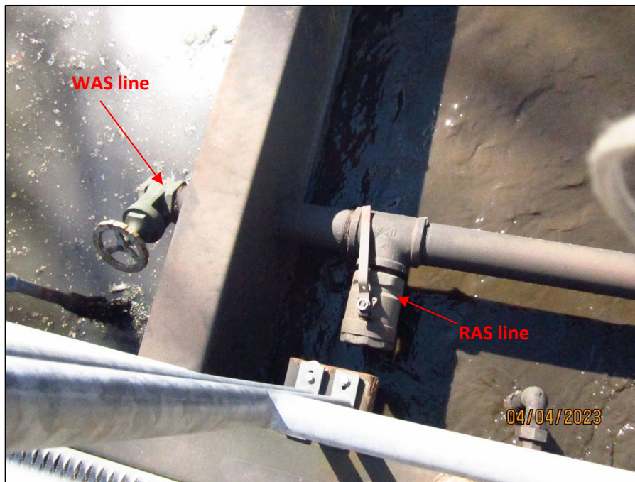
Photograph 7. IMG_0023.JPEG View of the RAS/WAS line discharge locations on the south side of the WWTP. The RAS valve was open, but there was not flow.
