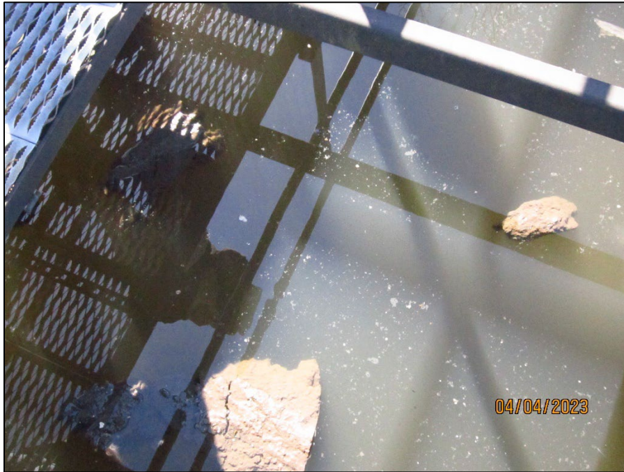
Photograph 11. IMG_0036.JPEG View of floating solids in clarifier.
