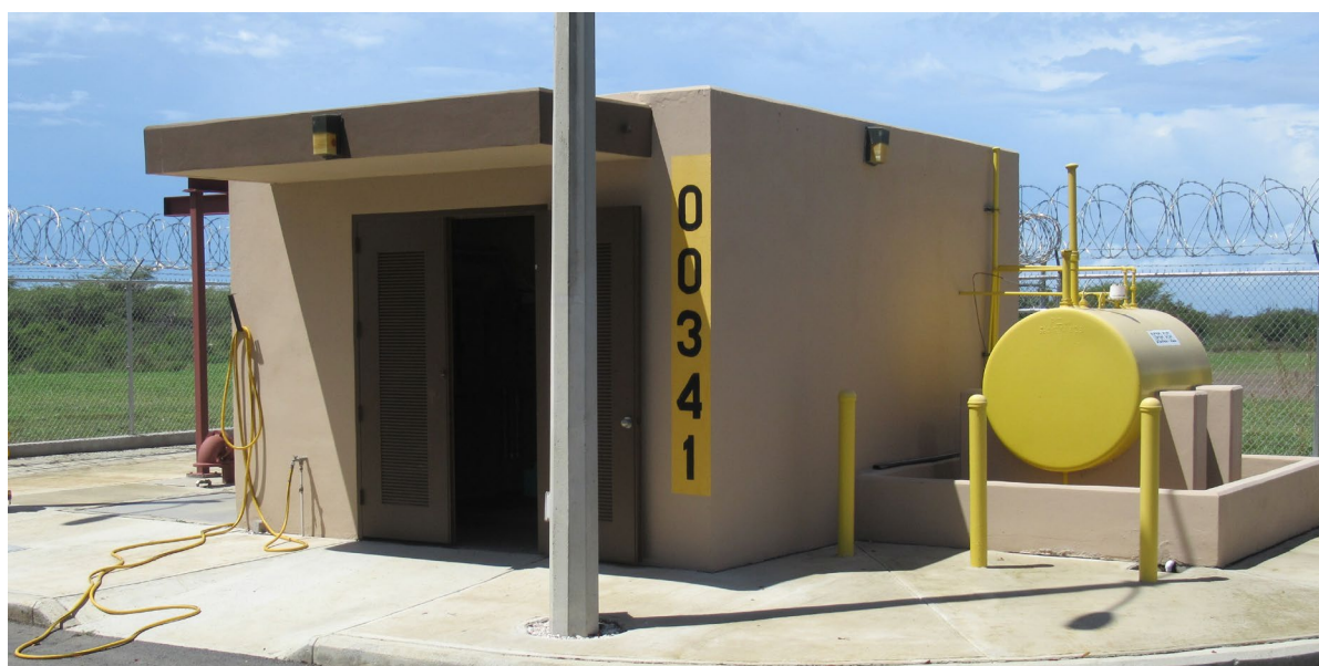
Photo 28 – Bldg. 00341; wastewater lift station
