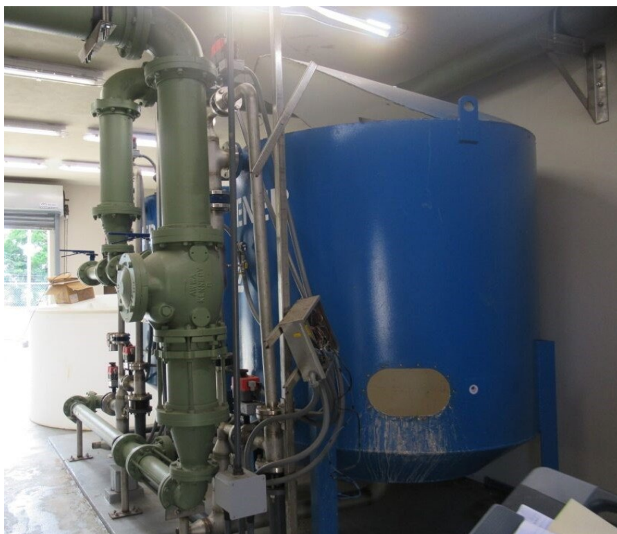
Photo 14 – Water softener tank 2; top of tank separated from its sides
