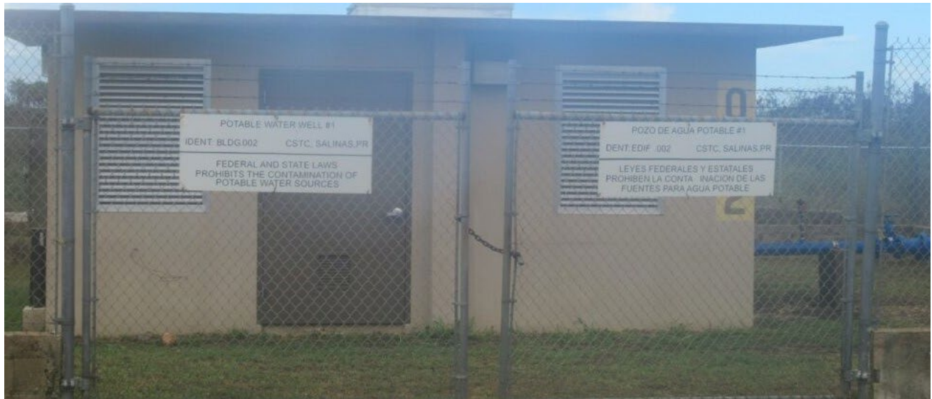
Photo 3 – Well No.1/Building (Bldg.) 002, secured enclosure and signage.
