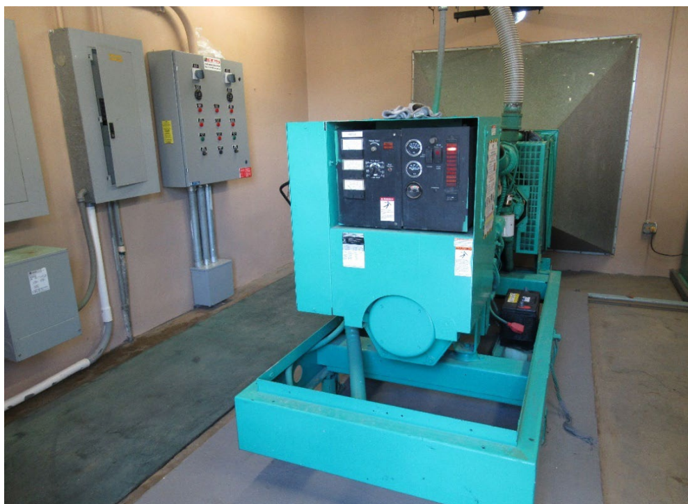
Photo 30 – Wastewater lift station diesel-fueled power generator
