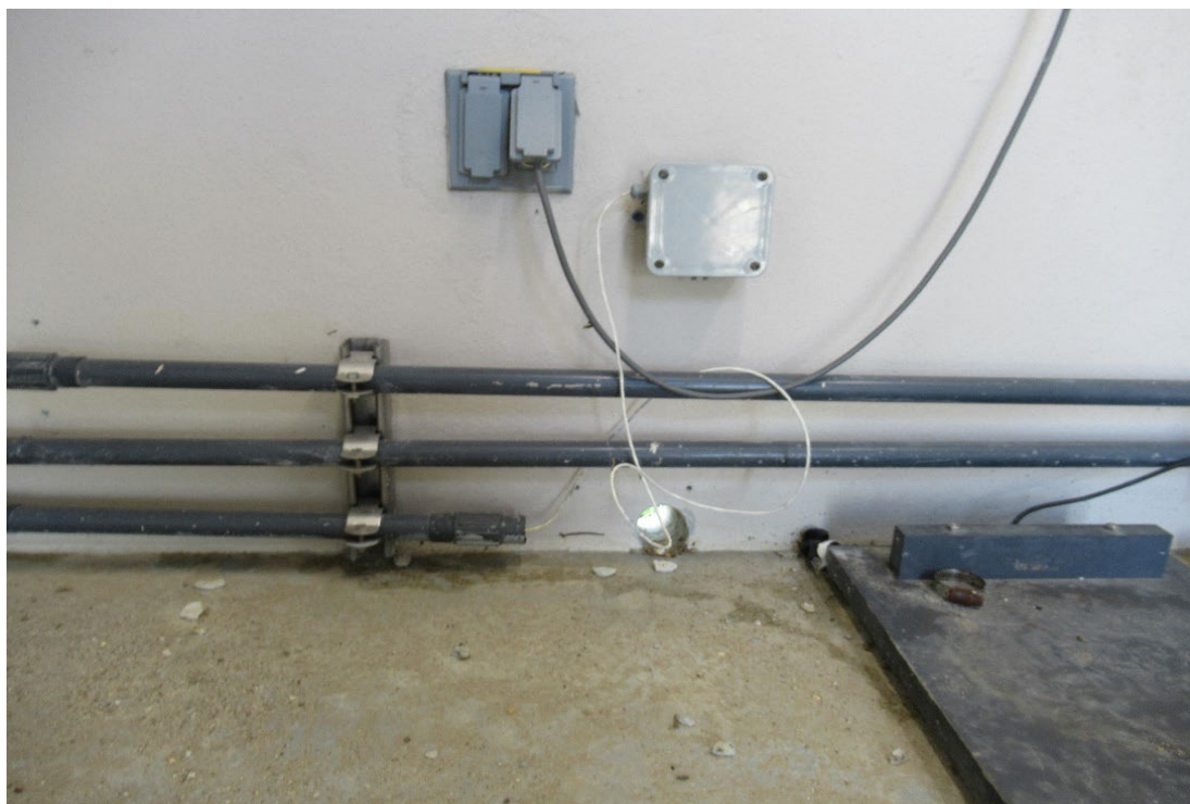
Photo 21 - Chlorine room; unscreened wall opening with unprotected wiring (2 of 2)
