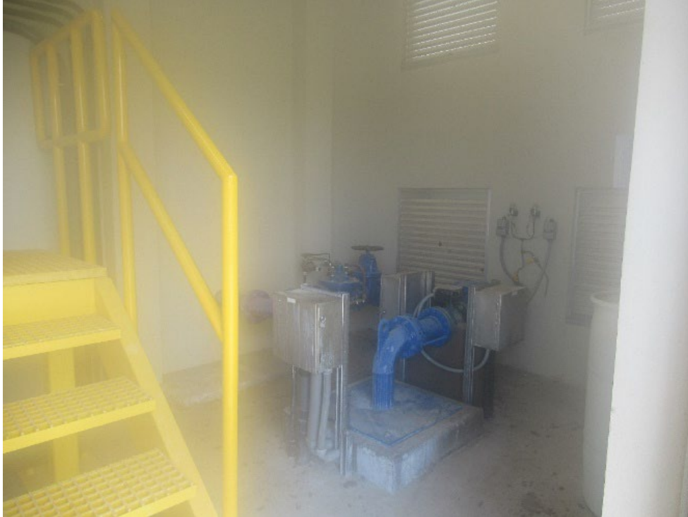
Photo 9 – Bldg. 003; interior, Well No.2 wellhead
