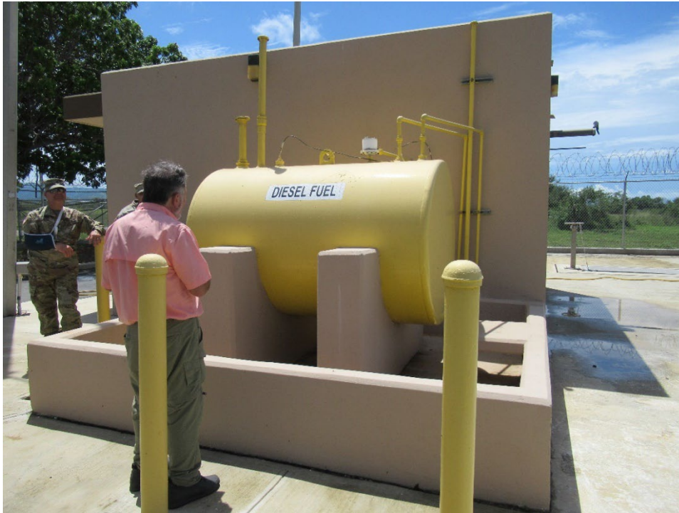
Photo 31- Bldg.00341; 550-gallon above ground diesel fuel storage tank
