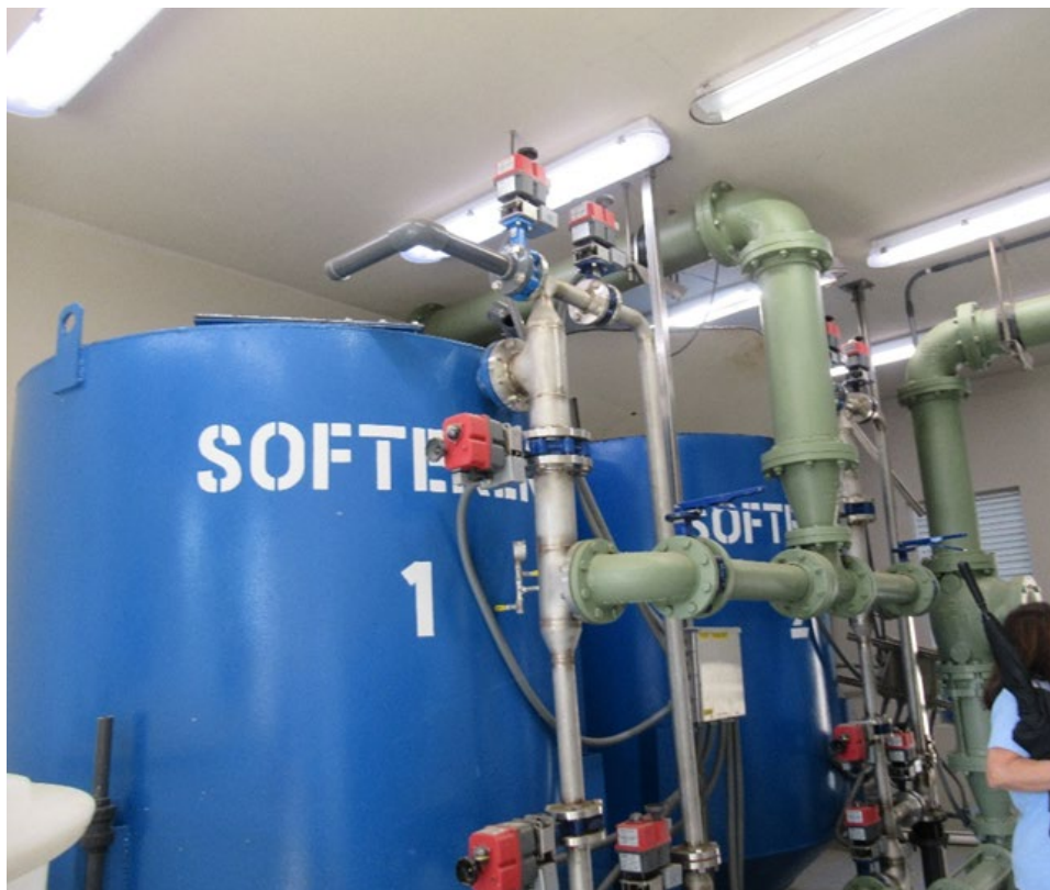
Photo 13 – Treatment & Chlorine Room; water softener tanks 1&2
