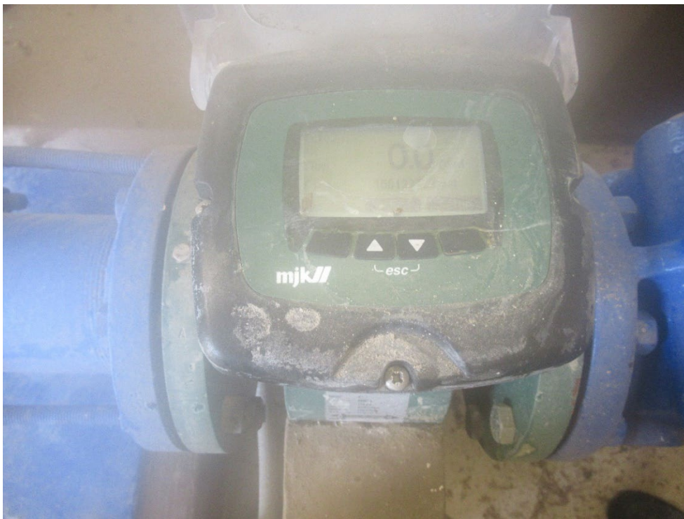
Photo 10 – Bldg. 003; Well No.2 flow meter
