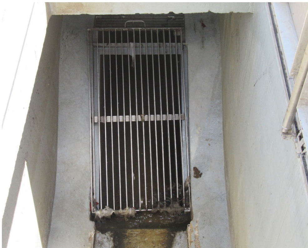
Photo 29 – Bldg. 00341; wastewater inlet screen
