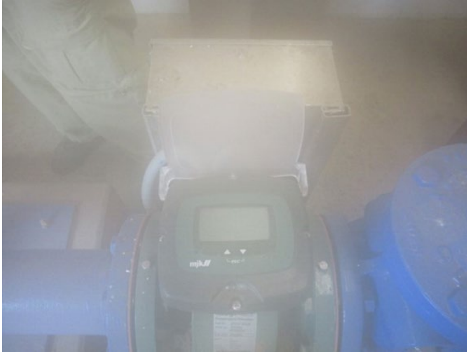
Photo 5-Well No.1 flow meter (non-functional)
