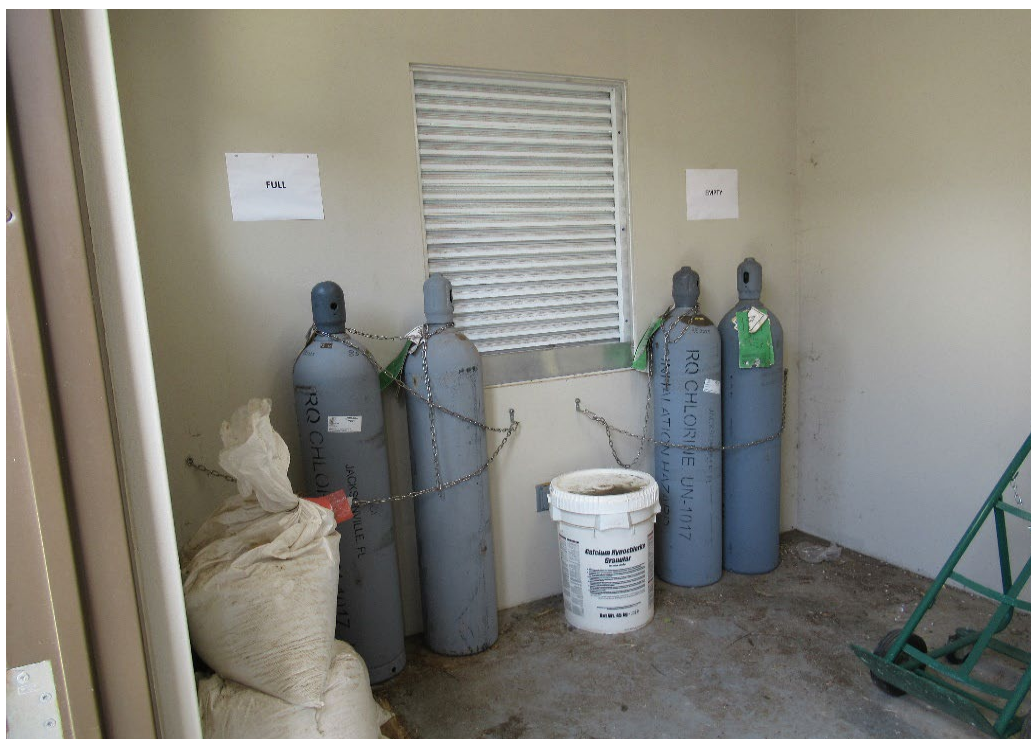
Photo 24 – Chlorine gas cylinders (full & empty), granular calcium hypochlorite
