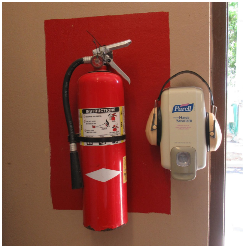
Photo 33- Bldg. 00341; fire extinguisher without inspection tag
