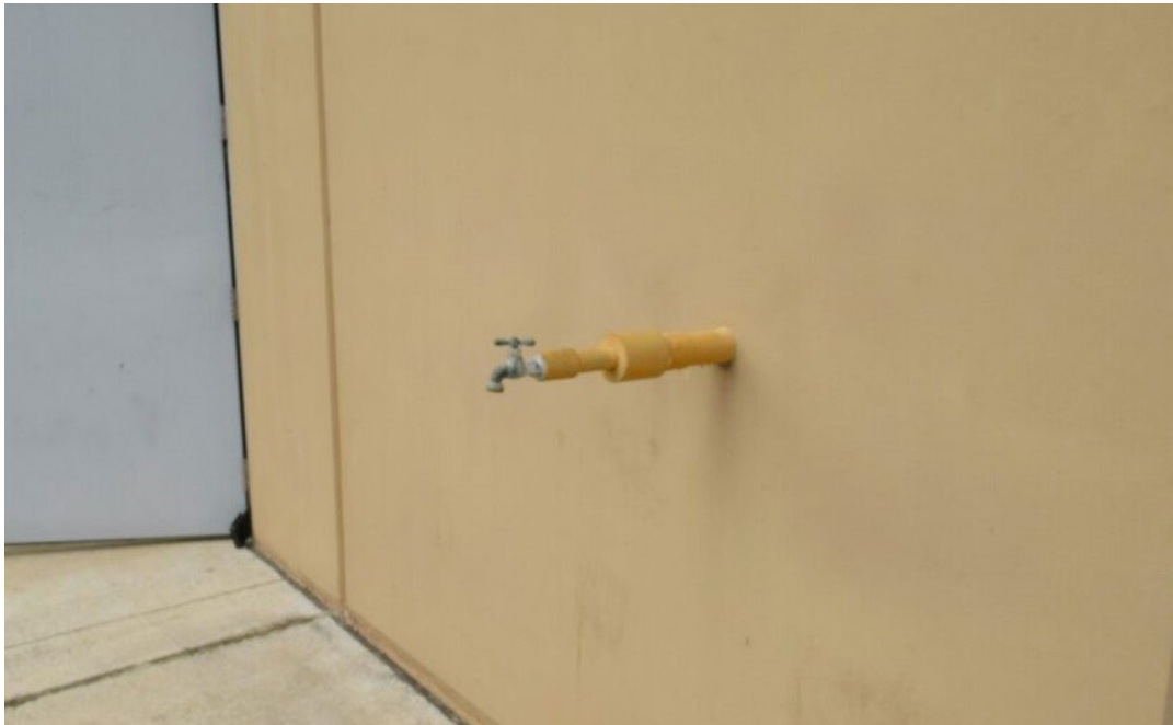
Photo 38 – Area of Bldg. 1011; threaded outdoor faucet
