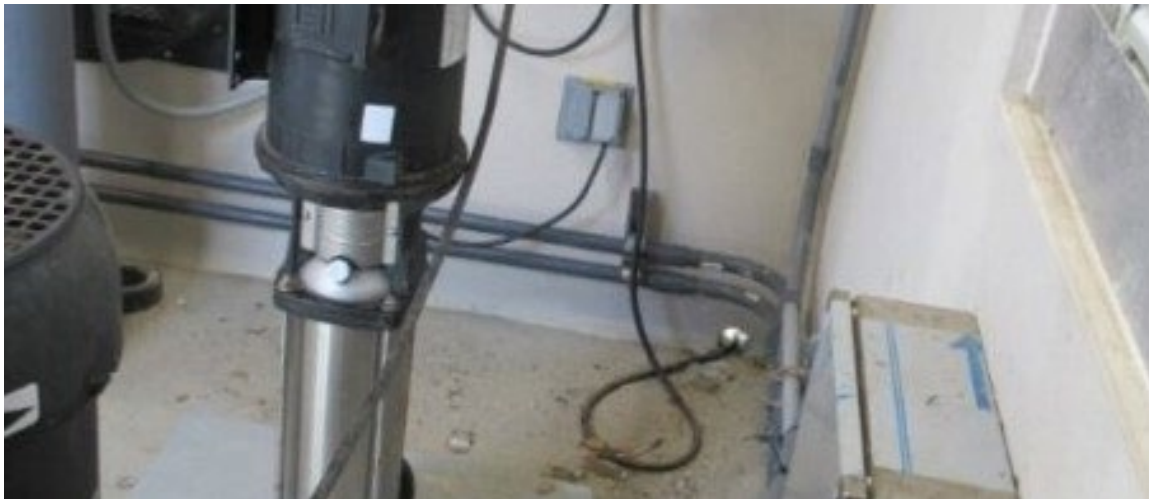
Photo 20 – Chlorine room; unscreened wall opening with unprotected wiring (1 of 2)
