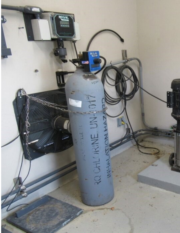
Photo 19 – Chlorine bldg. exhaust fan, chlorine gas tank and scale (1 of 2)
