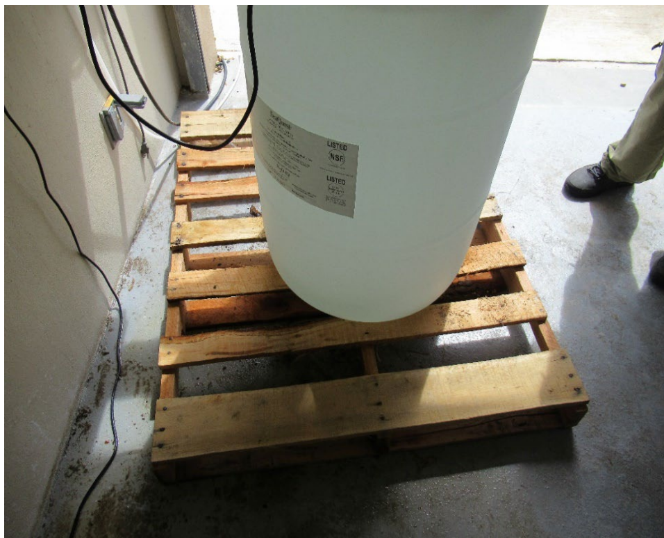
Photo 17 – Treatment & Chlorine Room; 55-gallon drum of phosphate chemical on wooden pallet
