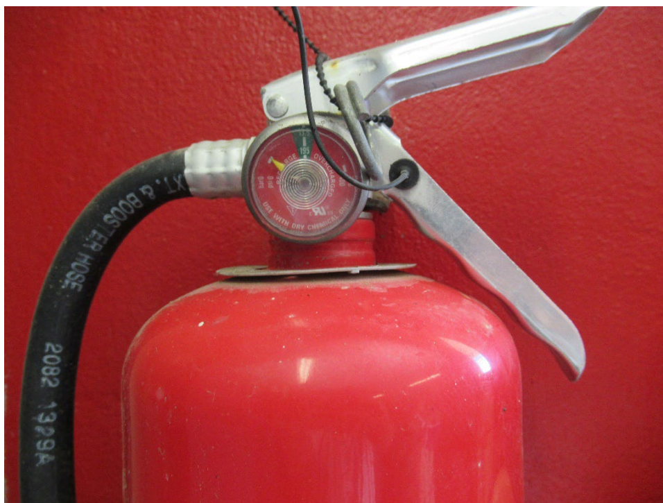
Photo 34 – Bldg. 00341; depressurized fire extinguisher
