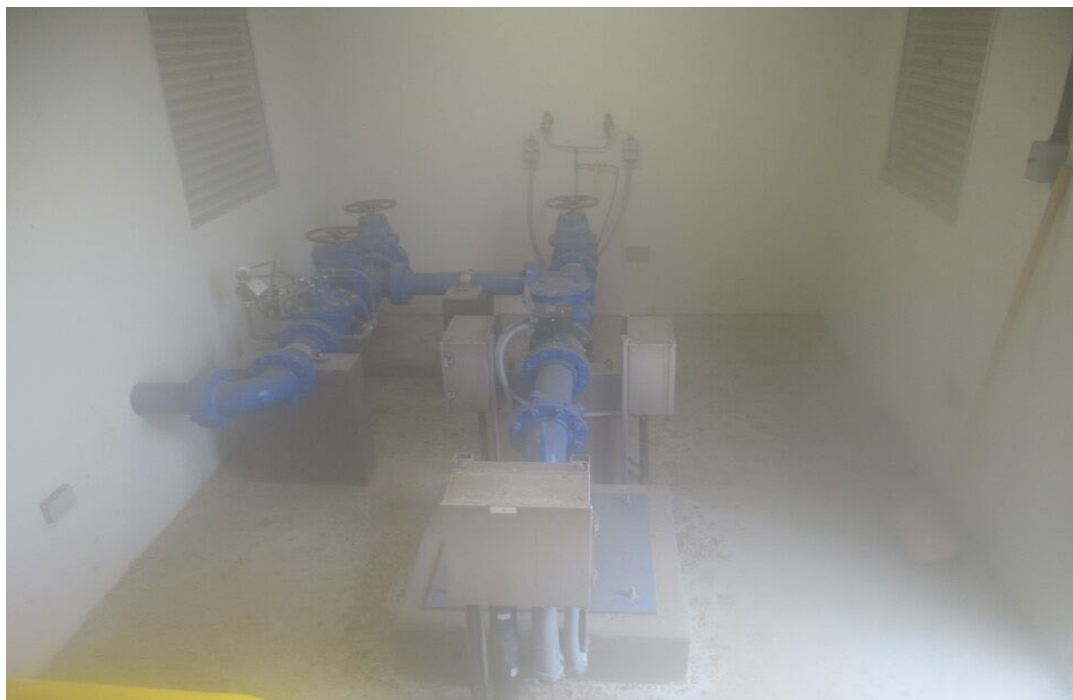
Photo 4 –Bldg.002; Well No. 1 well head
