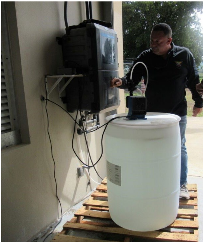
Photo 16 – Phosphate chemical (55gallon drum), chemical analyzer and feed pump
