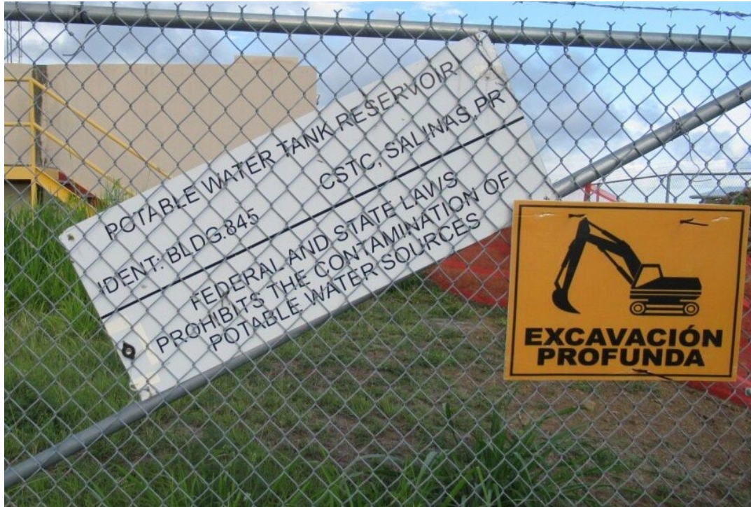
Photo 39 – Bldg. 845; potable water storage tank secured enclosure and signage
