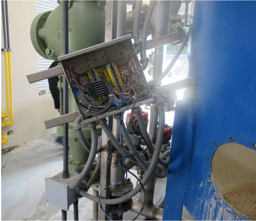
Photo 15 – Water softener tank 2 electrical hub
