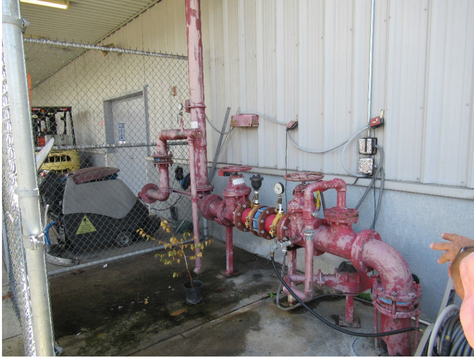
Photo 35- PX bldg.; fire suppression water supply and check valves
