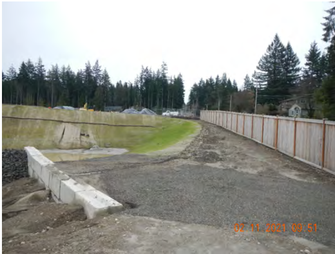
Photo #:19 (DSCN2045) Description: Facing east, photo of the unstabilized area along the southern fencing line. Photo taken on 02/11/21.
