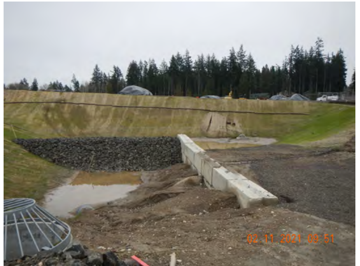
Photo #:20 (DSC2046) Description: Facing east, photo of the unstabilized area along the southern perimeter fence line. Channelized erosion was observed in the direction of a stormwater detention pond. Photo taken on 02/11/21.
