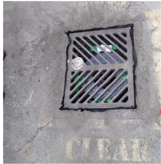
Photo #:22 Description: Facing north, photo of a witches hat in the inlet of the catch basin.
