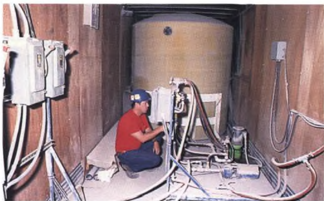
Foaming agent is stored in 2,000-gal. polypropylene tanks anchored to the floor in the trailer's end section.
