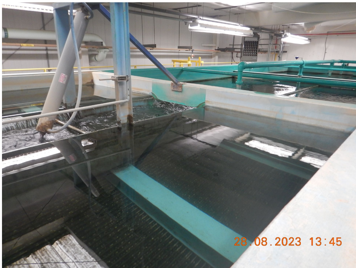
View of a portion of the treatment processes of Plant #3 and #4. (DSCN2612). Photographed by D. Esparza
