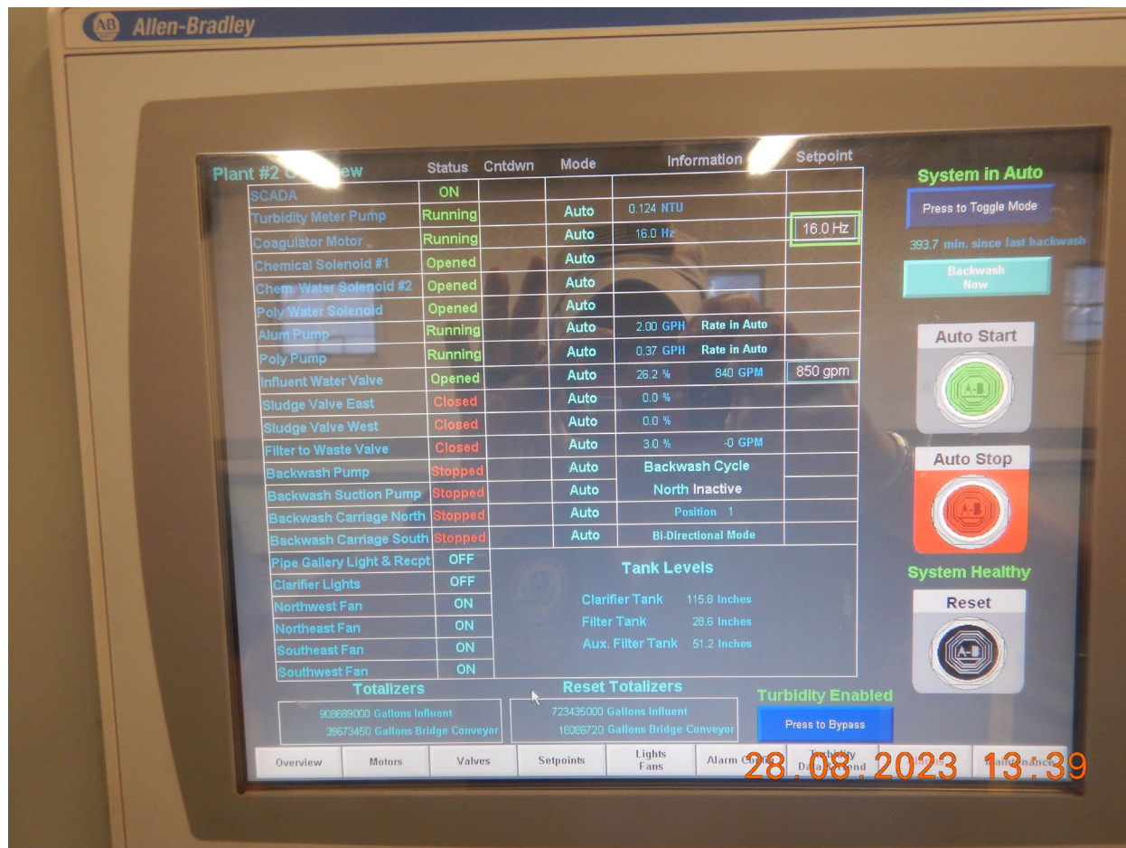
View of Plant #2 Supervisory Control and Data Acquisition (SCADA) data display. (DSCN2609). Photographed by D. Esparza
