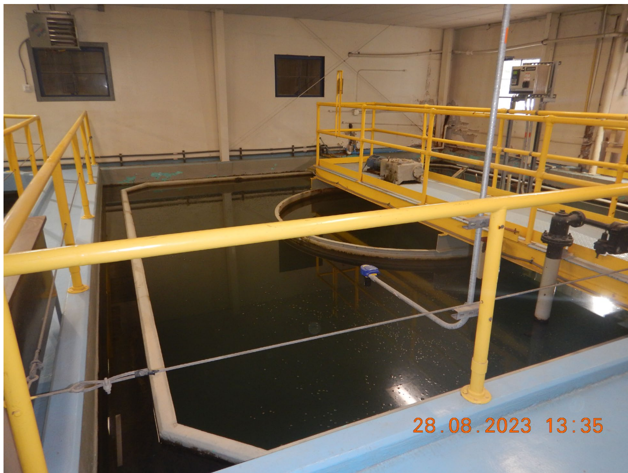
View looking towards Plant #2 clarifier. (DSCN2606). Photographed by D. Esparza
