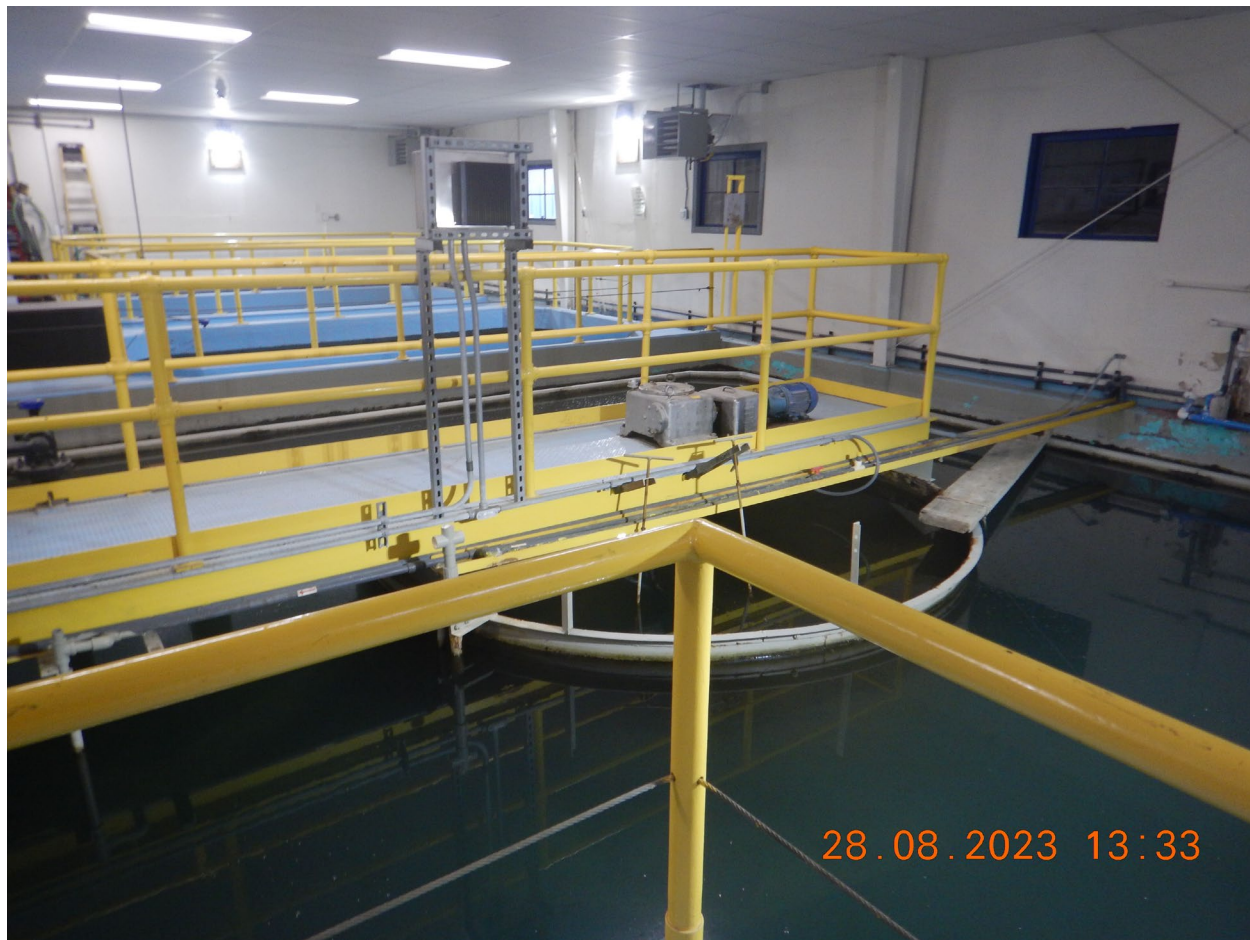
View of the Plant #1 clarifier and filters #1 and #2. (DSCN2605). Photographed by D. Esparza
