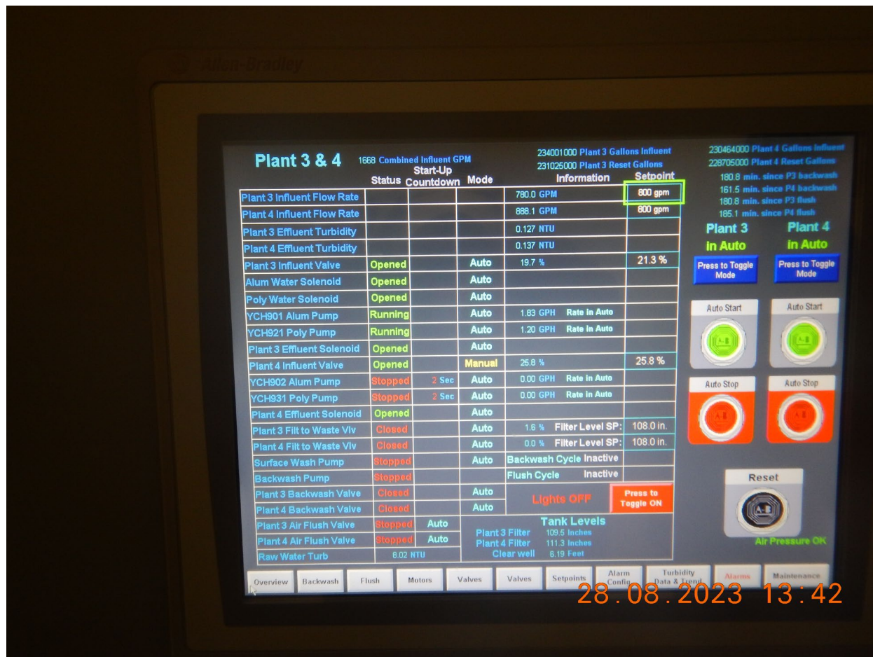
View of Plants #3 and #4 Supervisory Control and Data Acquisition (SCADA) data display. (DSCN2611). Photographed by D. Esparza
