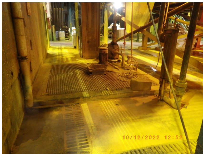
11: APOL0320 Description: Yellow pigment process floor pit Location: Northeast side of Building 2 Camera Direction: Southeast Date/Time: 10/12/22, 12:52 p.m.
