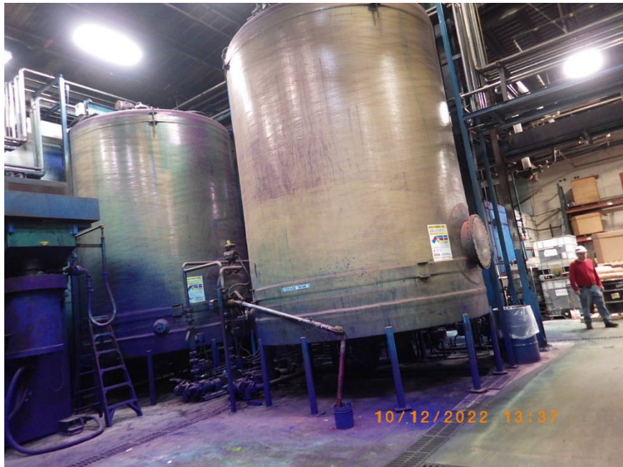
37: APOL0346 Description: Blue pigment storage tanks Location: Blue Room, south corner of Building 1 Camera Direction: North Date/Time: 10/12/22, 1:37 p.m.
