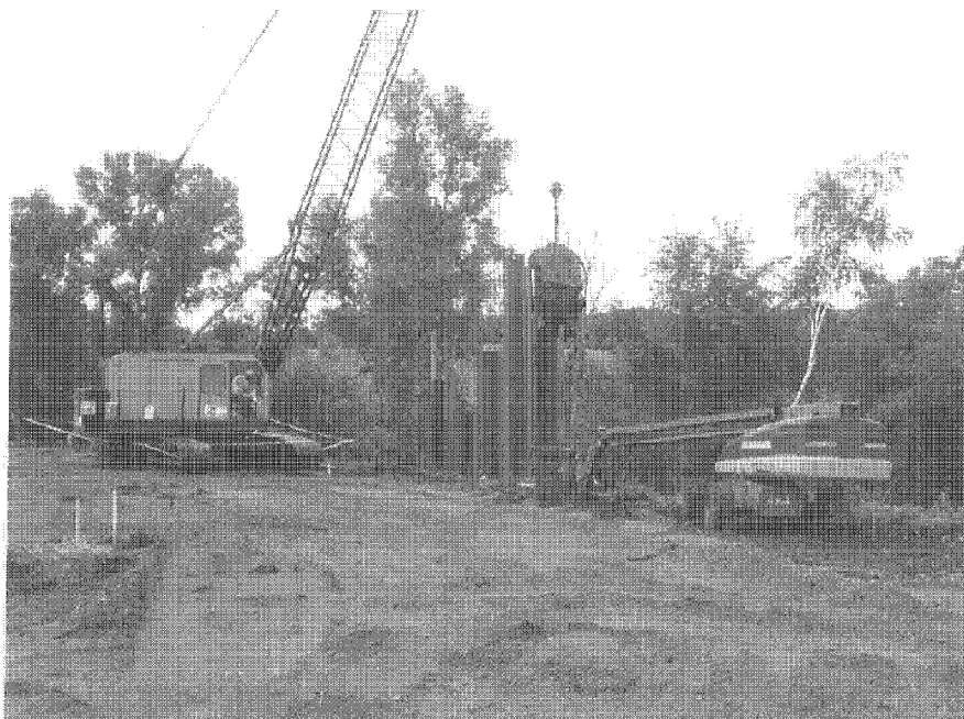
• Photograph 4: D9 Area – Sheet Piling Early Refusal along East End of Wall Due to C&D Waste along Slope (6/2/2010).
