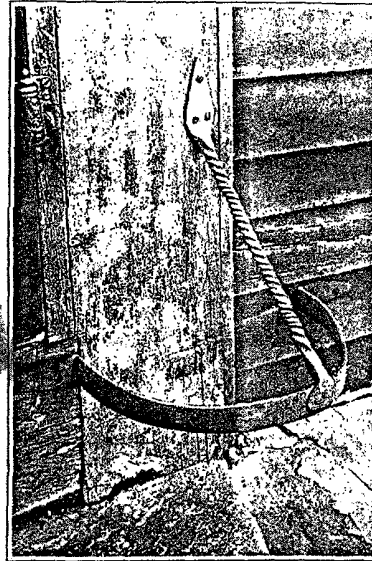
Illustration of painted surface in complete disintegration. The surface was allowed to remain too long before repainting was done, and it was no longer in a receptive condition to assimilate more paint.
