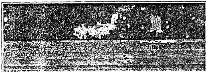
A rather extreme case of cracking. When this condition exists it is necessary to remove the paint either by scraping or by burning and scraping combined.
