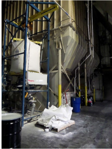
Photo-7 Metal Melt Baghouse Facility, Magox spill
