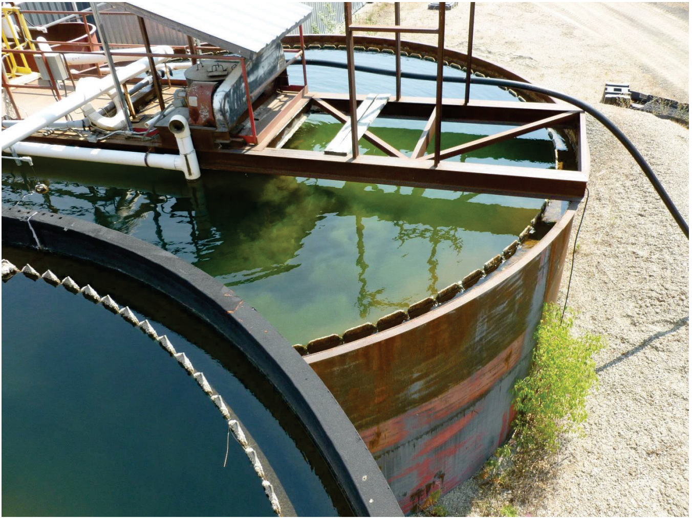
Photo 6 / P1010009 – Wastewater Plant Clarifier
