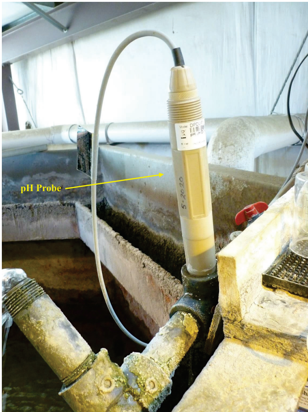
Photo 10 / P1010003 – Effluent pH Monitoring Probe
