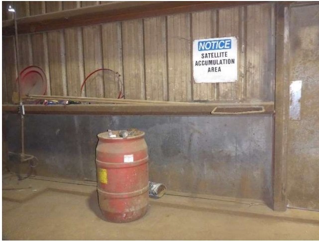
Photo 27: EAF Baghouse - Loadout Building - Contaminated PPE container
