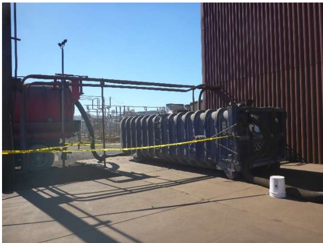
Photo 12: East of EAF Baghouse – Vac box, vacuum hose, and contractor truck
