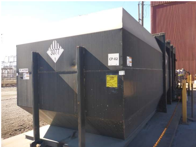
Photo 14: East of EAF Baghouse – Compactor
