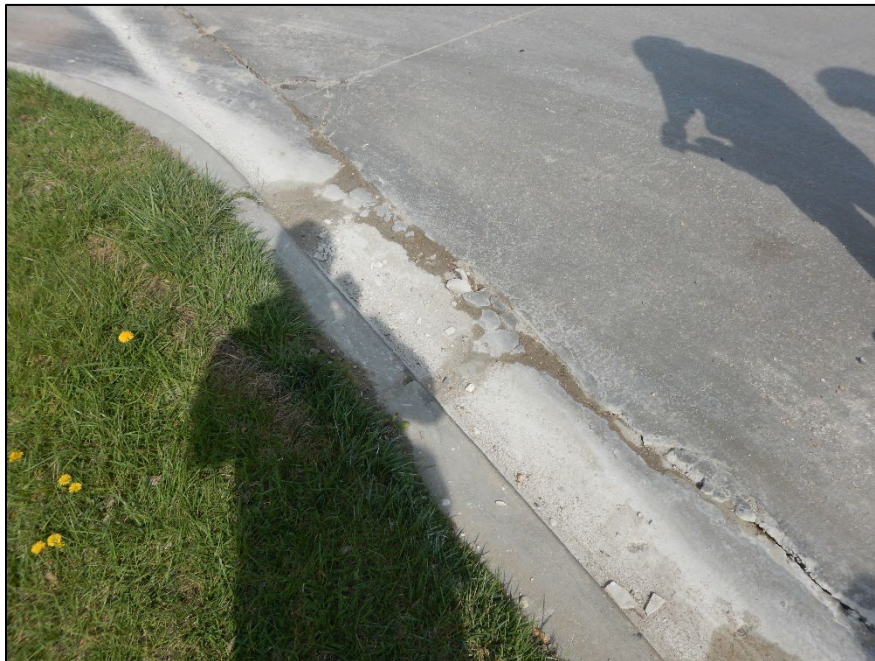
Photograph 16. DSCN8786.JPEG View downgradient of Outfall 001. Note the white drywall debris in the curblin.
