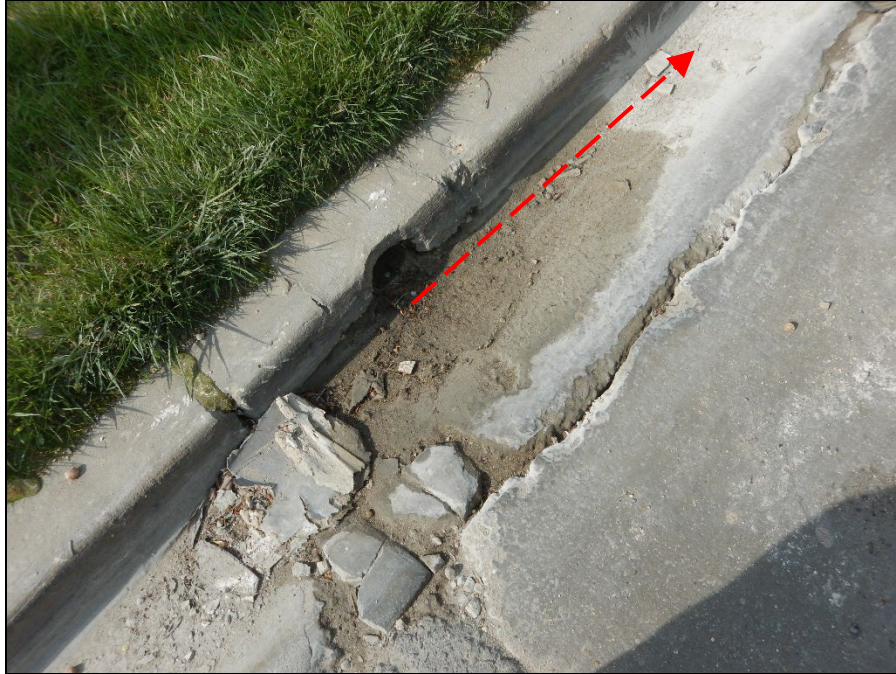
Photograph 15. DSCN8785.JPEG View of Outfall 001 in the Chrysler Drive curblin. The outfall was not discharging at the time of the inspection. Note the white drywall debris in the vicinity.
