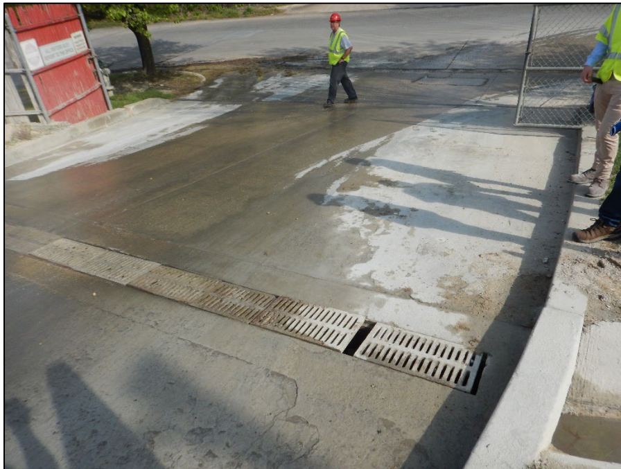
Photograph 18. DSCN8770.JPEG View of the wash area trench drain near the north gate with product and sediment track-out downgradient of the drain.
