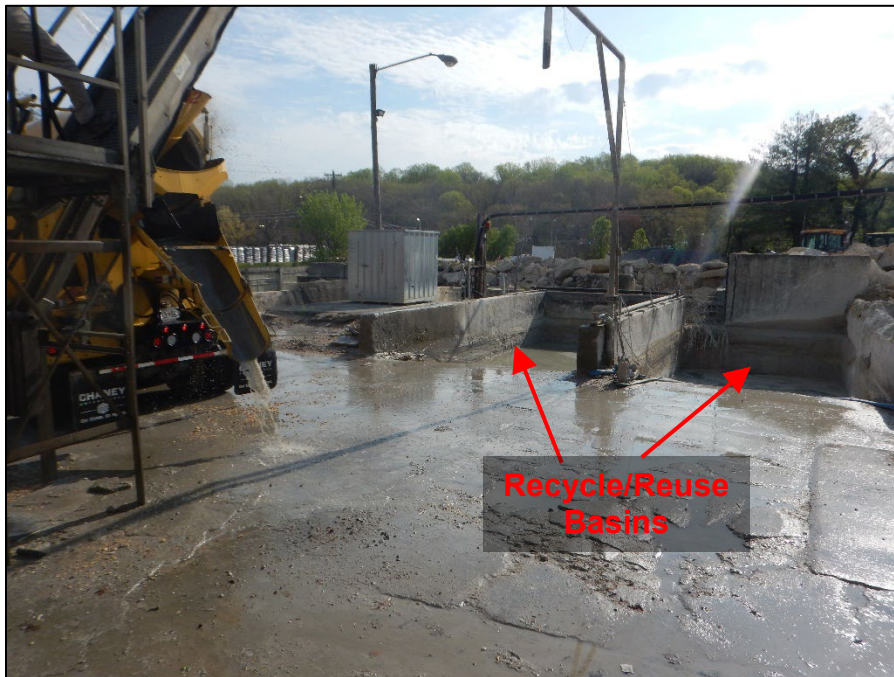
Photograph 4. DSCN6738.JPEG View of two recycle/reuse basins located in the center of the Facility.
