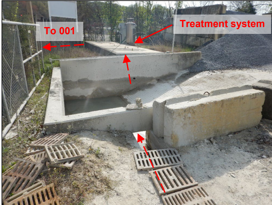
Photograph 13. DSCN8780.JPEG View, facing east, of the sediment basin ahead of the treatment system for Outfall 001. The basin overflows into the treatment system when full. The treatment system was in standby and not discharging at the time of the inspection.
