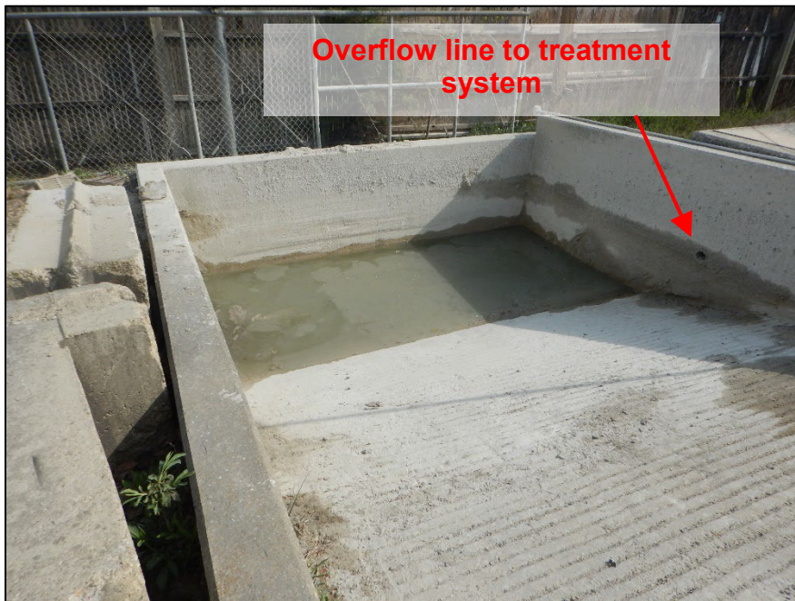
Photograph 14. DSCN8781.JPEG View of the sediment basin upstream of the treatment system connected to Outfall 001. Note the location of the overflow line.
