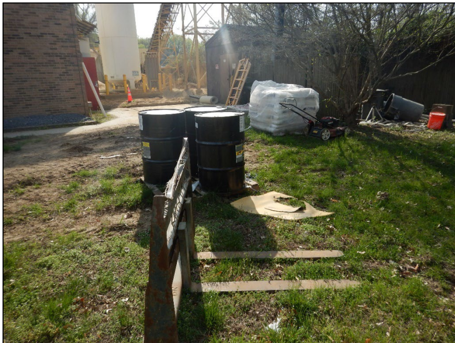
Photograph 22. DSCN8748.JPEG View of chemical drums and other material stored uncovered outside the office/batch plant building.
