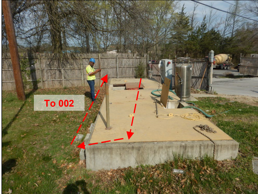
Photograph 7. DSCN8749.JPEG View of the treatment system connected to Outfall 002.
