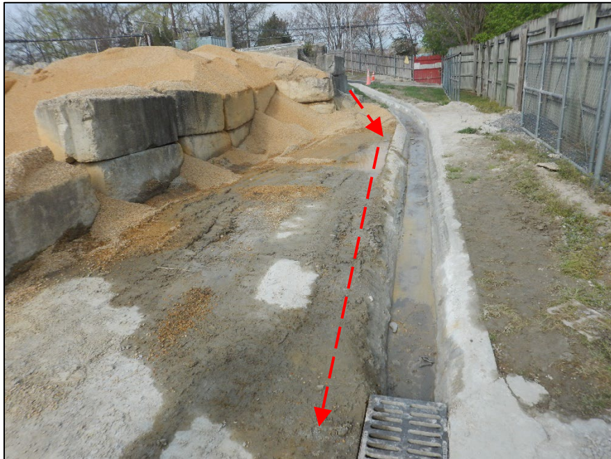
Photograph 12. DSCN8778.JPEG View, facing west, of the conveyance channel that feeds the sediment basin ahead of the Outfall 001 treatment system. Note the stockpiles were beyond containment and material and debris had migrated into and directly adjacent to the channel.
