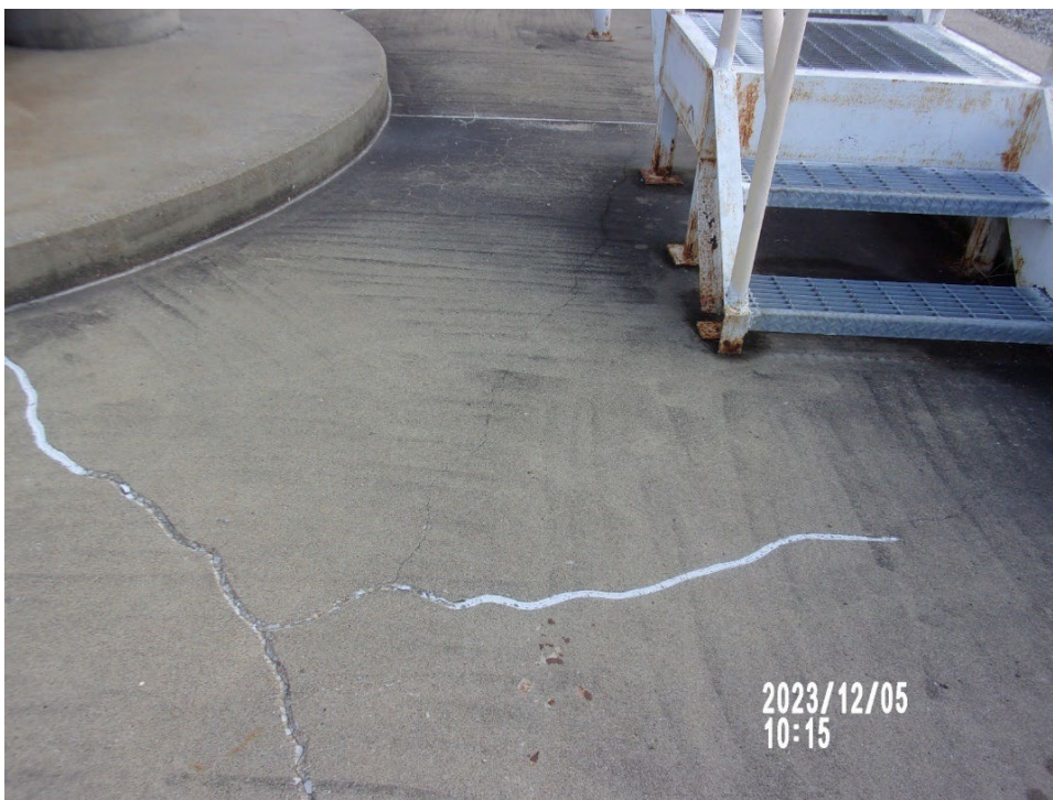
Photo 6: Cracks near the hazardous waste accumulation tank.
