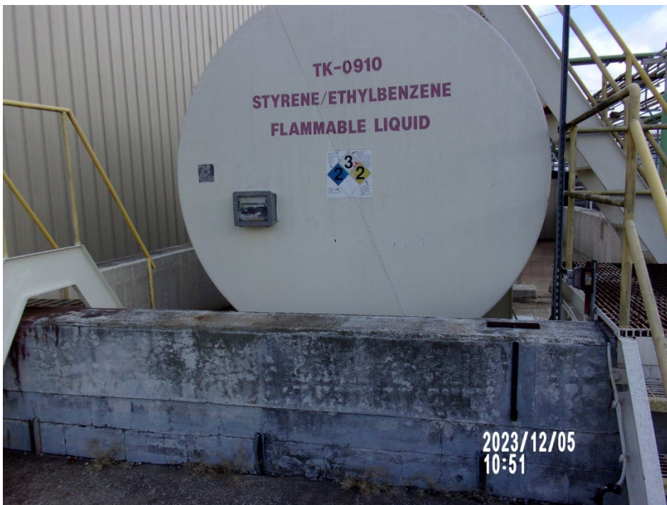
Photo 20: Former 90-Day Hazardous Waste Accumulation Tank Converted to a Product Tank.
