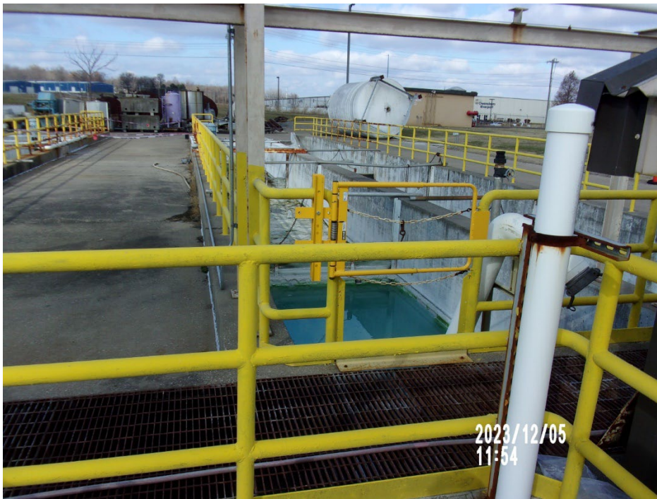
Photo 37: Wastewater Treatment Tanks.
