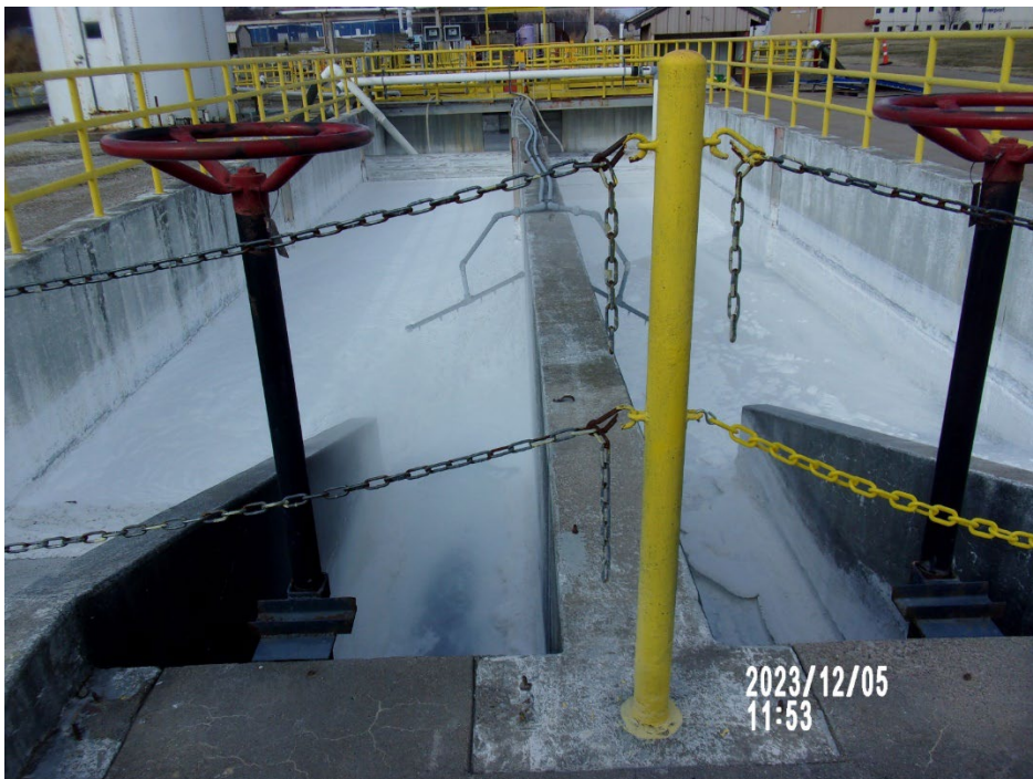
Photo 36: Wastewater Treatment tanks.
