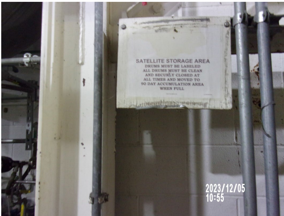
Photo 23: Satellite Accumulation Area Sign Utilized by the Facility.
