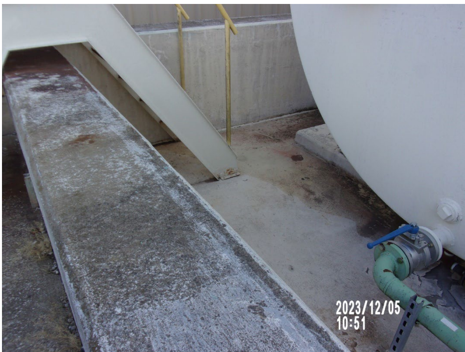
Photo 22: Secondary Containment for the Former 90-Day Hazardous Waste Accumulation Tank. The concrete in this area had been coated.
