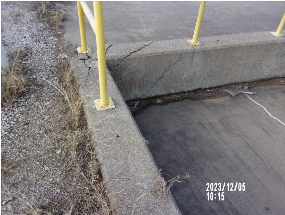
Photo 7: Cracks in the concrete containment wall in the area adjacent to the hazardous waste accumulation tank.
