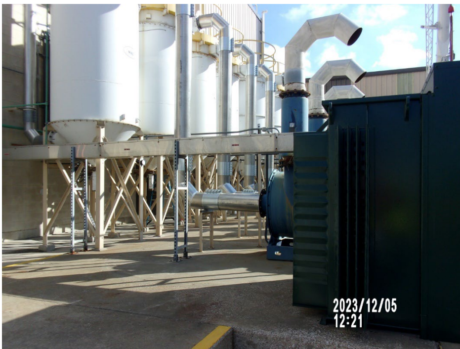
Photo 39: Air Pollution Control equipment for the facility.
