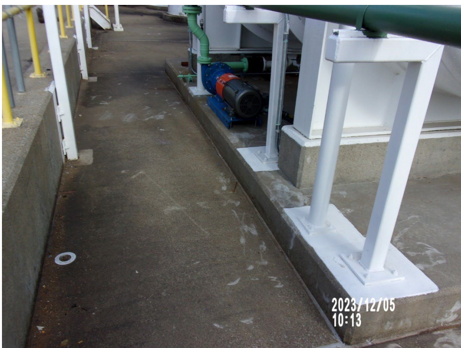
Photo 4: Secondary containment under the hazardous waste accumulation tank. The concrete is not coated.
