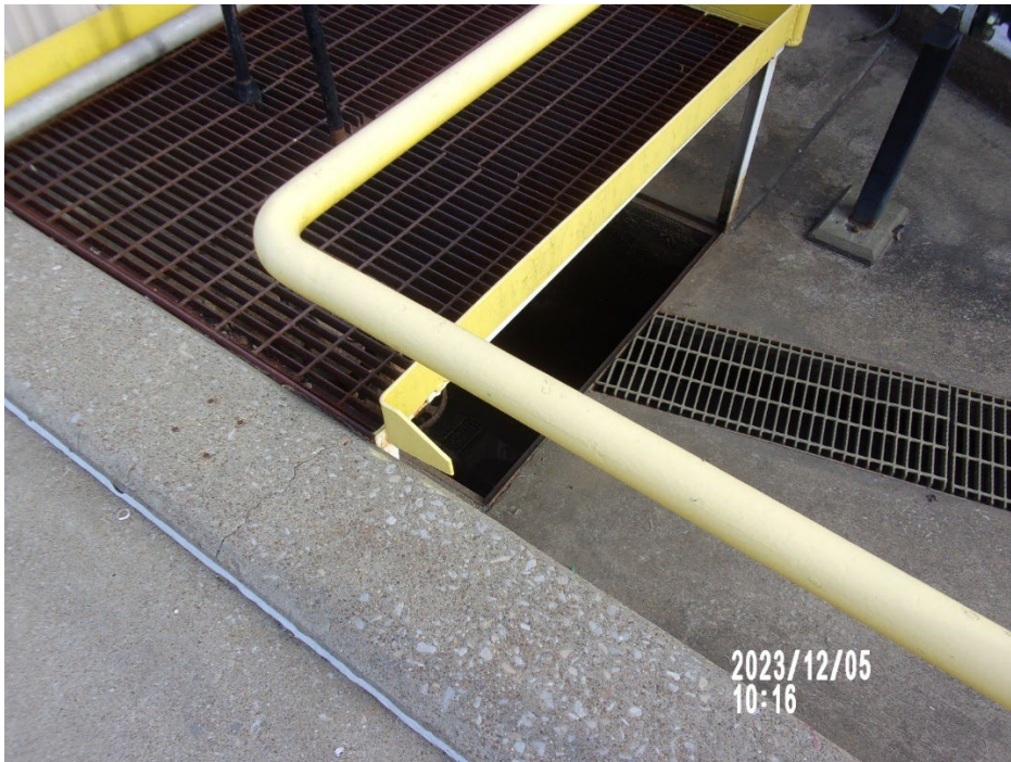
Photo 8: Small hairline crack in the containment wall near the hazardous waste accumulation tank. The concrete is not coated.
