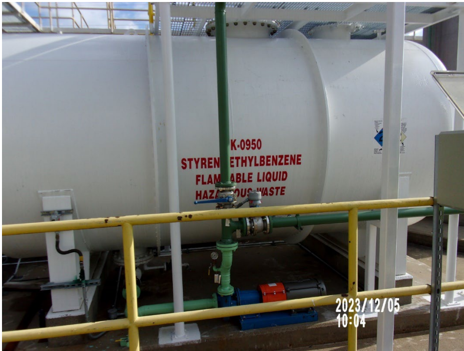
Photo 1: Hazardous Waste Accumulation Tank.
