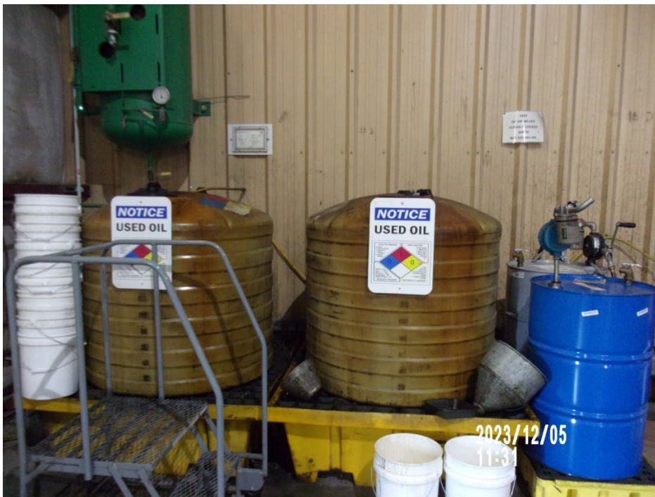
Photo 32: Used Oil Tanks in the Facility Maintenance Area.
