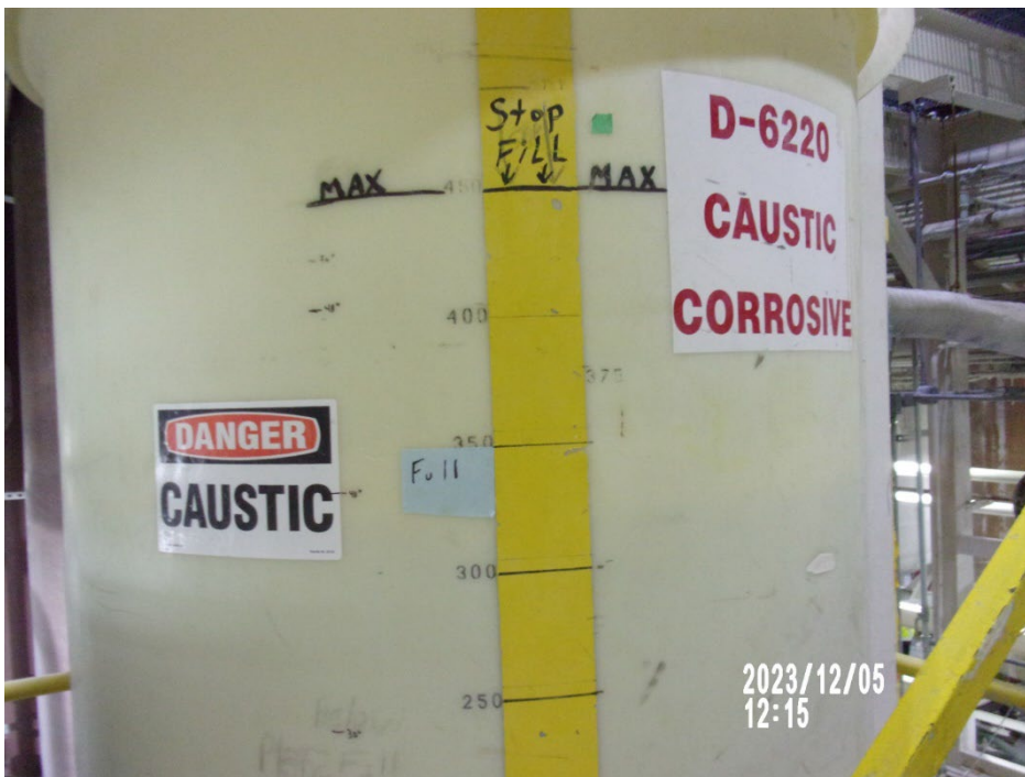
Photo 38: Caustic Storage tank for pH Neutralization.
