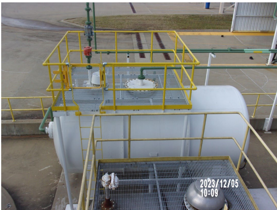
Photo 3: Top of the hazardous waste accumulation tank.
