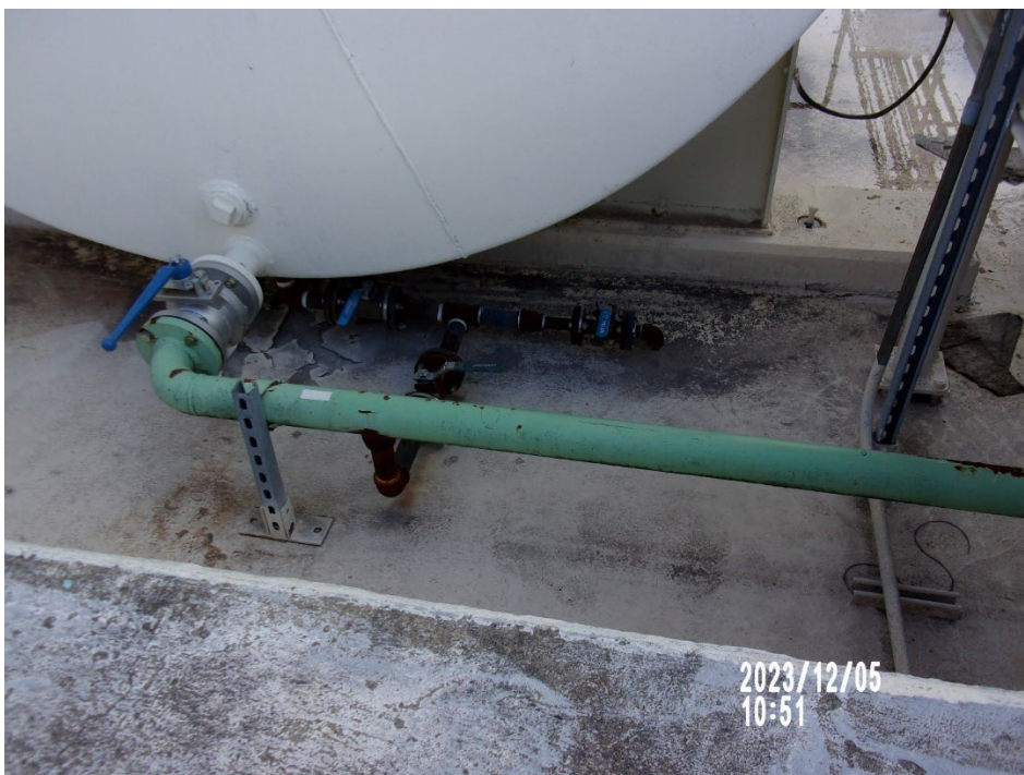
Photo 21: Secondary Containment for the Former 90-Day Hazardous Waste Accumulation Tank. The concrete in this area had been coated.
