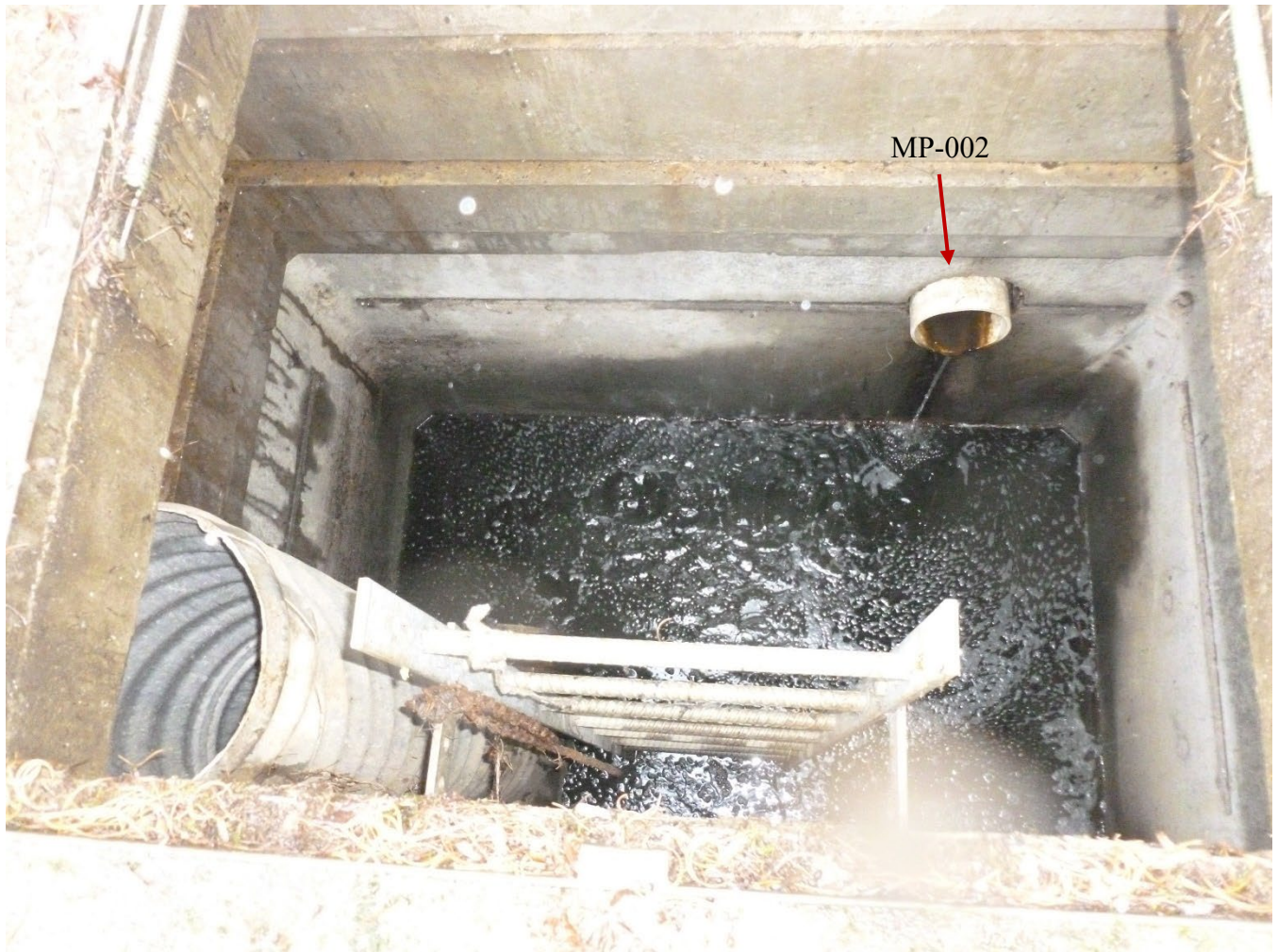
Photo 5 / P1010073 – Outfall 002 in Vault
