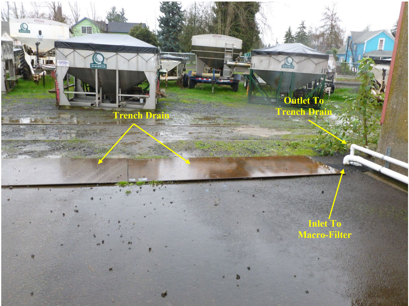
Photo 3 / P1010070 – Covered Trench Drain with Inlet and Outlet
