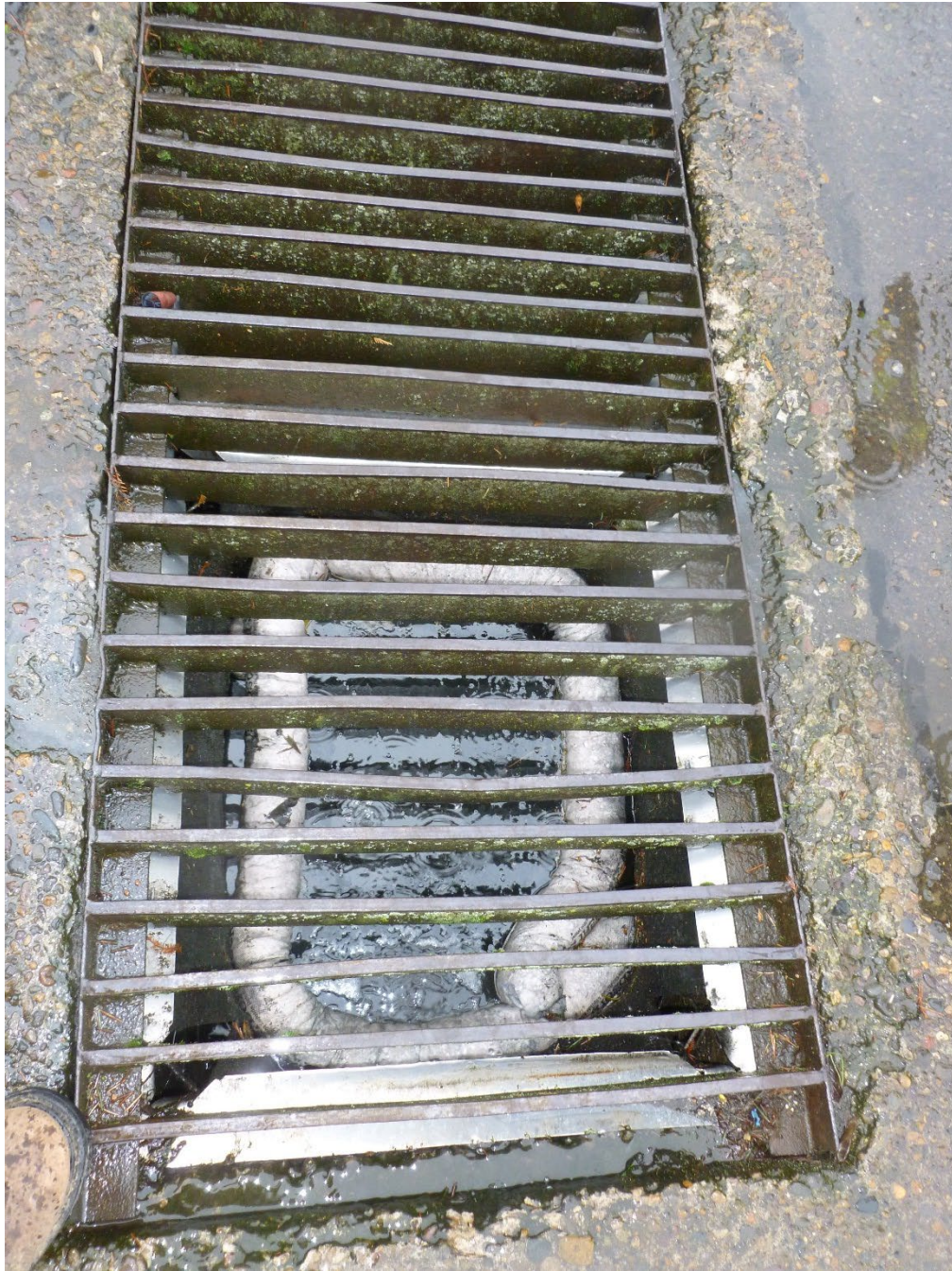
Photo 4 / P1010072 – Catch Basin, with insert
