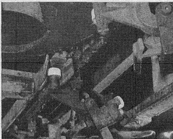
Nylon guide rollers on overhead conveyor also act as insulators and load-bearing members.
