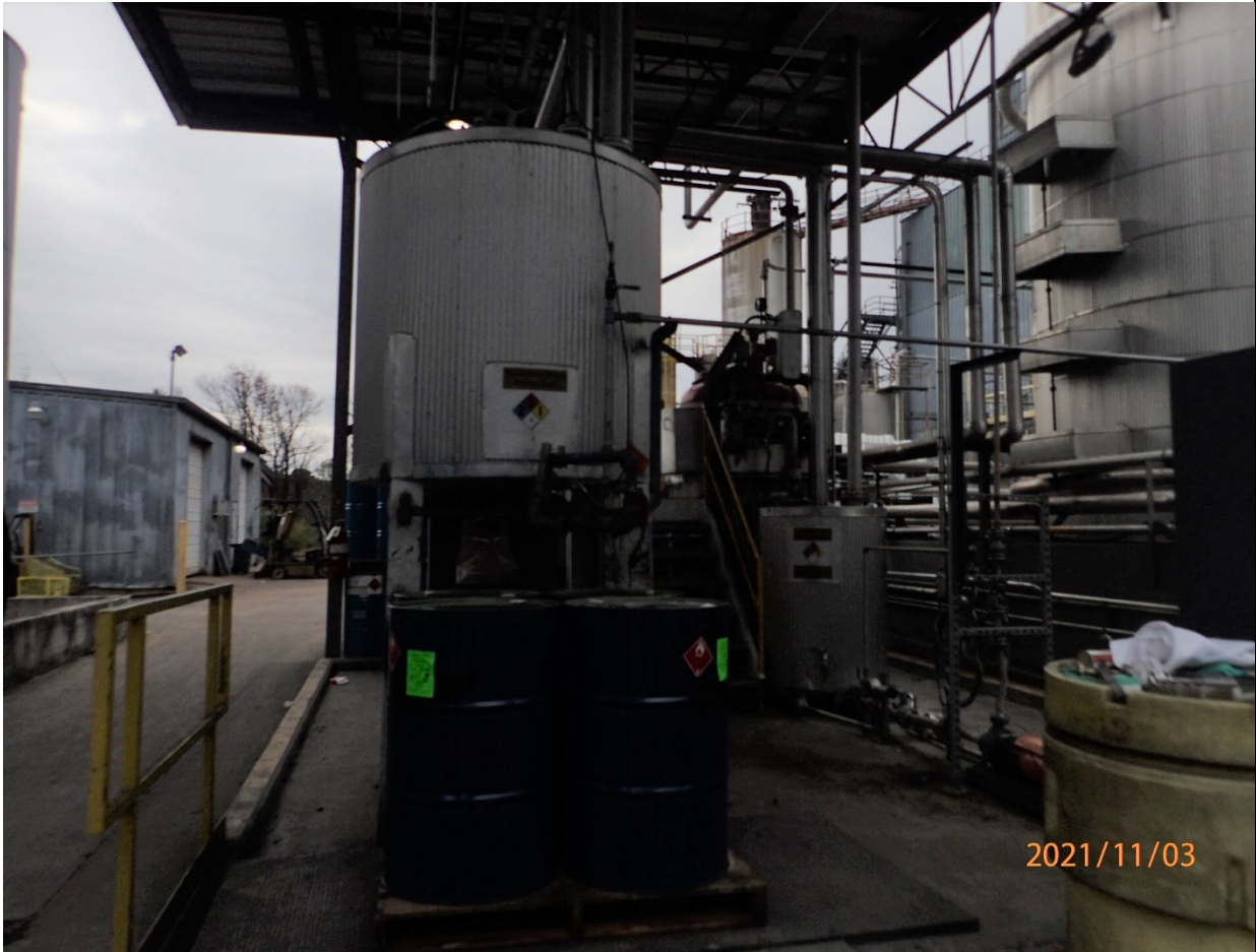
Photo 5: Solvent Reclamation Unit.
