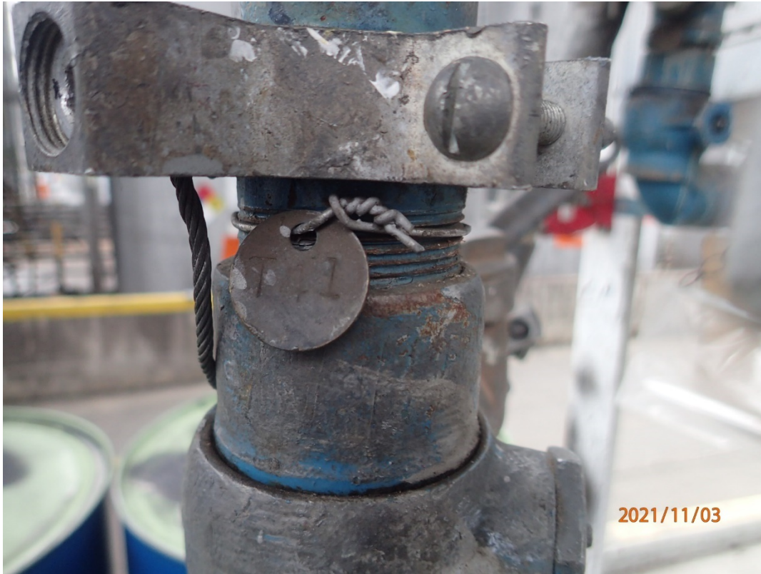
Photo 8: The ancillary equipment on the solvent reclamation unit and still bottoms tank were marked/ tagged as required by Subpart BB. The tags however were illegible due to dirt/ dust.
