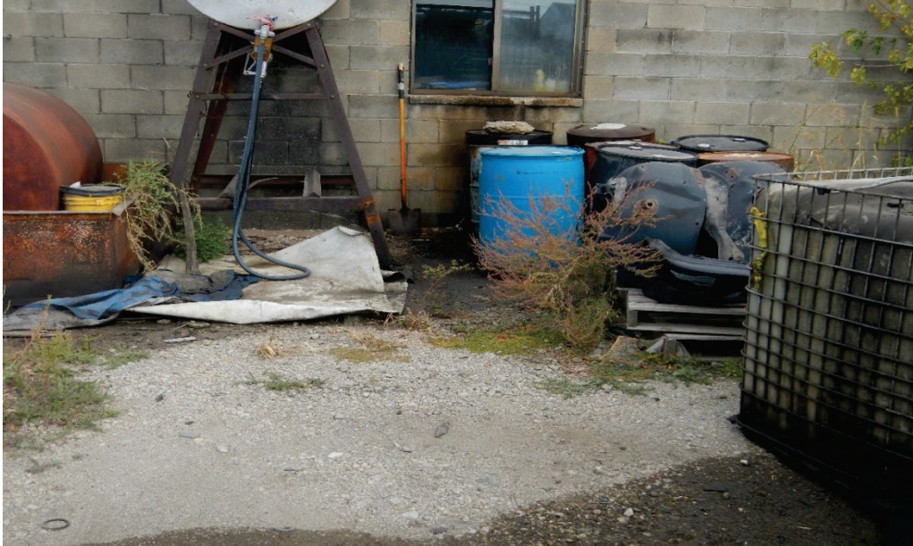
Photo 9, significant ground discoloration outside of the vehicle process building
