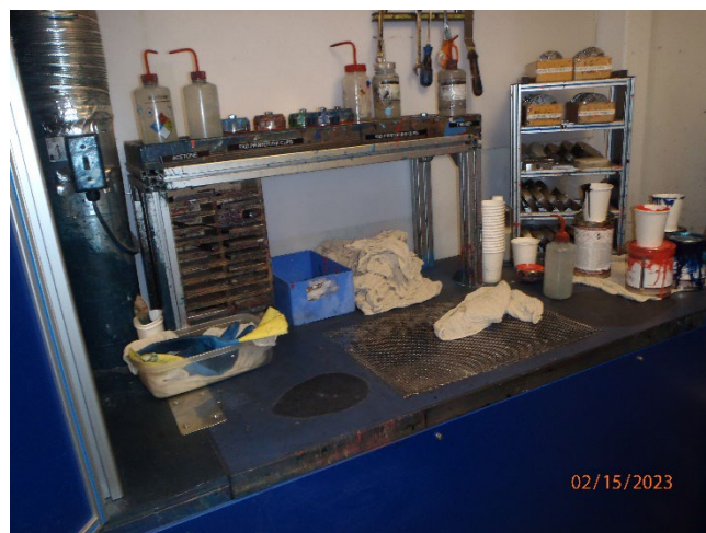
Figure 19: P2150033.JPG – Hood in the Printing Room
