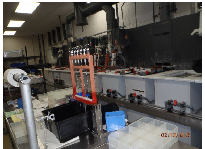
Figure 11: P2150023.JPG – New Electropolishing Line
