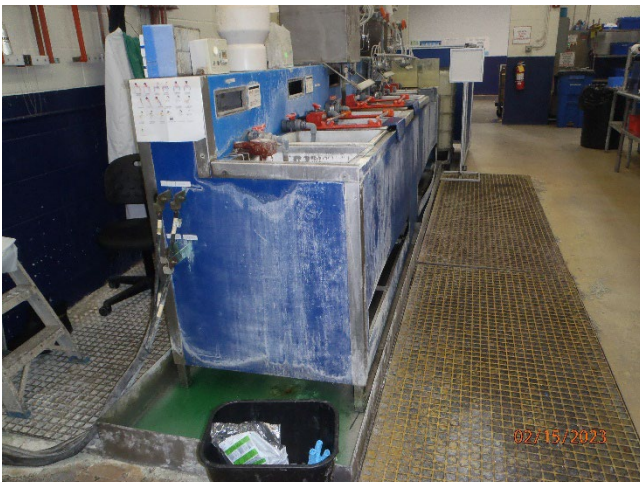
Figure 10: P2150022.JPG – Old Electropolishing Line
