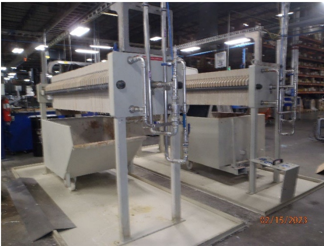
Figure 7: P2150017.JPG- ECM Filter Presses and hoppers
