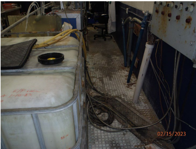
Figure 14: P2150027.JPG – Floor in the rear of the Old Electropolishing Line and Tote
