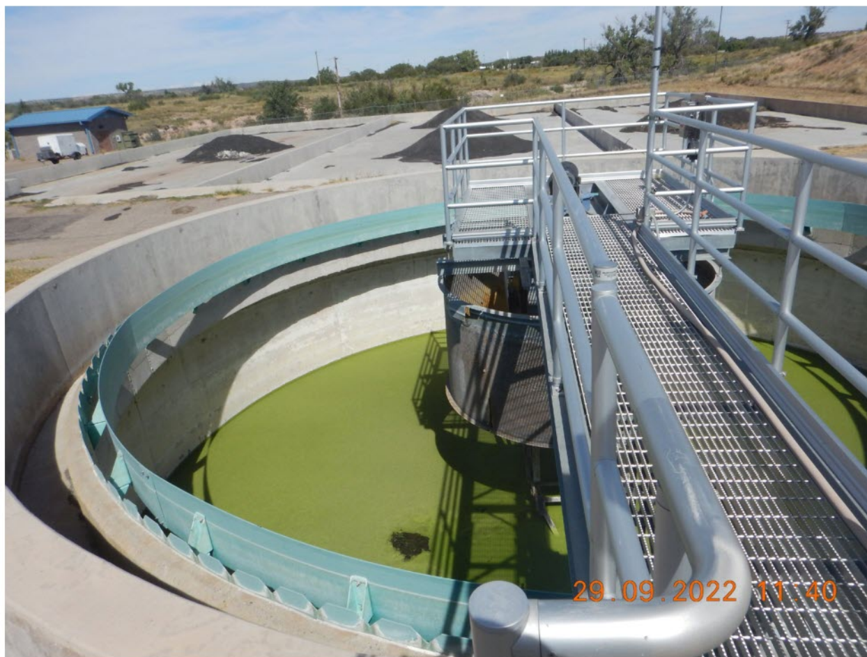
View of the Northside clarifier currently offline. (DSCN2359) photographed by D. Esparza.
