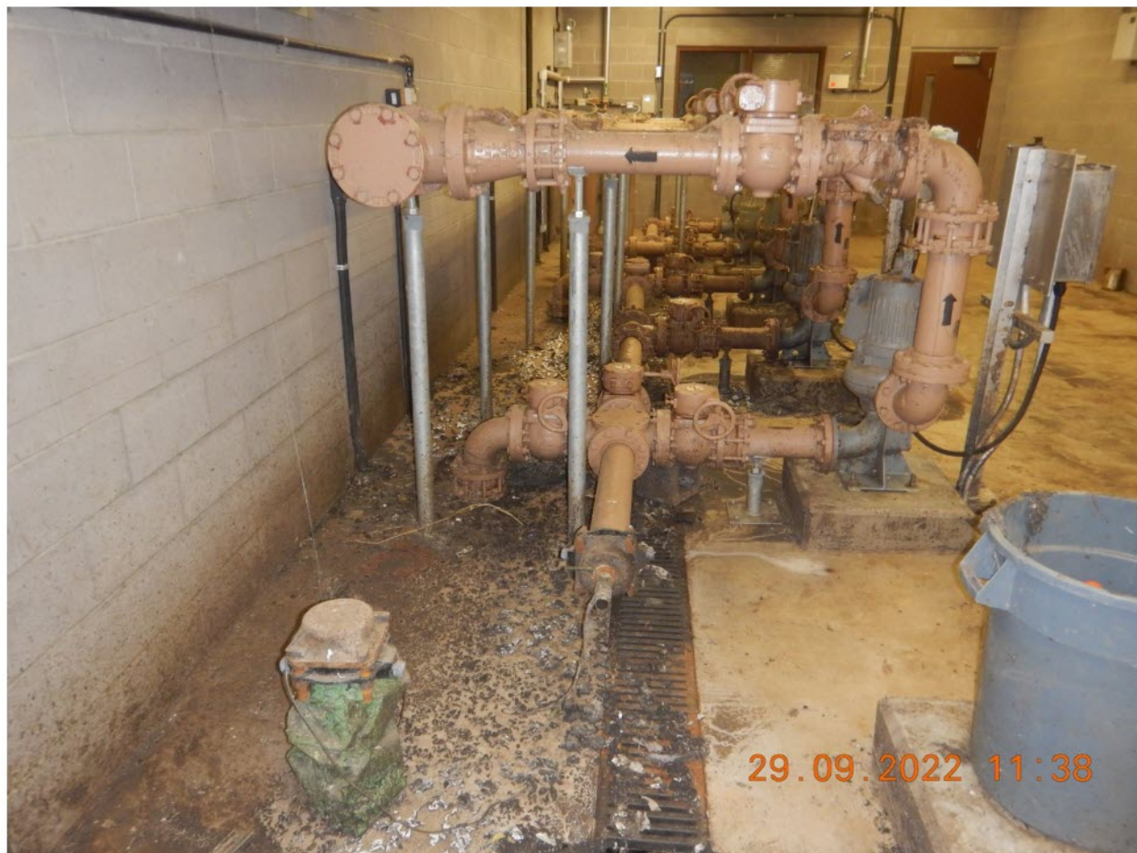
Another view of the visible overflow debris inside the pump room looking approximately Southeast. (DSCN2357). Photographed by D. Esparza.
