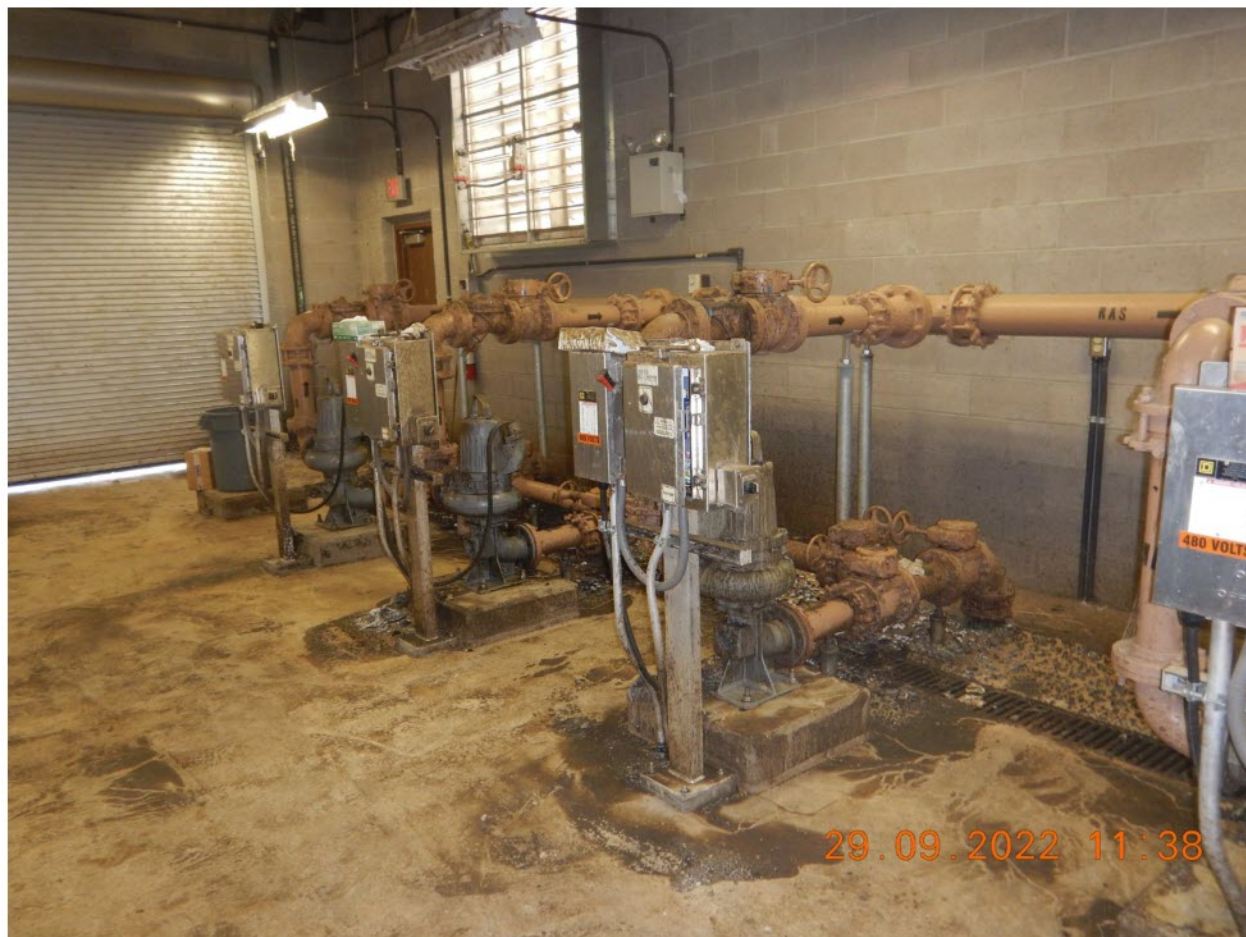
View of the visible overflow debris inside the pump room looking approximately Northeast. (DSCN2356) Photographed by D. Esparza.
