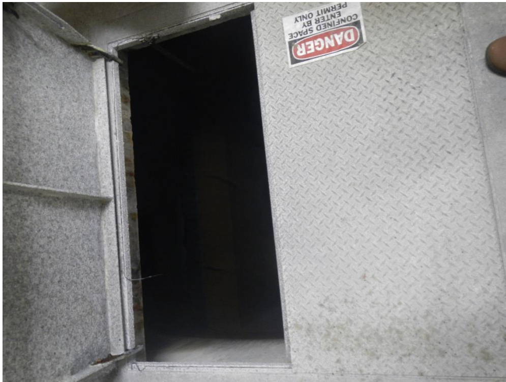
Photograph 2: Post-mix basin hatch, which lacks sanitary seal.
