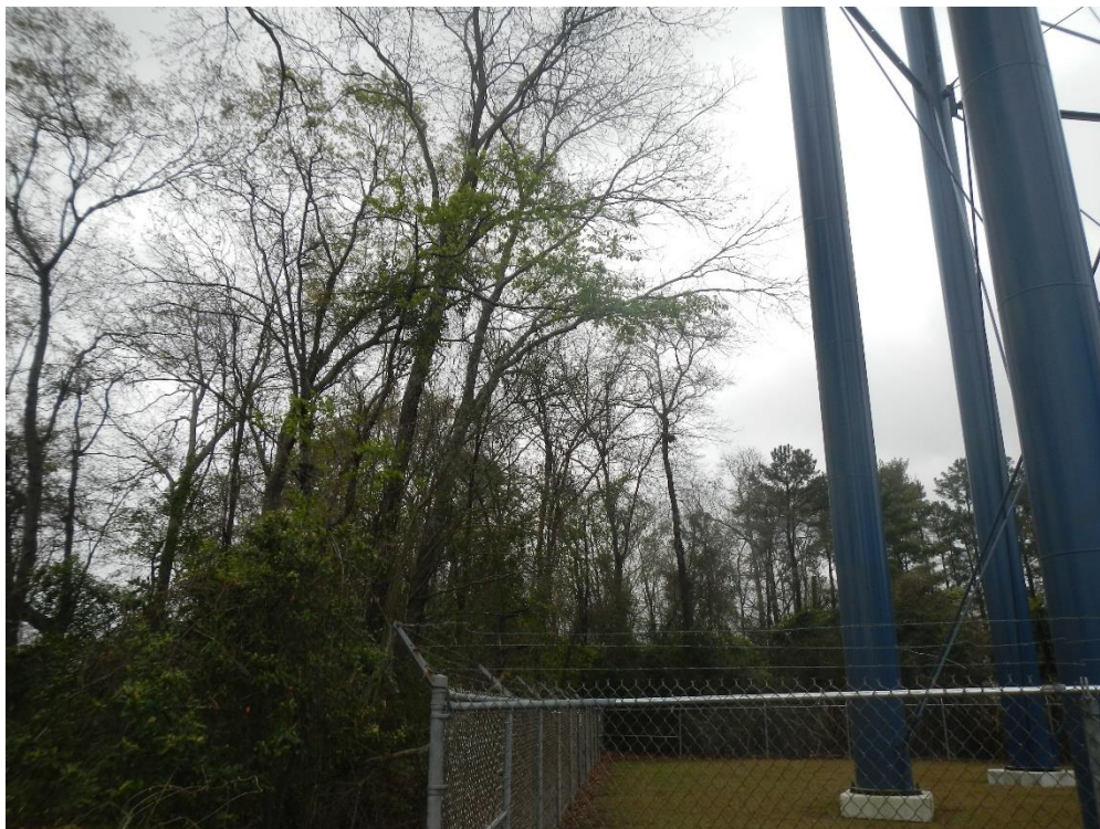
Photograph 3: Base of Platt Springs elevated storage tank with vegetation in the vertical plane.
