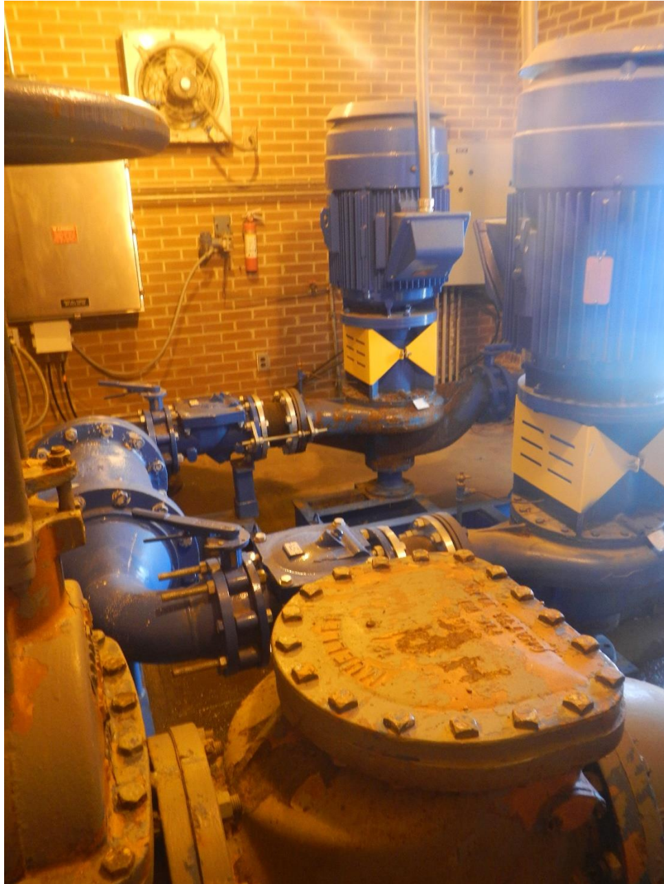
Photograph 6: Altitude valve at Green Hill high service pump station exhibiting corrosion.
