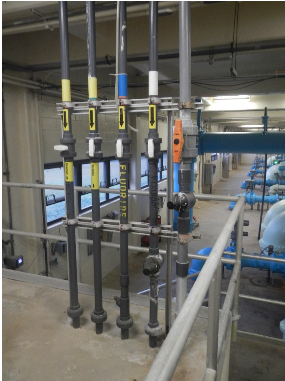
Photograph 1: Misabeled chemical injection pipes at Lake Murray plant.
