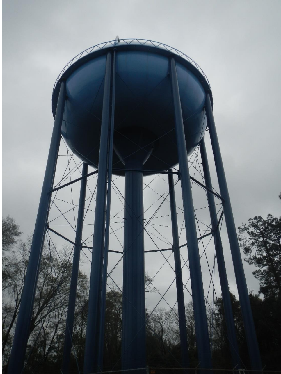
Photograph 4: Platt Springs elevated storage tank with vegetation in the vertical plane.
