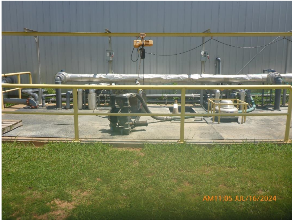
Photograph 1: Three 66,000-gallon wastewater collection pits (underground).
