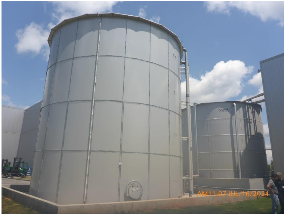
Photograph 2: Wastewater equalization tanks.
